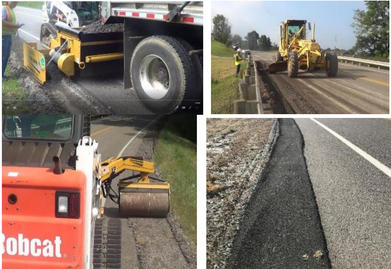
Figure A.4 Pictures taken during construction of berm test section in Monroe County
