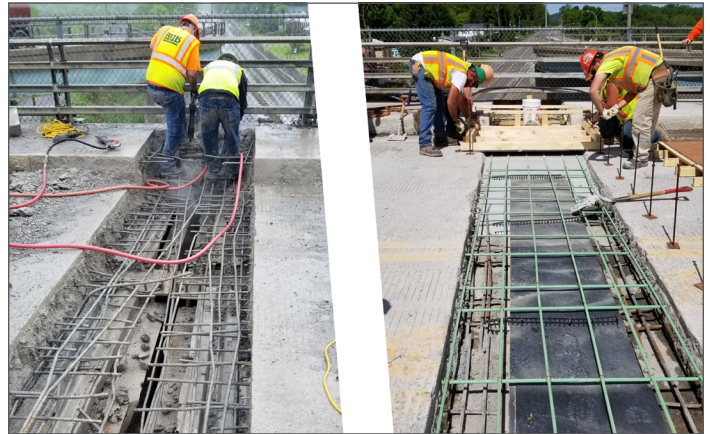
Replacement of an expansion joint with a UHPC link slab. Source: New York State Department of Transportation
