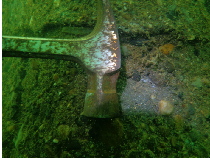
Figure 50. Photo. Typical cold joint after cleaning.
