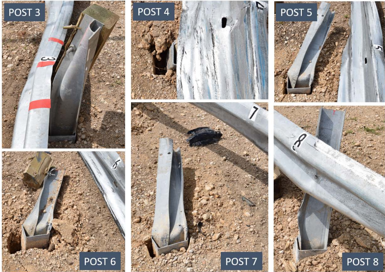
Figure 7.4. Movement of Some of the Sleeves after Test No. 611011-1.
