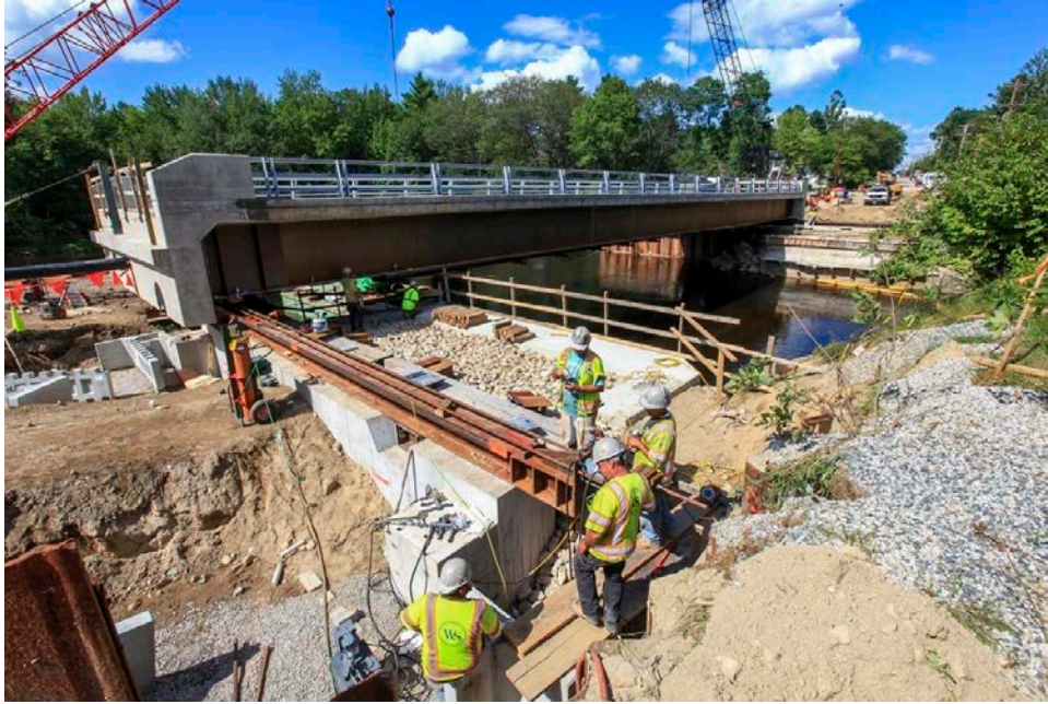
Figure 22. Photo. Sliding of superstructure.
