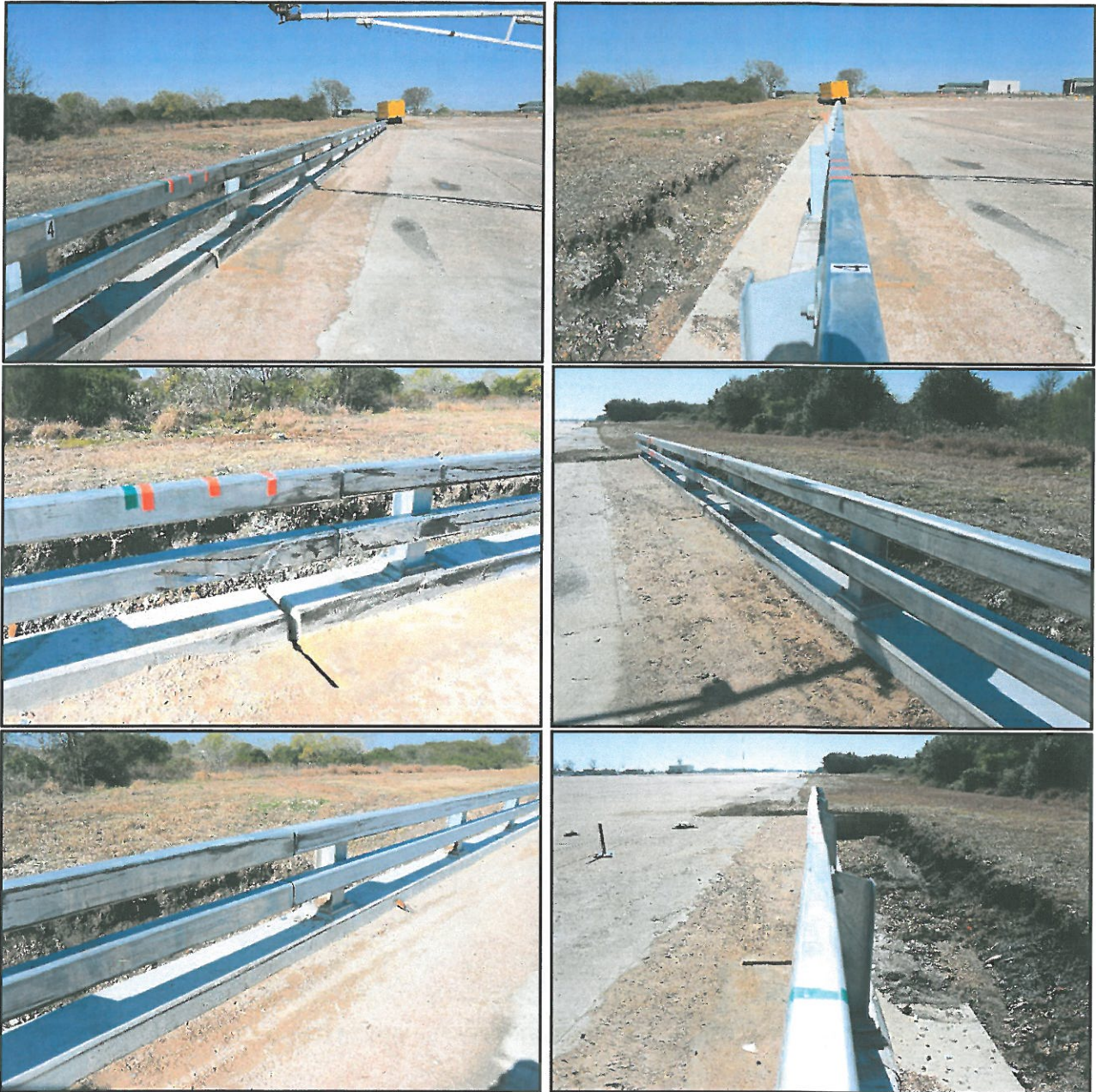
Figure 5.3. Overall Damage to Alaska Bridge Rail after Test No. 608331-01-1A.
