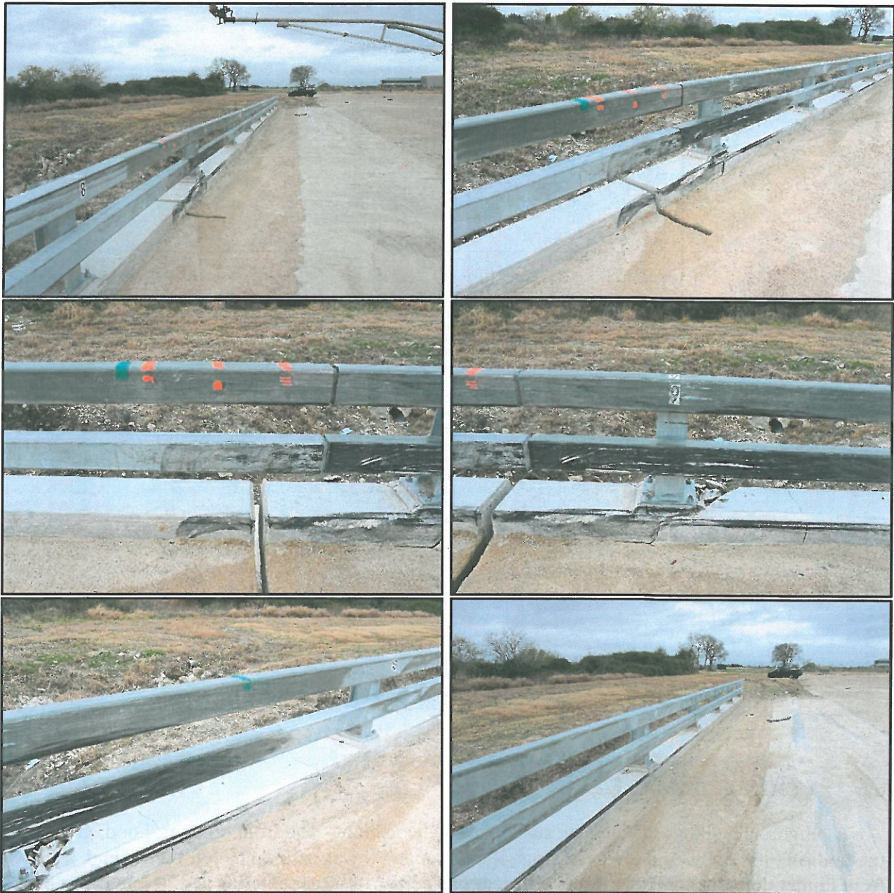
Figure 6.3. 2019 MASH 2-Tube Bridge Rail after Test No. 608331-01-2.
