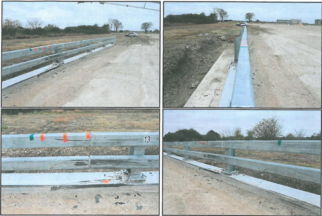
Figure 7.3. 2019 MASH 2-Tube Bridge Rail after Test No. 608331-01-3.
