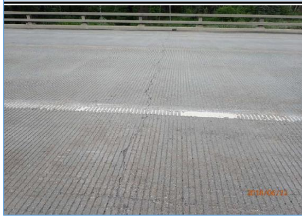
Figure 2.3 Cracks on silica fume deck at Troublesome Creek Bridge (Alaska DOT&PF Bridge Section, 2018)
