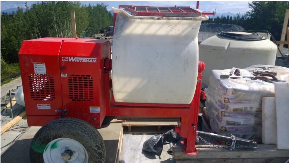
Figure G-14. Whiteman 7 cubic foot mixer used on site for grout mixing
