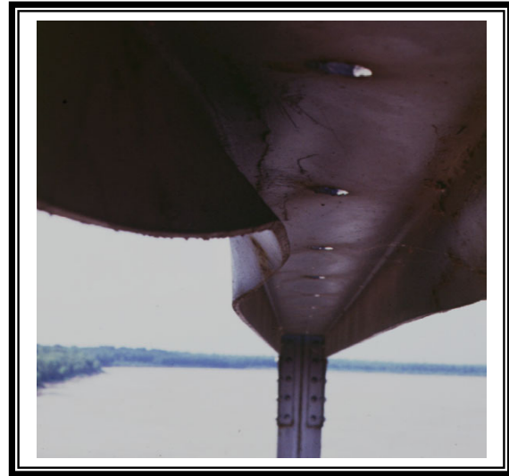
Figure 49. Typical Category L/U damage.
