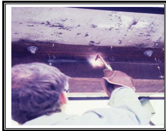
Figure 8. Line heat in progress on the web of a wide flange beam.
