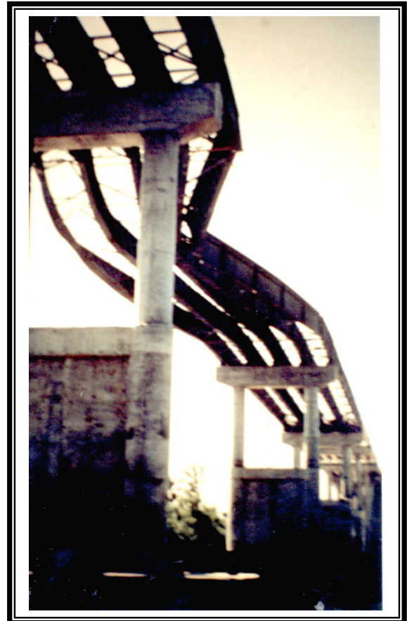
(b) Category W damage to main girders during construction of a Louisiana bridge.
