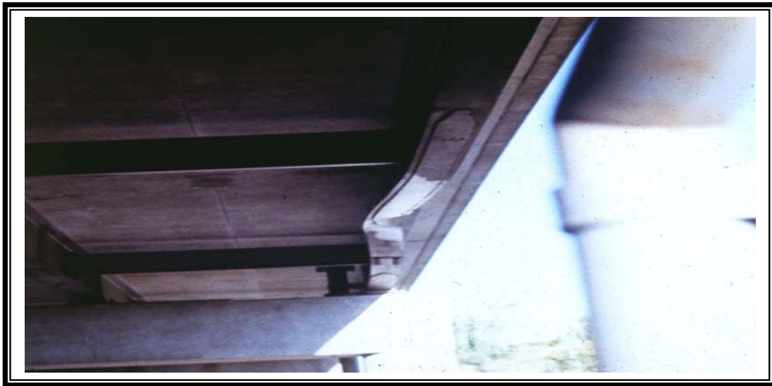
(b) Category T damage on a composite bridge girder impacted by an over-height vehicle in Wisconsin.
