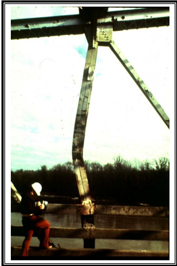
(a) Category W damage on a built-up double channel truss member. The damage was caused by a log falling from a truck on a bridge in North Louisiana.
