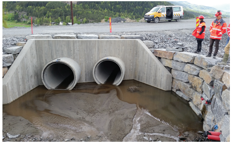
Figure 5: New culvert in Norway designed to prevent road destruction. Photo credit: FHWA
