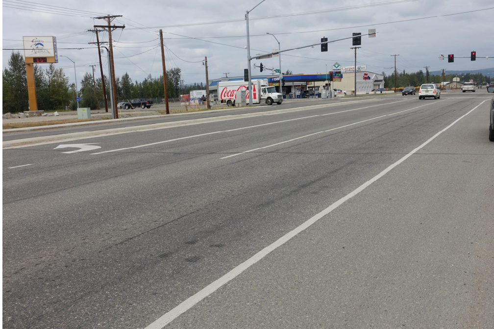
Figure 4.54 Peger Rd Resurfacing / FMATS Ped Impr / NR Signal Interconnect, PG 52-40, constructed in 2017
