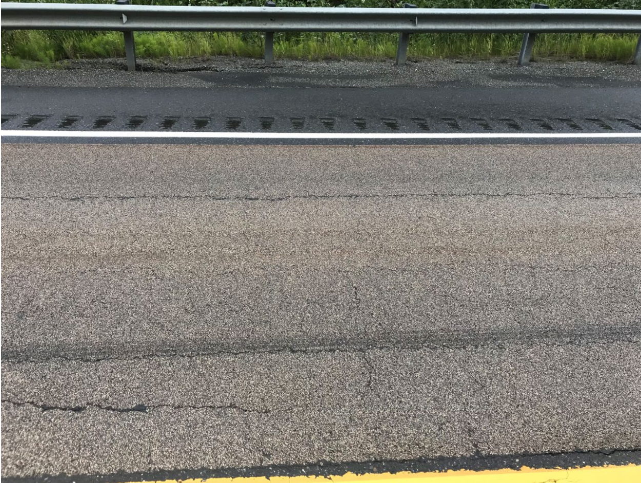
2018 Photo – observed cracking pattern
