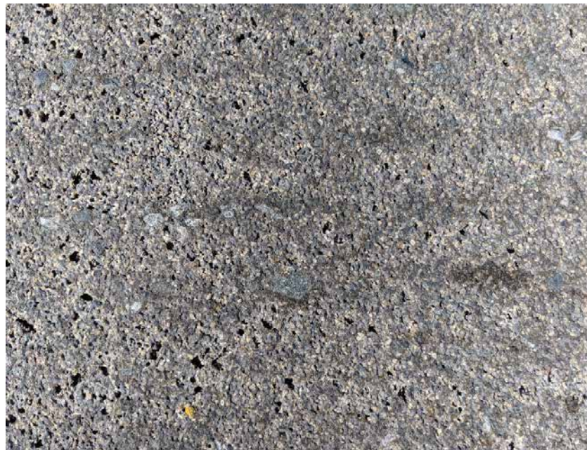
2019 – Bare Pavement and Significant Wear
