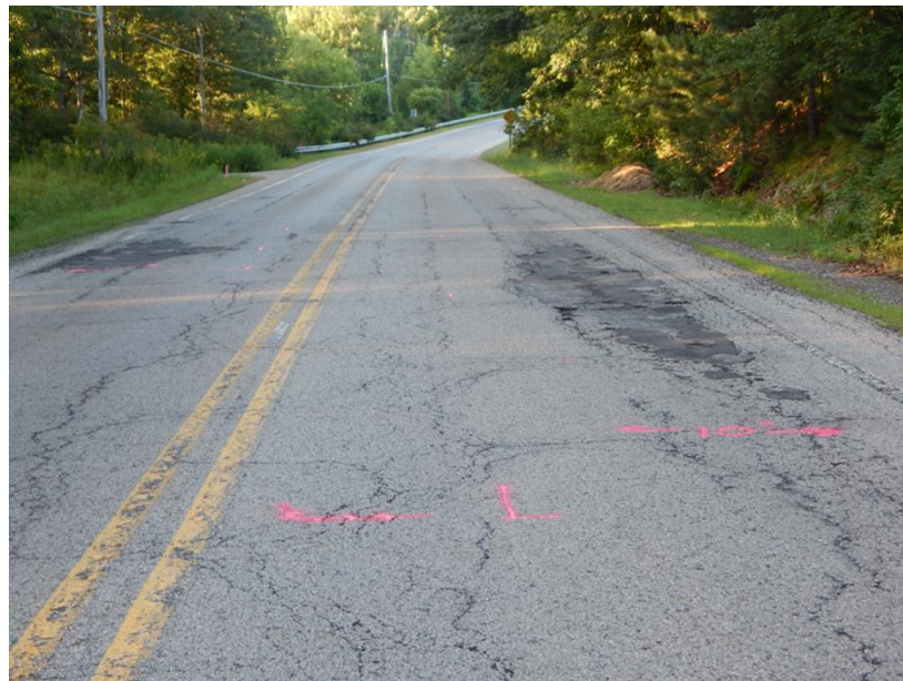
Figure 4. Failed areas of the existing pavement.
