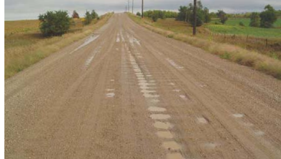
Figure 61. Photo. Too little crown (<4%).
