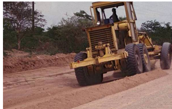
Figure 62. Photo. Too much crown (>6%).
