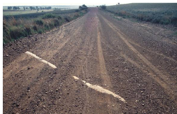
Figure 20. Photo. Insufficient, poor quality gravel.
