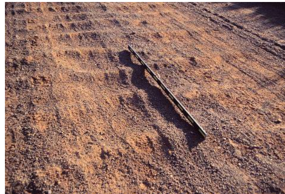
Figure 58. Photo. Poor gravel selection for treated road.
