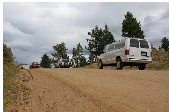
Figure 60. Photo. Good crown (4 to 6%).
