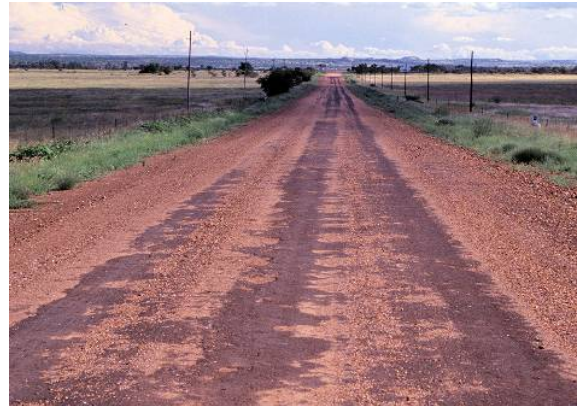
Figure 70. Photo. Insufficient additive application.
