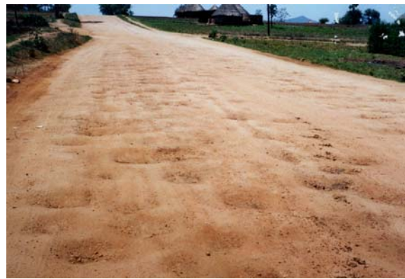
Figure 23. Photo. Potholes caused by poor drainage.
