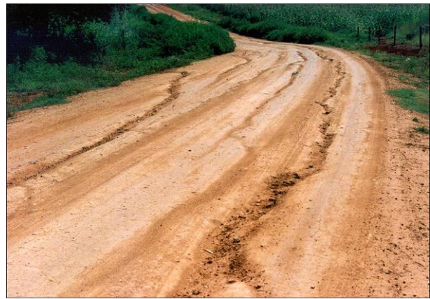
Figure 37. Photo. Longitudinal erosion.
