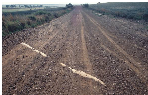
Figure 20. Photo. Insufficient, poor quality gravel.
