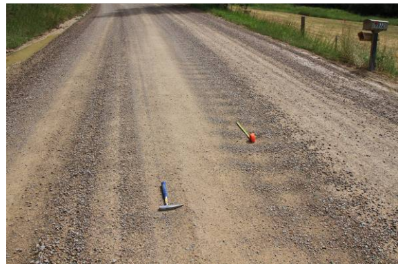
Figure 59. Photo. Chloride applied to poorly prepared road.
