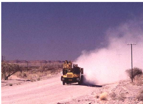
Figure 85. Photo. Unacceptable level of dust. (5 on scale of 1-5).
