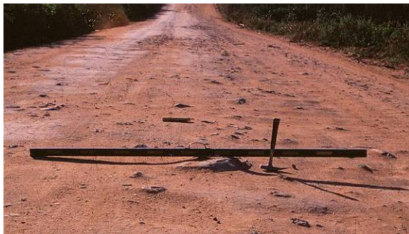
Figure 88. Photo. Estimating gravel loss from stone protrusion.
