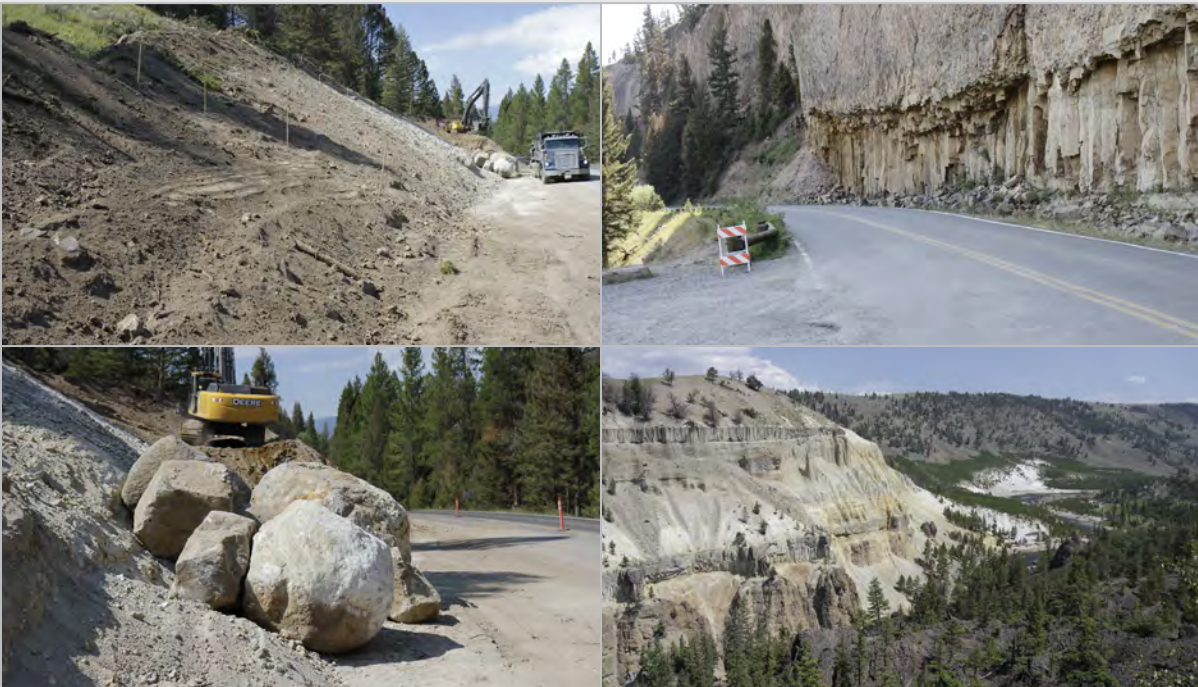
Top left: Topsoil is pushed to the top of slope for placement following construction. Top right: Vertical walls make construction challenging through this area. Bottom left: Large boulders are excavated and placed elsewhere in the project area. Bottom right: View from the corridor to the valley below
