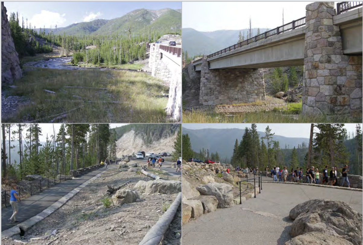
Top left: Little evidence exists of the former roadway alignment along the Gibbon River. Top right: New alignment with retaining walls of native stone and bridge over the Gibbon River. Bottom left and right: An expanded parking area and pedestrian pathways provide access to the falls viewing area.
