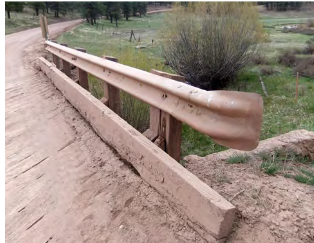
Figure 4-3: Example of a guardrail not meeting safety requirements (Source: Parsons Brinckerhoff, Cuba La Cueva, New Mexico)
