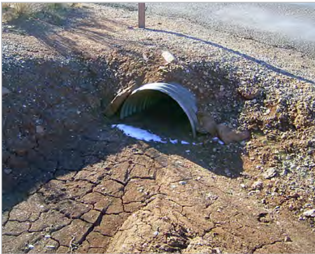
Figure 4-2: Example of a culvert clogged by sediment (Source: Parsons Brinckerhoff, Capitol Reef Route 10, Utah)
