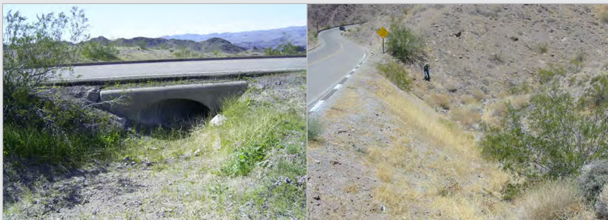
Left: culvert entrances located within clear zone, creating a hazard for motorists. Right: steep side slopes without guardrails.
