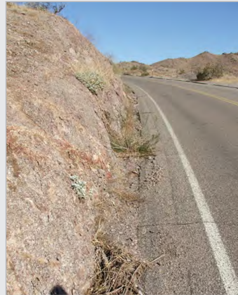
Steep roadside embankments without shoulder
