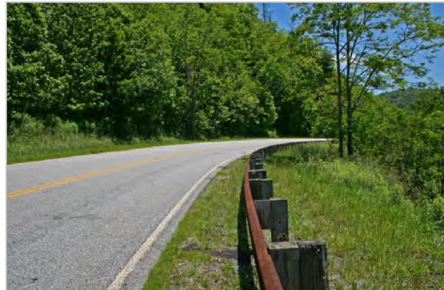
Figure 4-1: Example of overgrown vegetation
