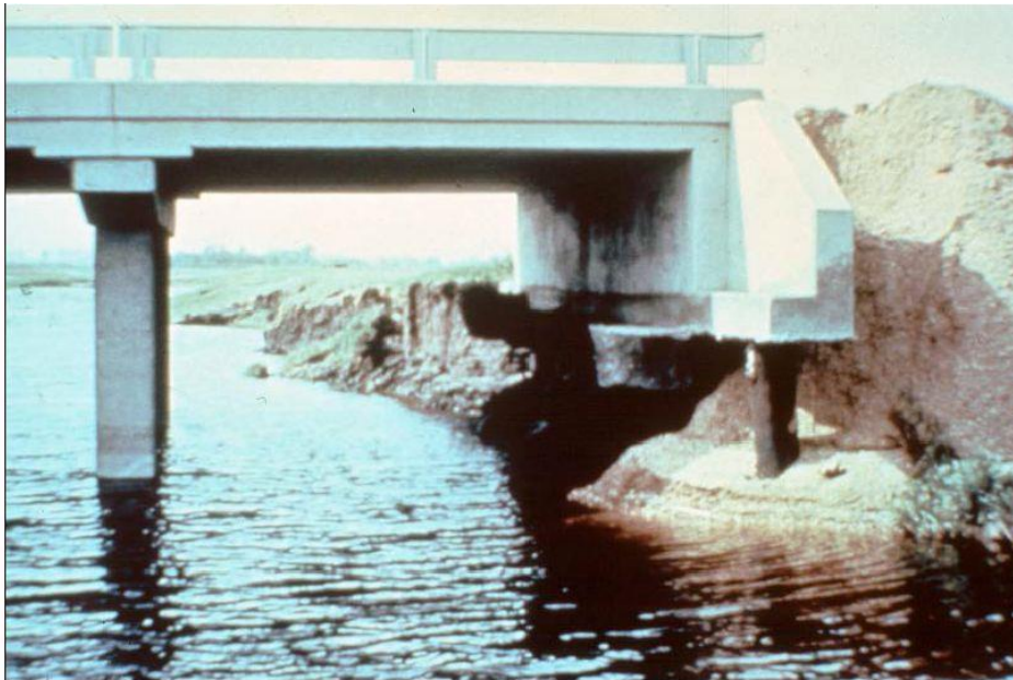
Figure 45: Example of Severe Scour at a Bridge Abutment 166
