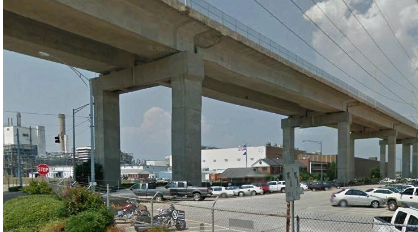
Figure 33: Image of Typical Bent Configuration for Bents 1 to 15 and Bents 18 to 32 on the Cochrane-Africatown USA Bridge 105
