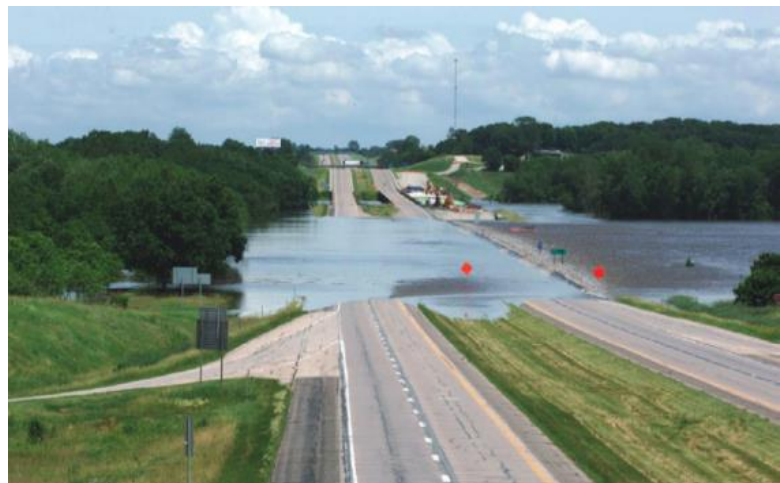
FIGURE 19: FLOODING OF I-80 NEAR CEDAR RAPIDS, IOWA. Source: IDOT Pilot study.
