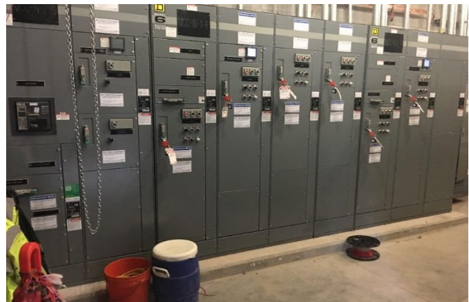
FIGURE 31: TYPICAL ELECTRICAL PANELS VULNERABLE TO WATER DAMAGE.
