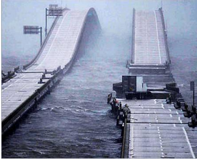
FIGURE 11: SOME OF THE 2004 DAMAGE TO THIS INTERSTATE BRIDGE CAN BE ATTRIBUTED TO THE SEA LEVEL RISE THAT OCCURRED IN THE PREVIOUS DECADES (I-10; PENSACOLA, FLORIDA).
