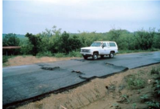
FIGURE 24: PAVEMENT DAMAGE FROM EXPANSIVE
