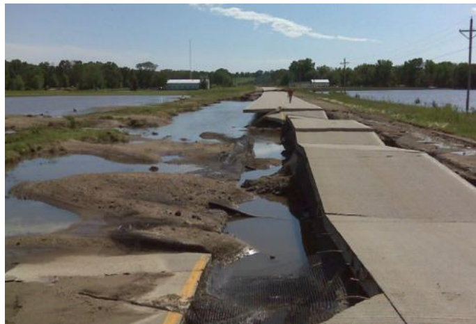
FIGURE 16: IA-1 FLOOD DAMAGE NEAR MOUNT VERNON, IOWA.
