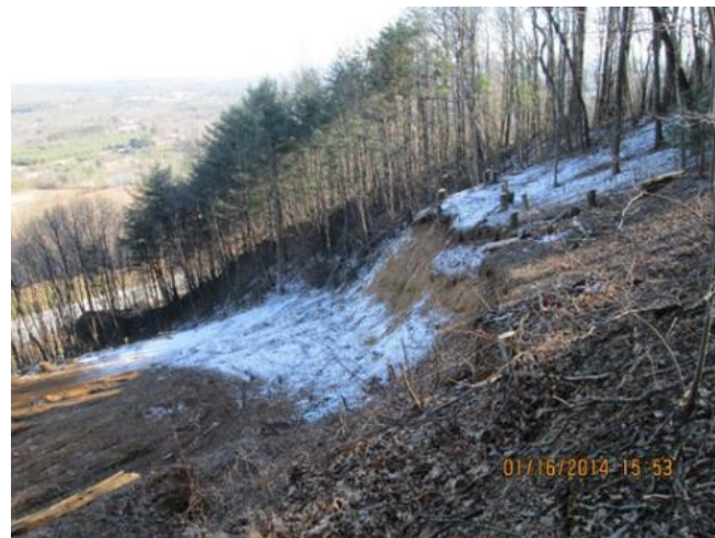
FIGURE 25: UPPER ESCARPMENT ALONG VIRGINIA I-77 FROM THE TEACR SLOPE STABILITY STUDY.
