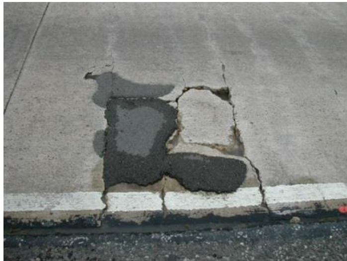
FIGURE 23: TYPICAL CRCP PUNCHOUT.
