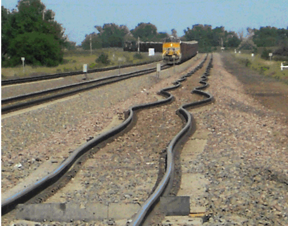
Figure 4: Aftermath of a Rail Buckling Event
