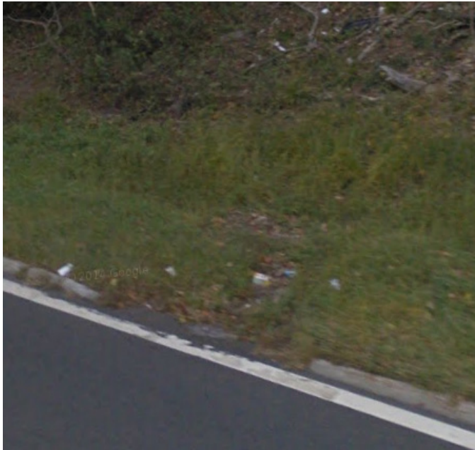
Figure 7: Overgrown grass and debris at a curb opening on Saw Mill River Parkway
