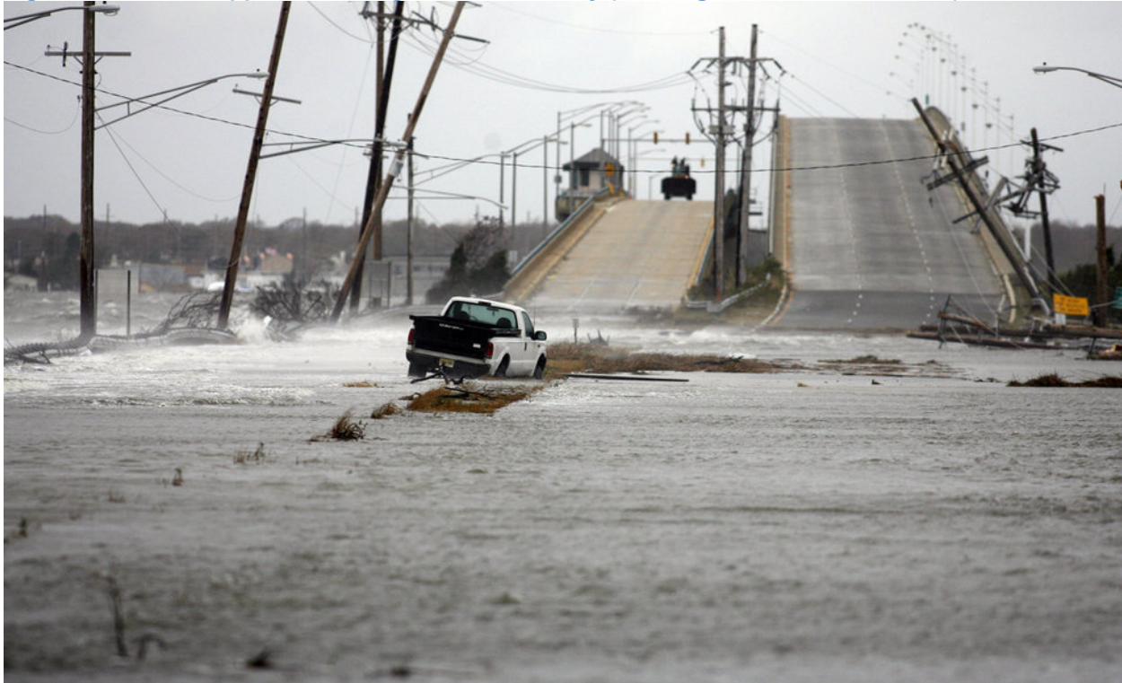
Figure 3: Eastern Approach during Hurricane Sandy (Looking West from Peninsula)
