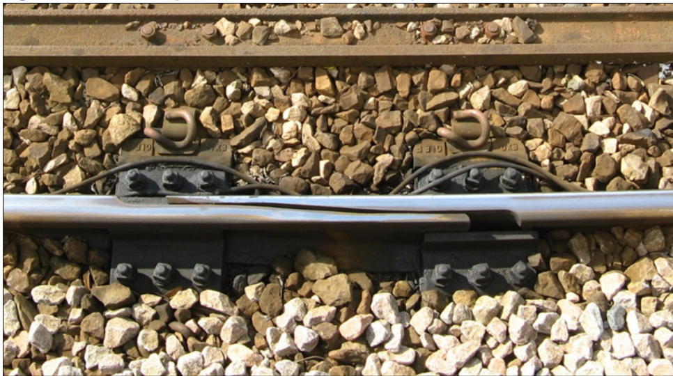
Figure 3: A CWR Expansion Joint With Rail Gap
