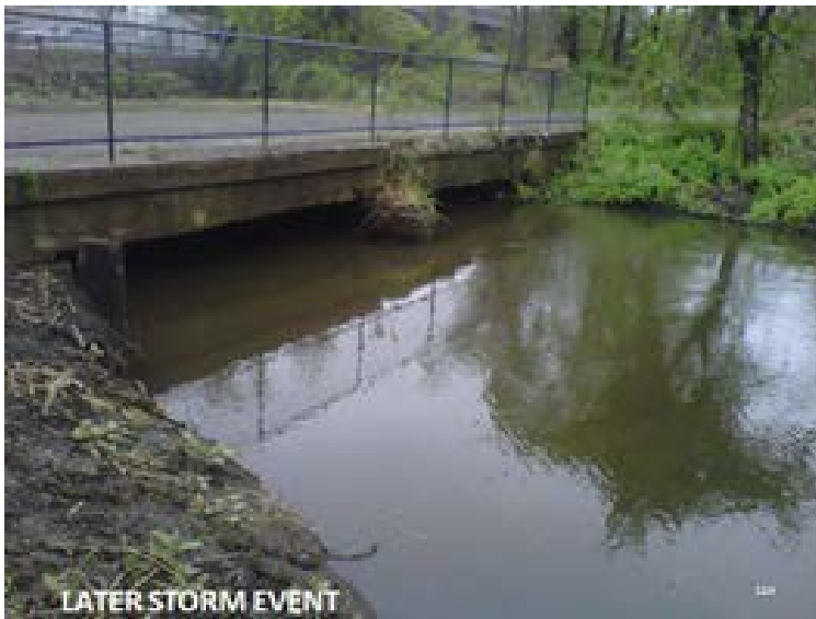
Figure 5: Culverts after later storm event
