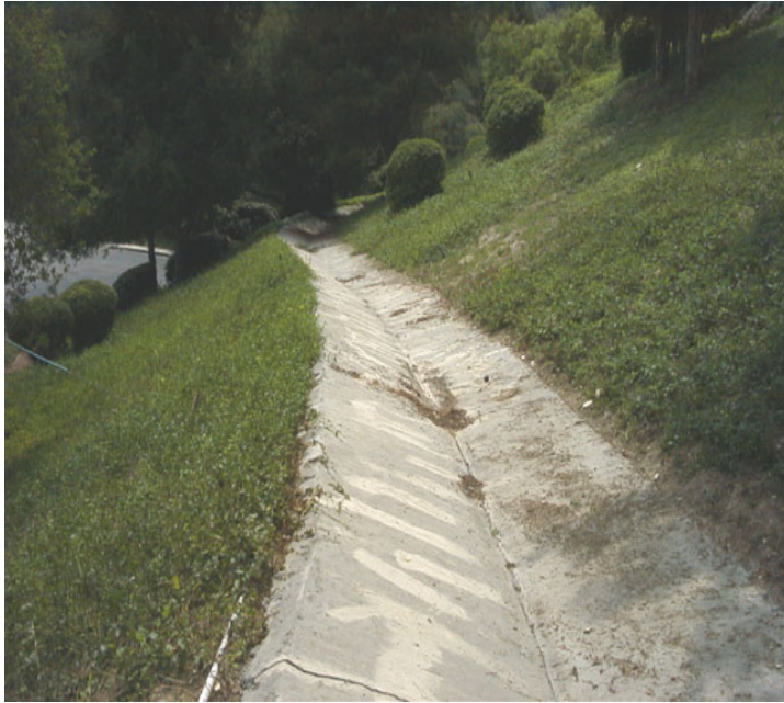
Figure 8: An example paved ditch to convey stormwater to an outfall location
