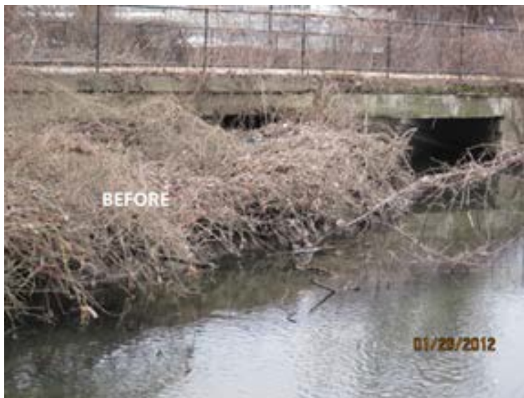
Figure 3: Debris blocking/clogging one of two box culverts on the South County Trailway, adjacent to the Saw Mill River Parkway south of Lawrence Street
