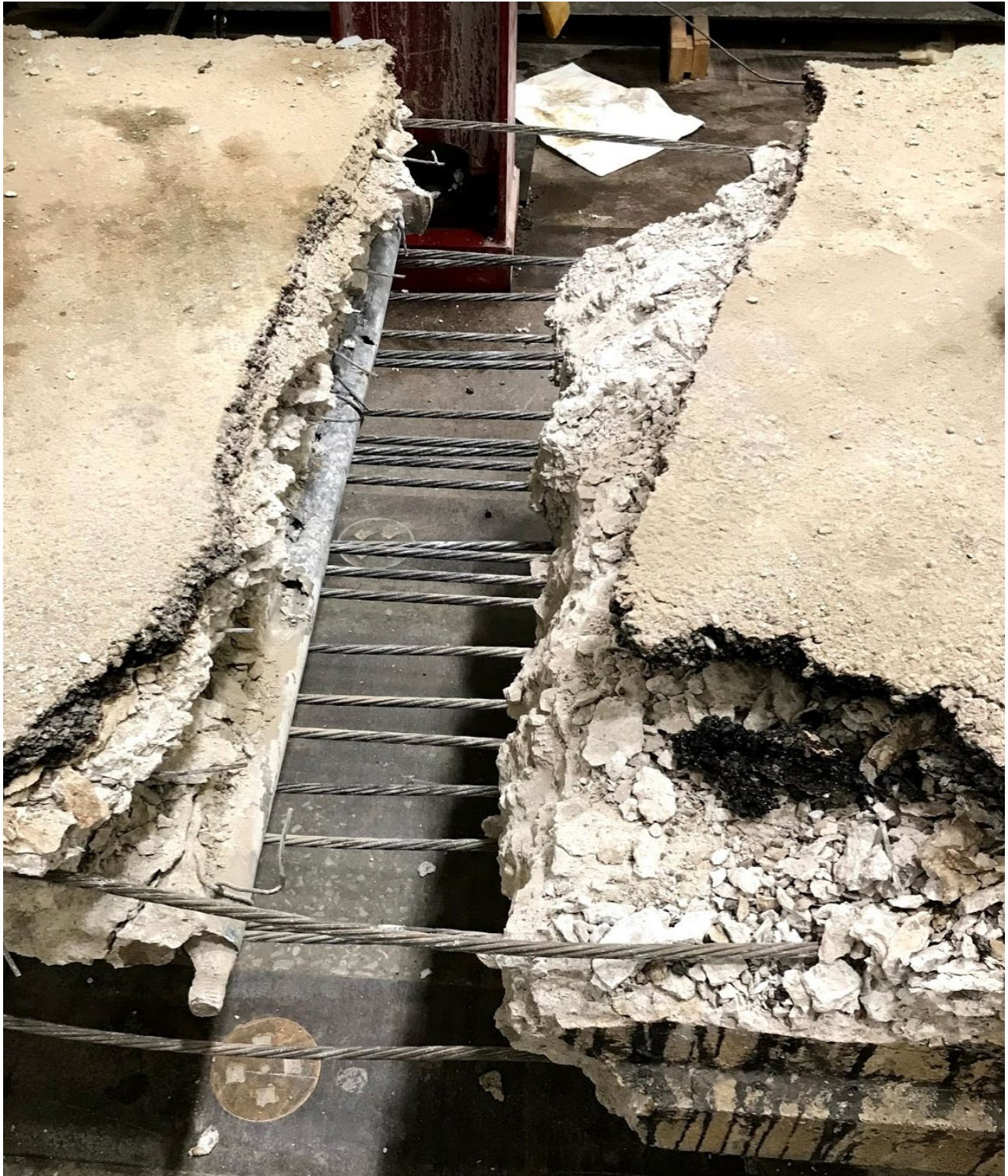
Figure 14. Photo. Exposed prestressing strands near midspan of the test specimen.
