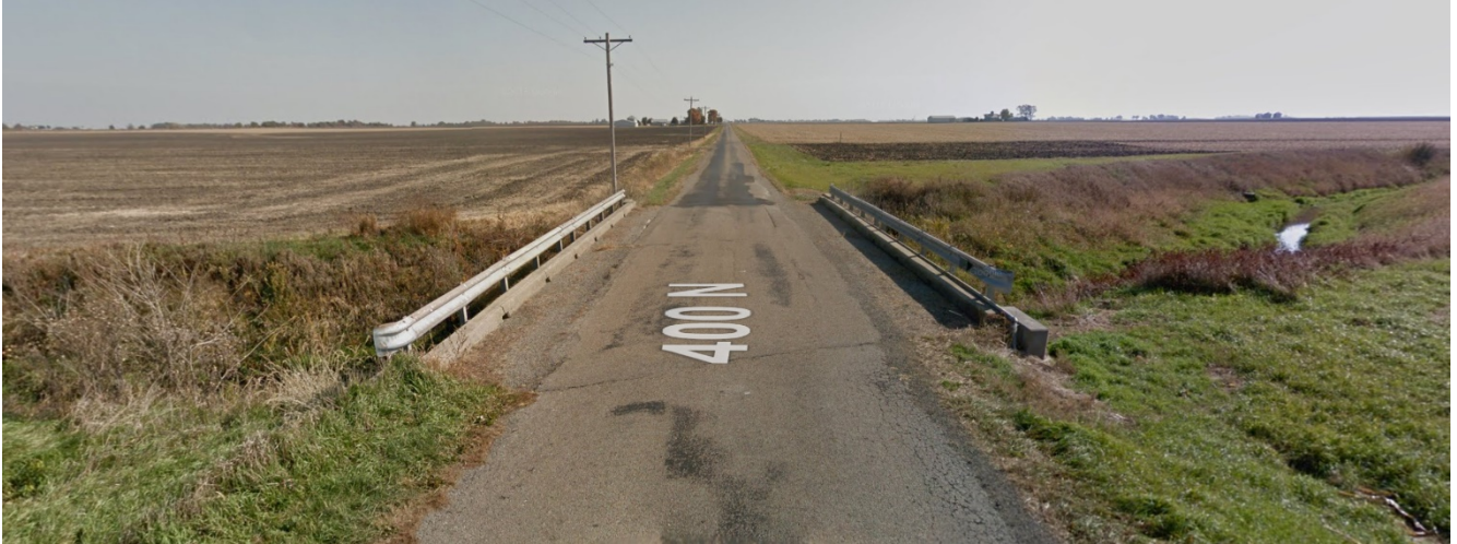
Figure 2. Photo. A picture of structure number 020-3087 taken in October 2015 via Google Maps.
