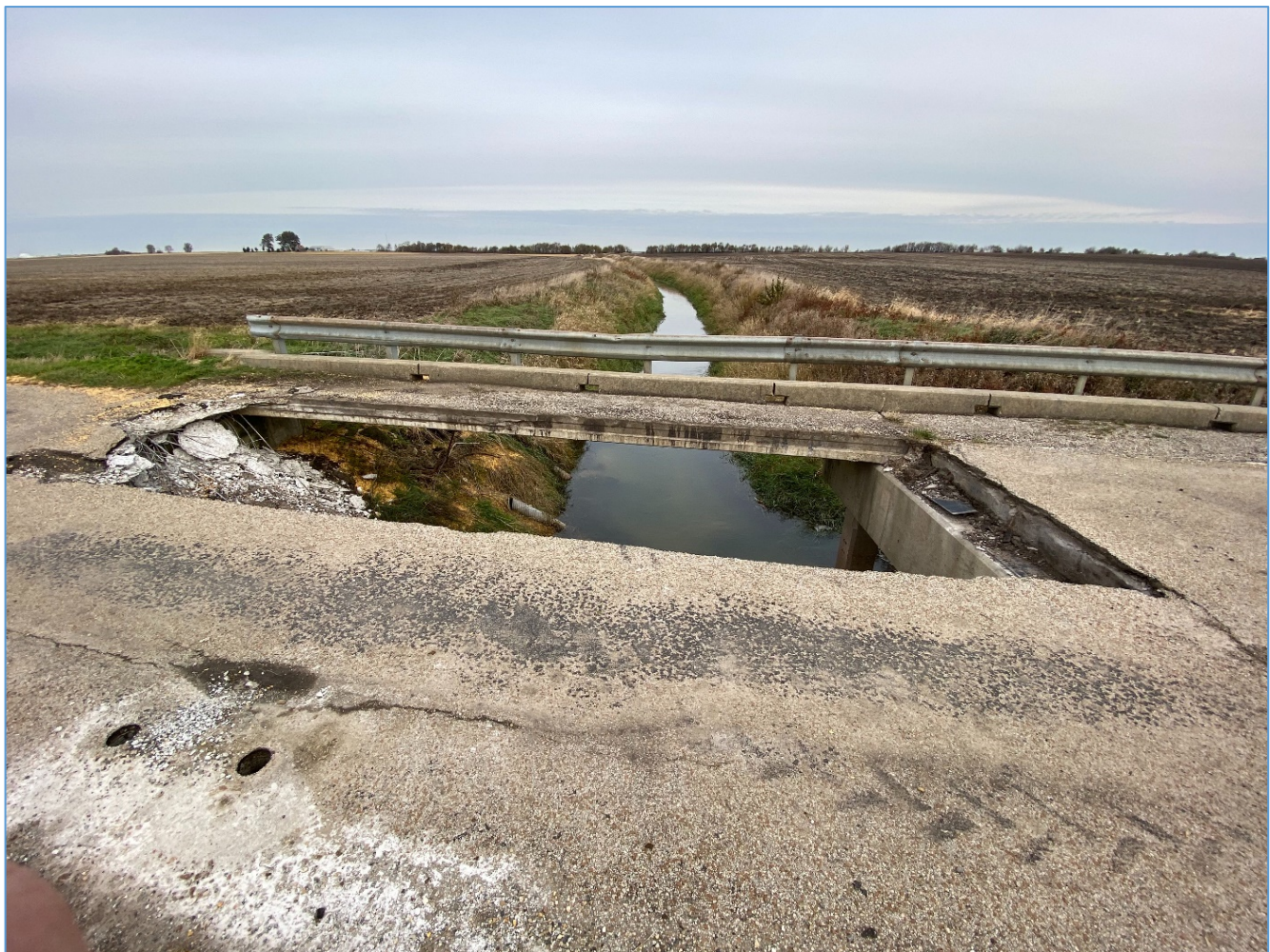
Figure 3. Photo. A picture of structure number 020-3087 after the failure of two beams, taken in November 2019 by the authors.
