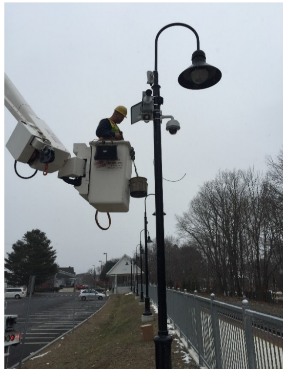
Figure 6 – Freeport Camera Pole
