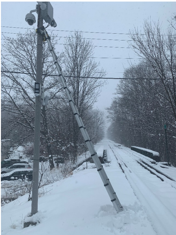
Figure 5 – Jordan Avenue Camera Pole
