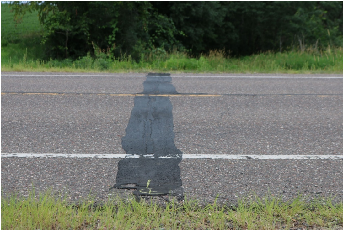
Figure 22 – Pavement Condition with Sealed Cross Crack Directly above Culvert 1, with Additional, Smaller Cracks Nearby
