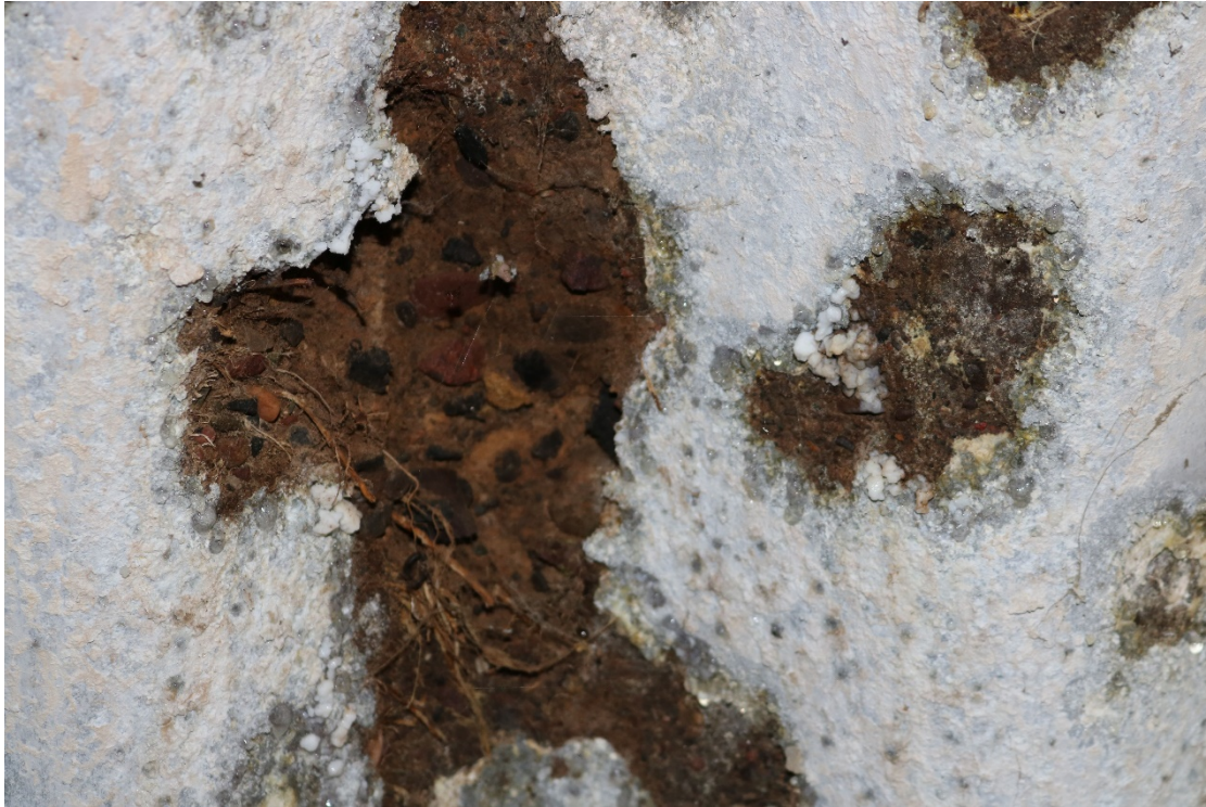
Photo 19 Close-up views of edges of pits with white corrosion products.
