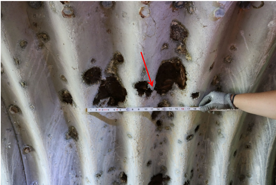
Figure 21 – Coalesced Through-Wall Pitting Corrosion below Roadway Shoulders at Springline of Culvert 1 (East Shoulder Shown); Red Arrow Indicates Location where Small Sample of Corrosion Products and Corroded Aluminum Was Removed for Laboratory Examination (see Section 5.4)
