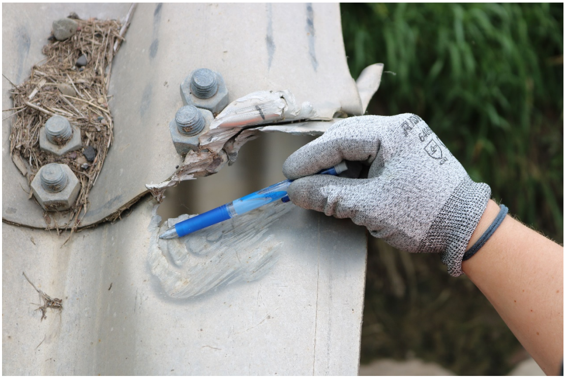
Photo 20 Area of previous damage at east end of culvert from which a small sample was removed for laboratory examination of uncorroded aluminum.
