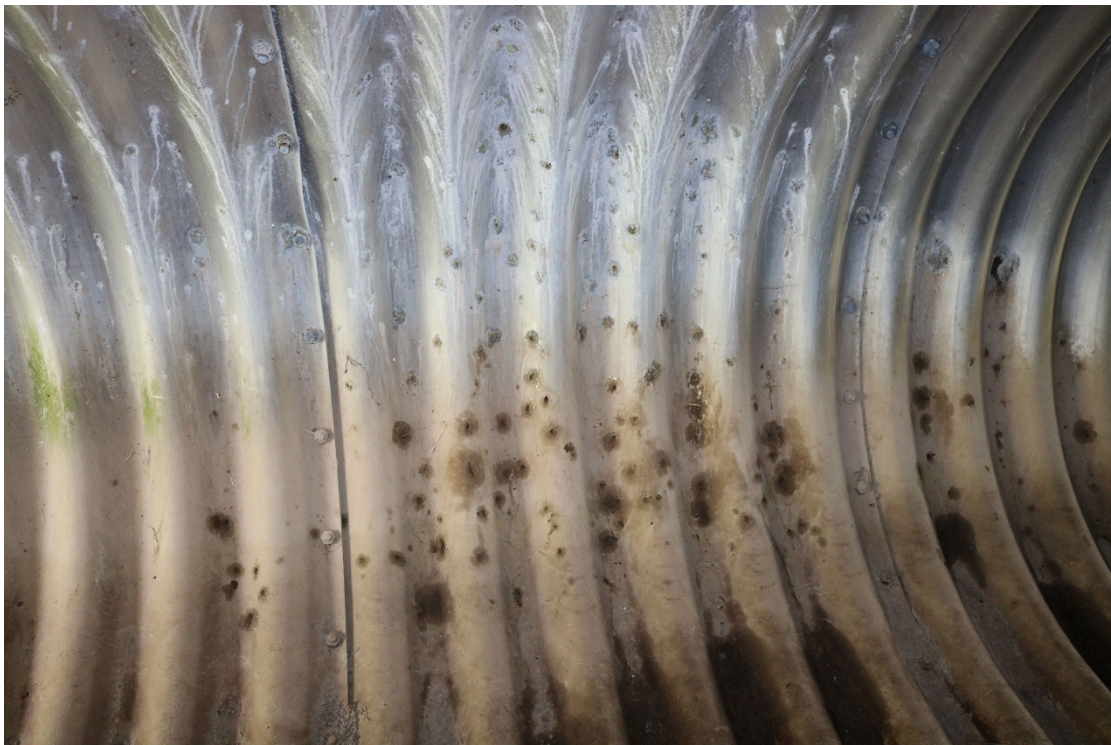
Photo 12 Area of through-wall pitting and corrosion staining at north springline, below west shoulder.
