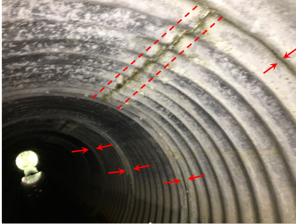
Figure 27 – Heavy White Corrosion Staining Emanating from Longitudinal Seam (between Dashed Red Lines) and at Circumferential Seams (between Pairs of Red Arrows) Further Into Photo; Photo Location Is Below Roadway Travel Lane
