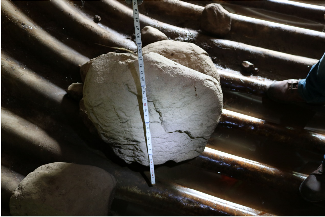
Photo 17 Boulders at invert of culvert.
