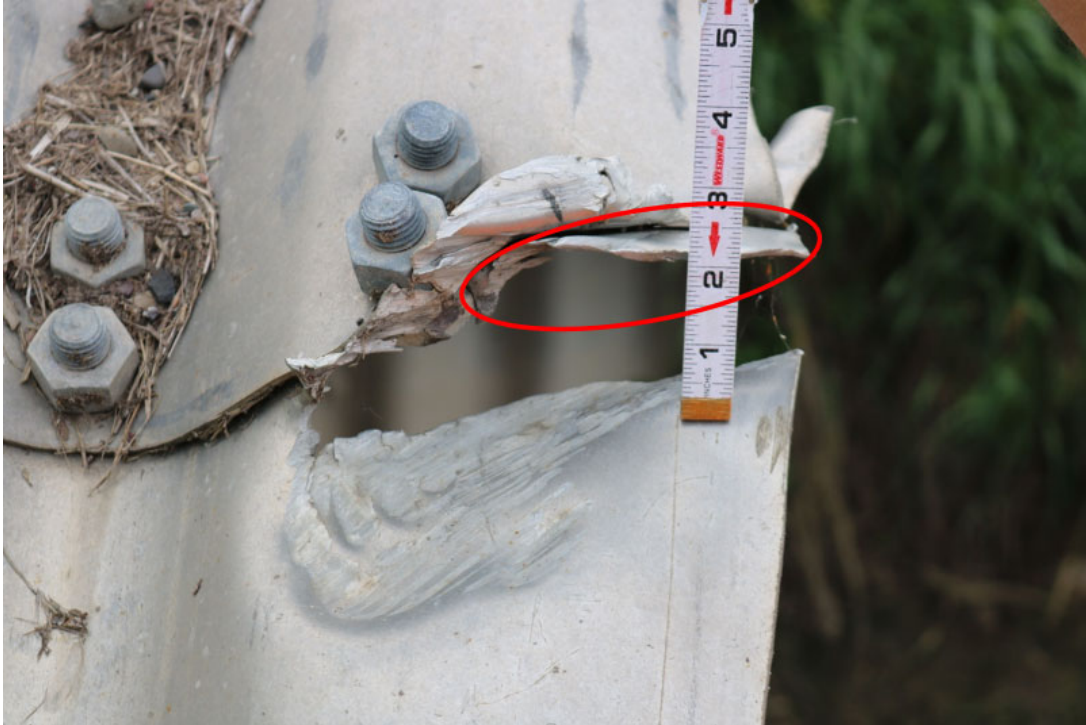
Figure 29 – Previously Damaged Location from which Small Sample of Uncorroded Aluminum Was Removed from Culvert 1 for Laboratory Examination (Red Oval)
