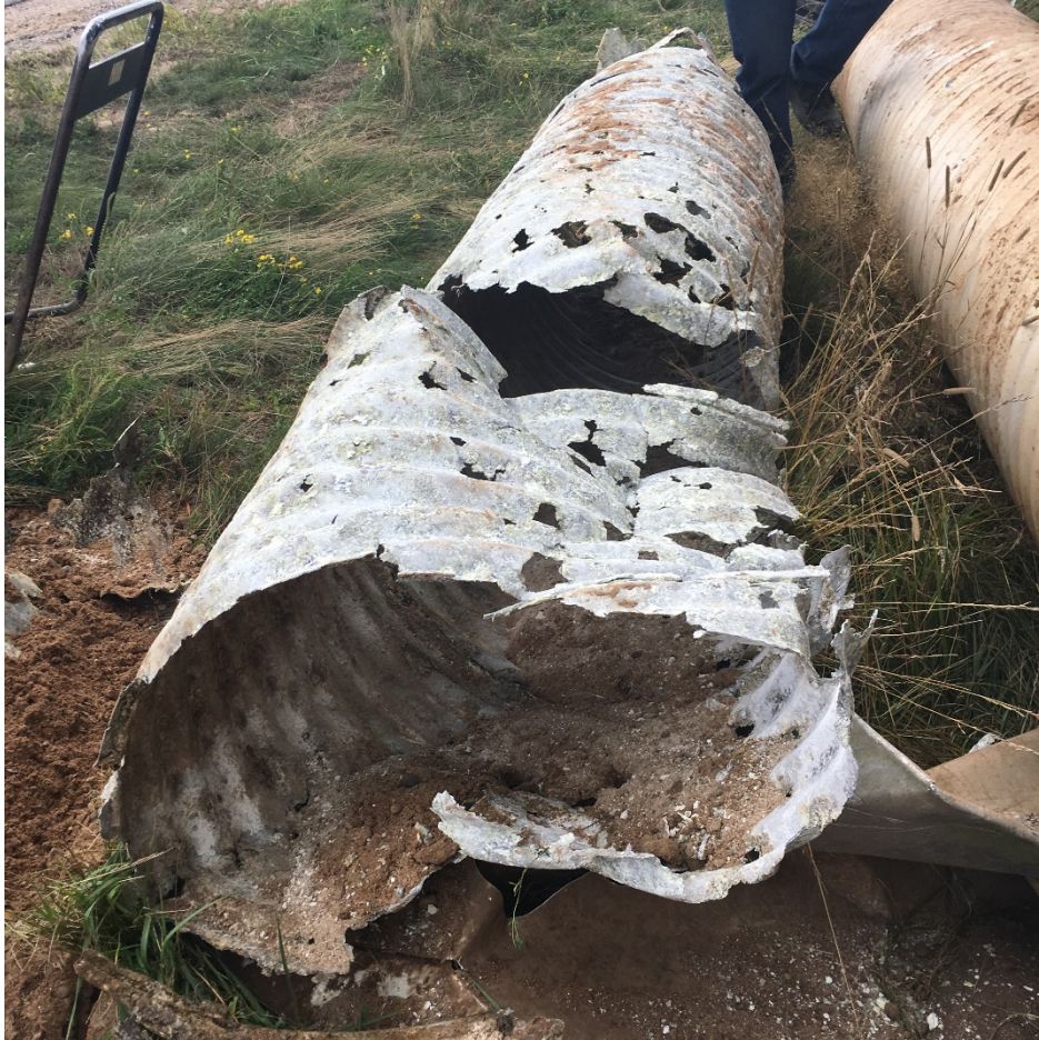
Figure 15 – Photo of Corroded Aluminum Pipe after Removal for Replacement in North-Central Wisconsin in August 2018 on State Highway 32 (Wisconsin DOT Photo)
