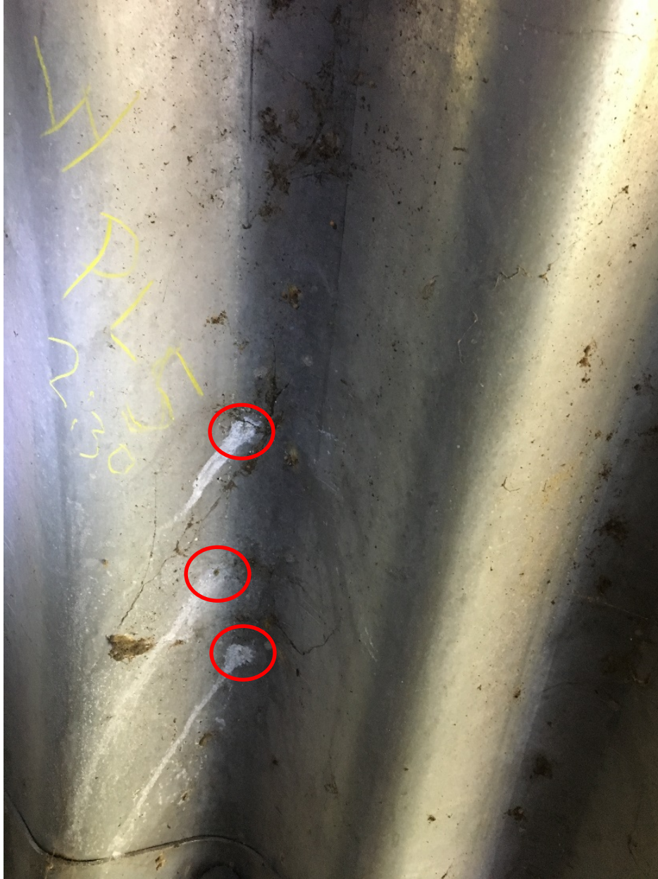
Figure 24 – White Corrosion Staining Emanating from Approximately Quarter-Sized Areas of Likely Pitting Corrosion (Red Circles) Near Mid-Length of West Barrel at 2:30 Clock Position (Looking Downstream)
