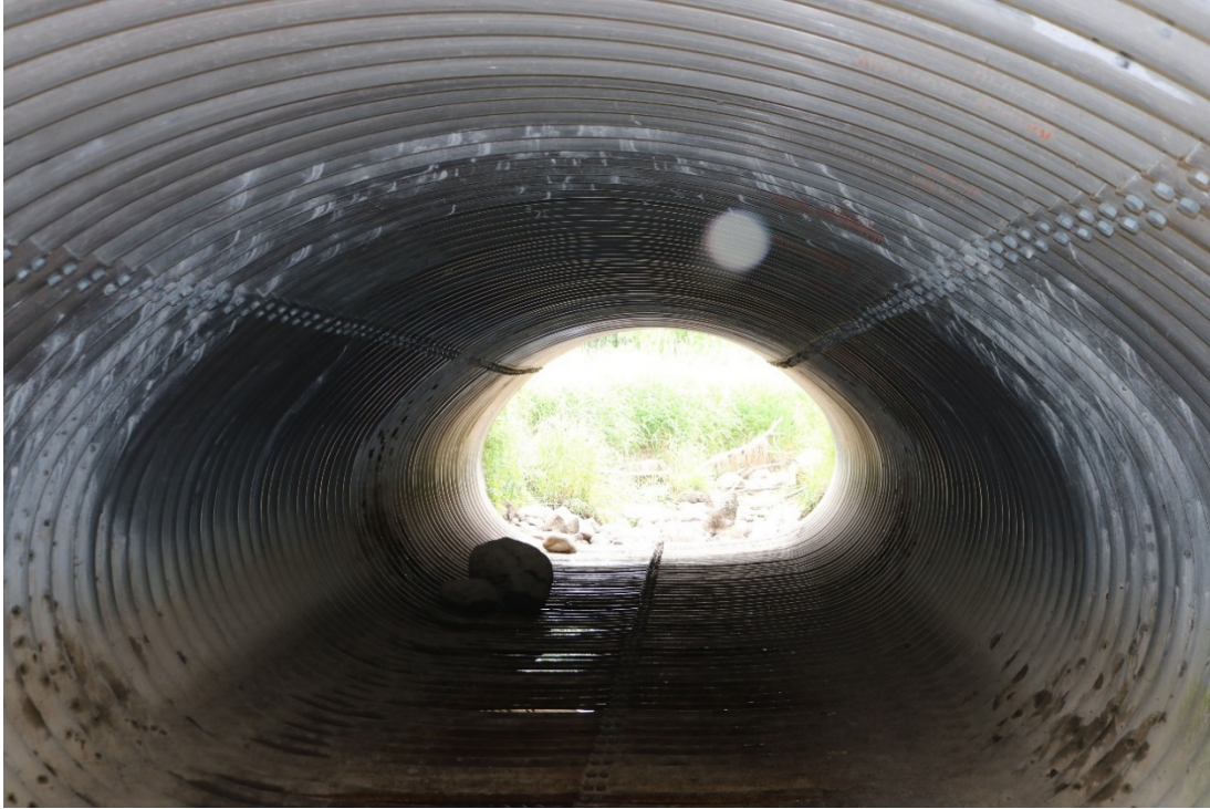
Figure 20 – Pitting Corrosion with White Staining below West Roadway Shoulder in Culvert 1; Similar Area Exists at Far Shoulder in Photo
