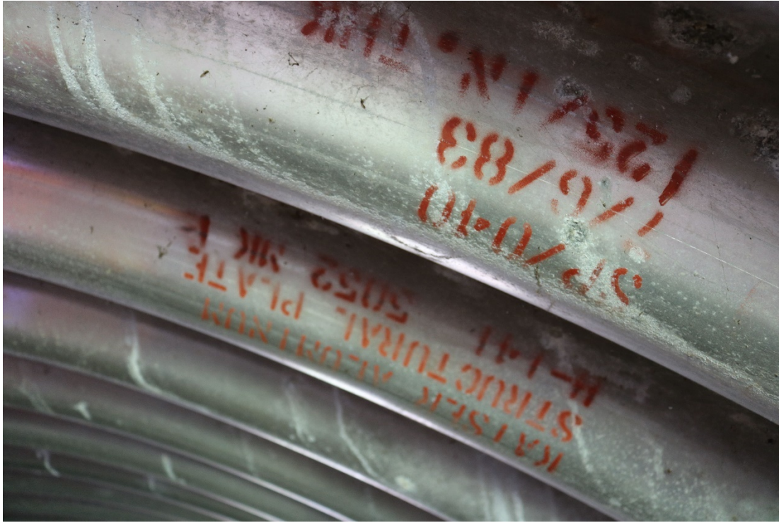
Photo 11 Close-up view of marking.
