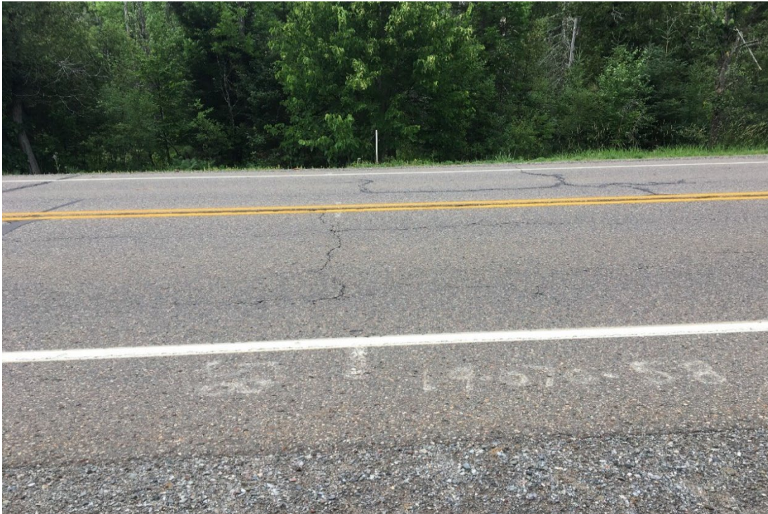
Figure 28 – Pavement Condition over Culvert 3 Showing Unsealed Cracks Across and Along Roadway
