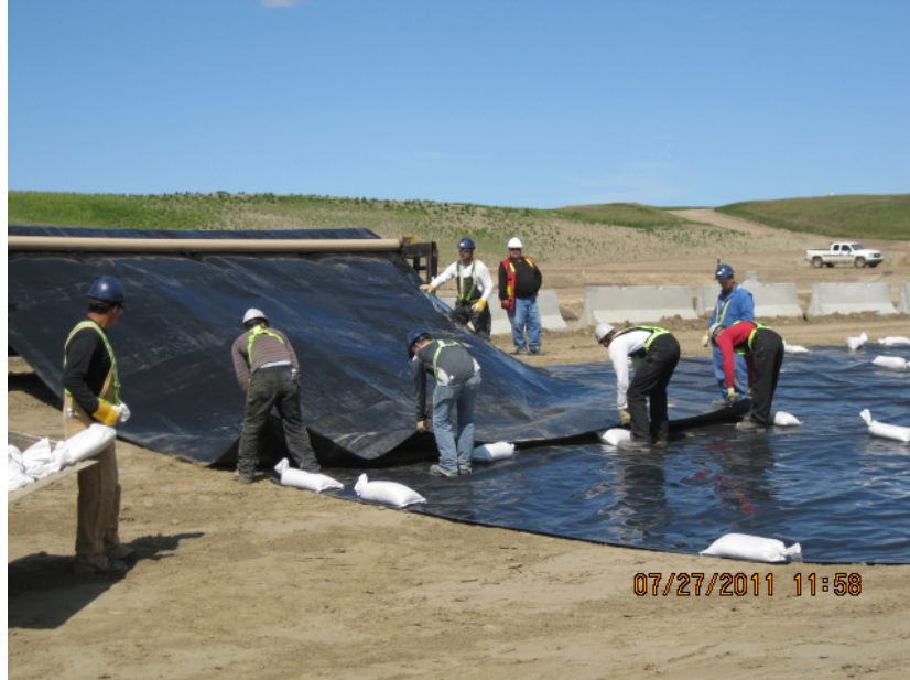
Figure 8 – Membrane Installation Adjacent To and Over Culvert (Courtesy of Big R Bridge)
