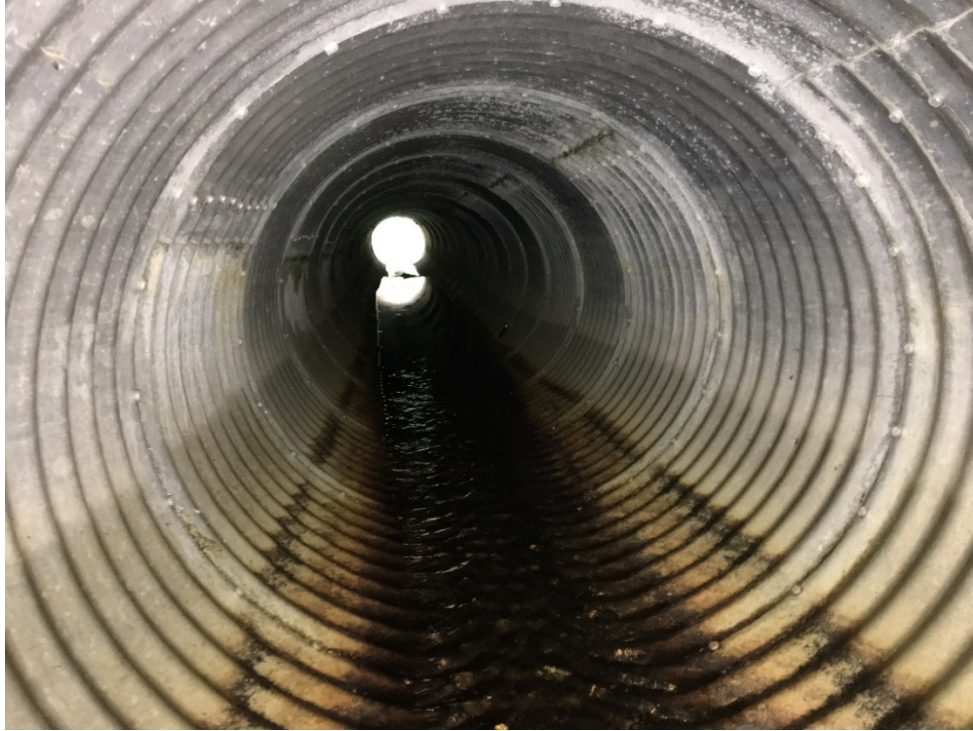
Figure 25 – Typical View Inside Culvert 3 with Riveted Circumferential Seams at 24 In. On Center and One Longitudinal Seam per 24 In. Long Ring; Note White Staining Emanating from Seams
