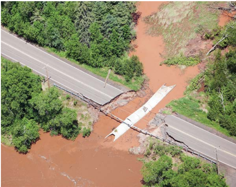
Figure 1. Roadway damage caused by increased flooding is a predicted outcome of climate change.
