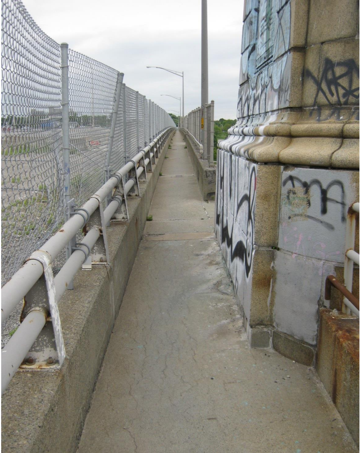
Figure 24. Limited accommodations for pedestrians and bicyclists were available on the bridge prior to this project. Image courtesy of Rhode Island DOT.
