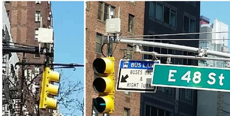
Figure 1. A Roadside Unit (RSUs) installed in New York City (Source: New York City DOT)
