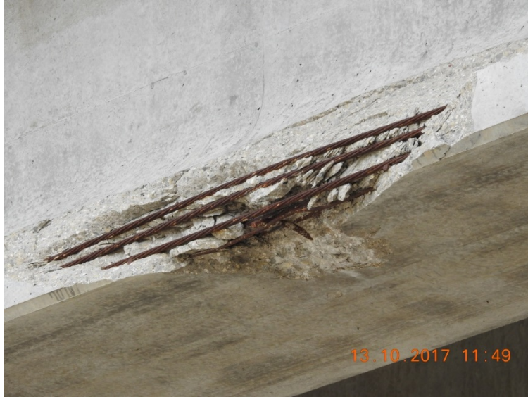
Figure 3.7. Impact damage to bottom flange of Girder 4 in B-20-157 (initial strike)
