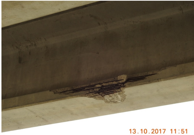
Figure 3.8. Damage to the bottom flange of Girder 1 in B-20-157 (rebound impact)
