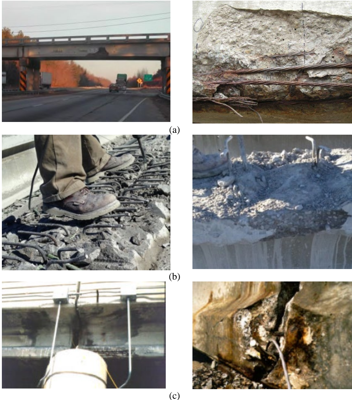
Figure 1.1. Modes of damage to prestressed girders: a) Accidental over-height vehicle impact (Harries 2006); b) Unintended damage during deck slab removal (Assad, 2014); and c) Corrosion damage to prestressed beam ends (Tabatabai et al., 2005)
