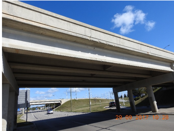
Figure 3.5. Bridge B-40-485 with minor damage on the prestressed girder
