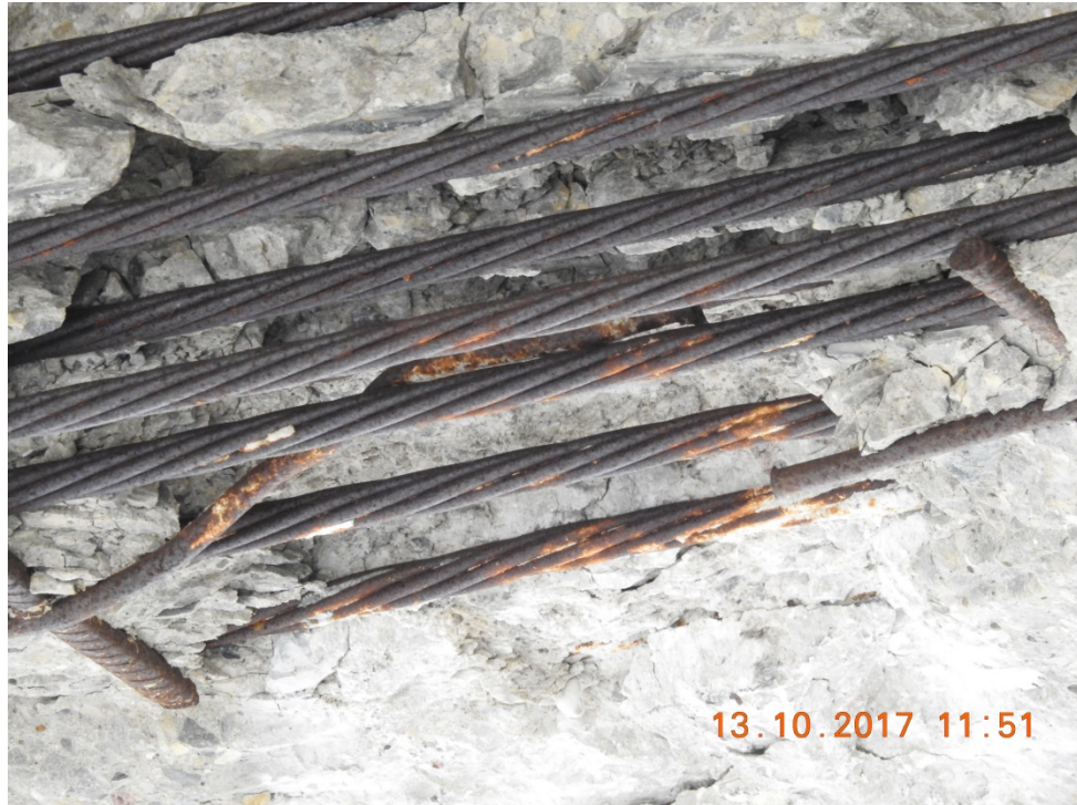
Figure 3.9. Corrosion of prestressing strands and reinforcing steel in Girder 4 on B-20-147
