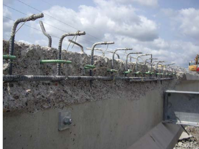
Figure 3.1. Damage to the top flange of prestressed concrete girder on B-64-122 resulting from deck removal.
