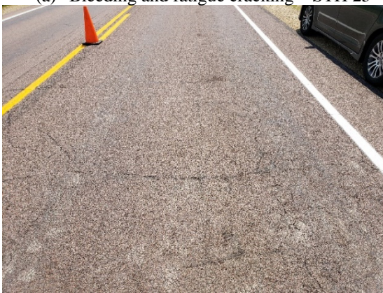
(c) Fatigue cracking – STH 25
