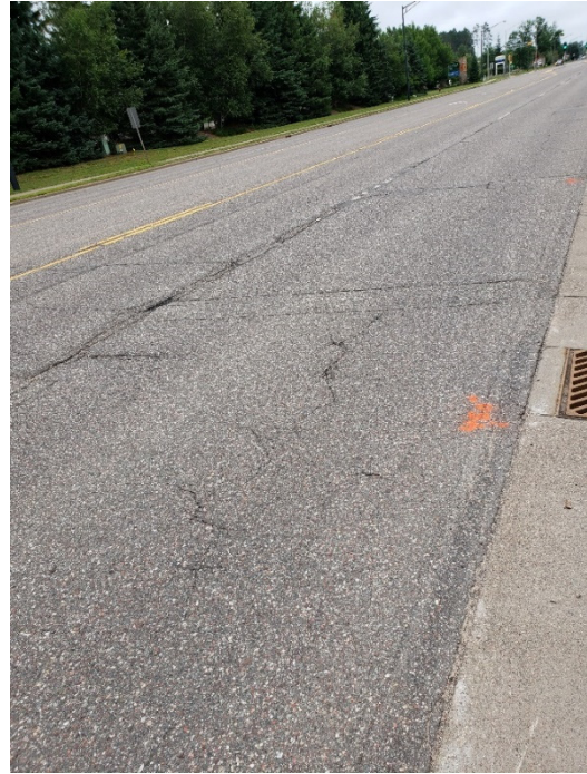
(b) Fatigue cracking STH 70
