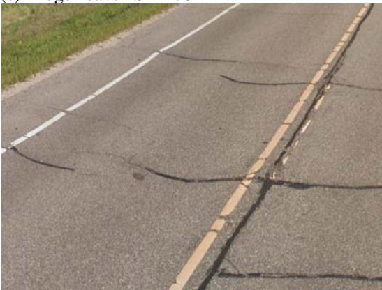
(e) Longitudinal and transverse cracking – STH 78
