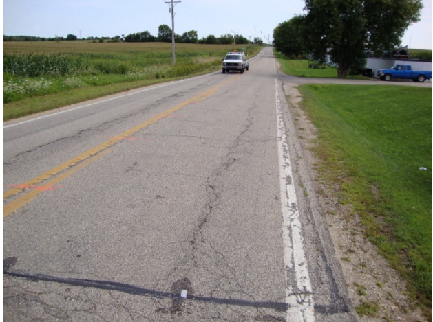
(a) Pavement section I with CA base layer in 2009 before mill and relay
