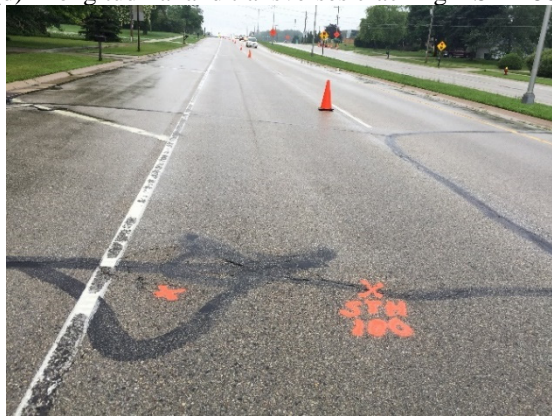
(f) Longitudinal and transverse cracking – STH 100
