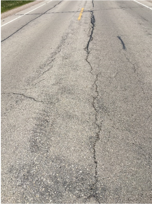
(a) Fatigue cracking – STH 96
