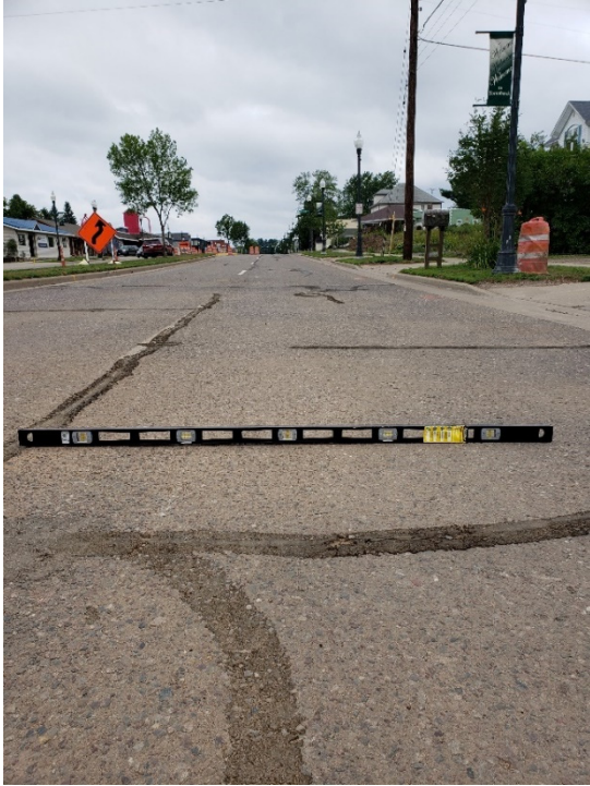
(a) Rutting – STH 86
