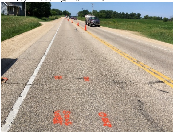
(e) Fatigue and transverse cracking – STH 22
