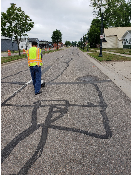
(b) Longitudinal and transverse cracking – STH 86
