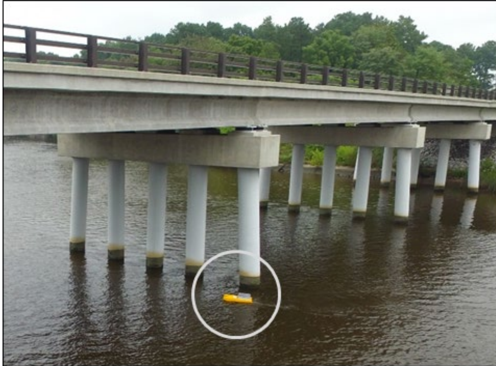
Figure 20. Photo. UWS platform collecting data at the Tuckahoe Creek bridge site. (UWS is highlighted in the grey circle).
