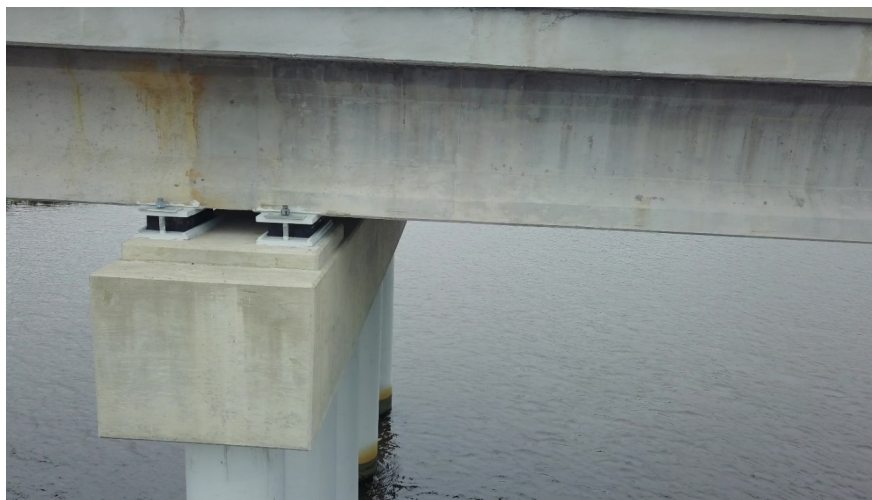
Figure 31. Photo. DJI Mavic imagery of a pier cap and the side of the bridge.
