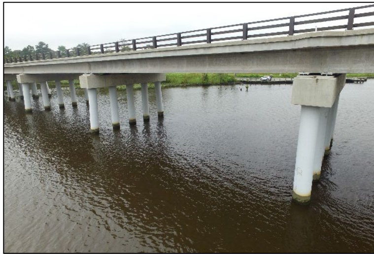
Figure 30. Photo. Close-up photo of the Tuckahoe Creek Bridge taken with the Phantom 3A UAS.
