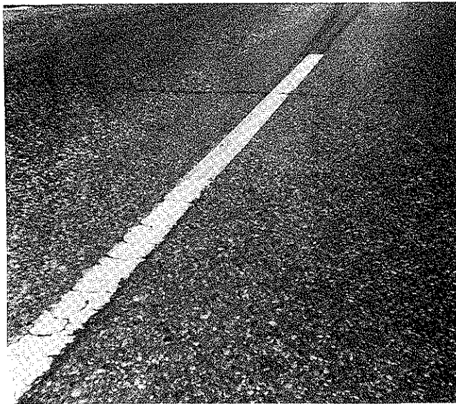
Figure 4 ETP on Bituminous Concrete Pavement (US 40 Colorado) After 30 Months (ETP Stripes in Background).
