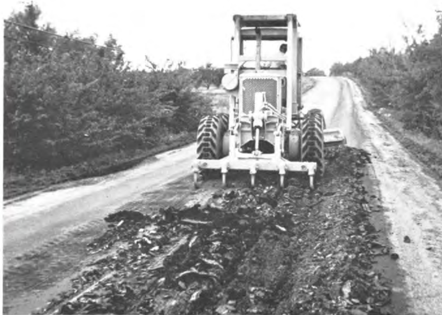
The first step in the recycling process was to rip the existing pavement with rear-mounted ripper teeth on a motor grader.
