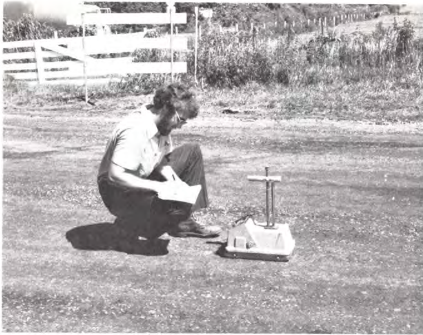
Density tests were taken with a Troxler nuclear gauge to assure uniform compaction.
