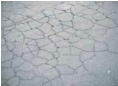
Figure 4.81: AC Chicken Wire/Alligator Fatigue Type Cracking in Wheel path
