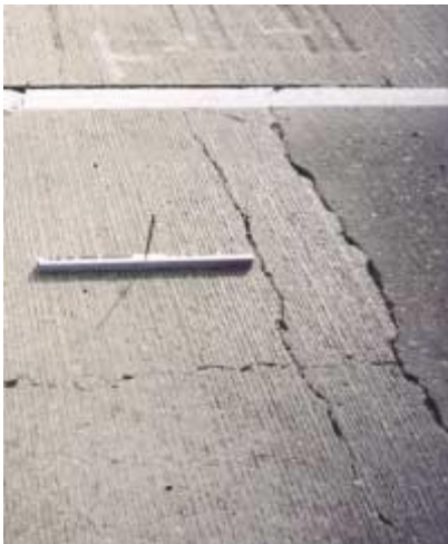
Figure 4.87: Moderate Severity CRCP Punchout Cracking
