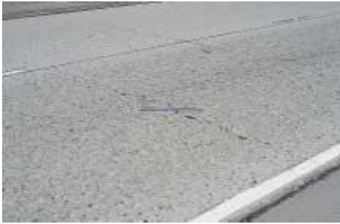
Figure 4.95: JCP High Severity Transverse Cracking
