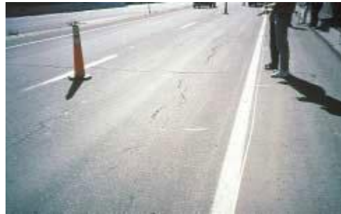
Figure 4.82: AC Low Severity Fatigue Type Cracking
