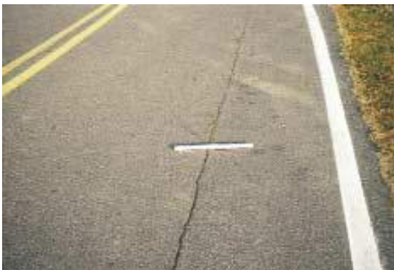
Figure 4.80: AC Moderate Severity Longitudinal Cracking (Wheel path)
