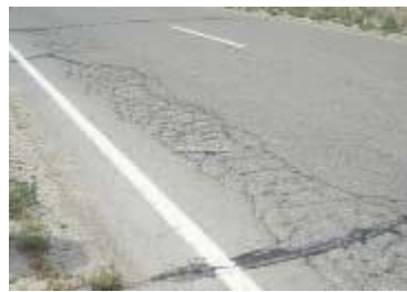
Figure 4.84: AC High Severity Fatigue Type Cracking
