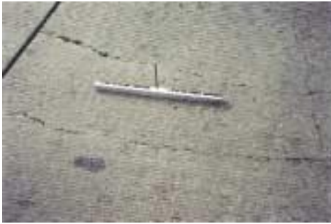
Figure 4.86: Low Severity CRCP Punchout Cracking
