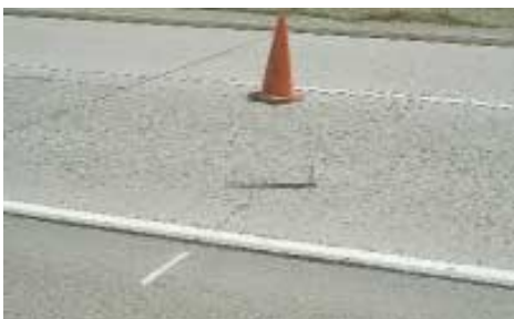
Figure 4.94: JCP Moderate Severity Transverse Cracking
