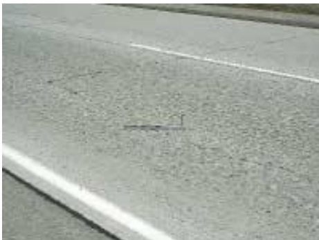
Figure 4.91: JCP Moderate Severity Longitudinal Cracking
