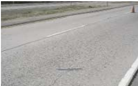
Figure 4.90: JCP Low Severity Longitudinal Cracking
