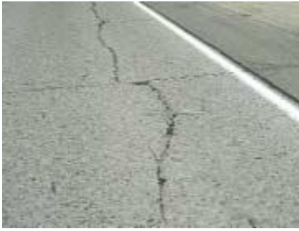
Figure 4.92: JCP High Severity Longitudinal Cracking
