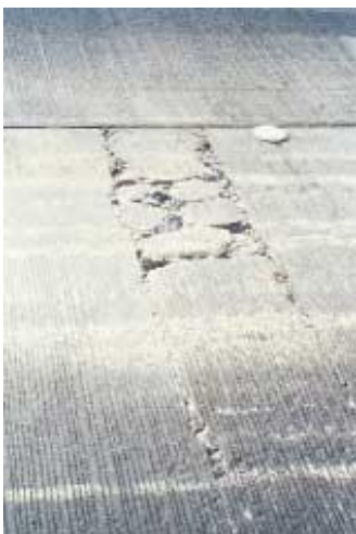
Figure 4.88: High Severity CRCP Punchout Cracking
