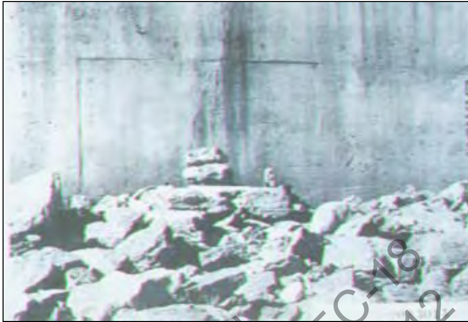
Figure 11.1. Photograph of riprap at pier 2, October 1956. (98,99)
