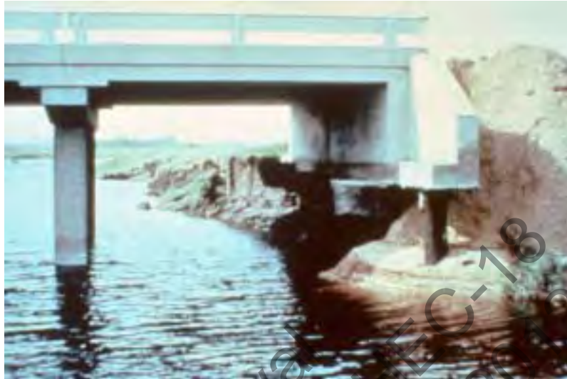
Figure 7.2. Scour of bridge abutment and approach embankment.
