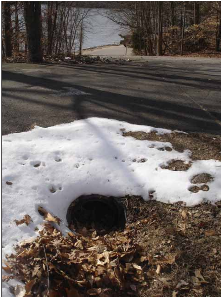
Figure 55. Photo. View of inlet of plastic HDPE example in Fountainhead Regional Park, Fairfax, Virginia.
