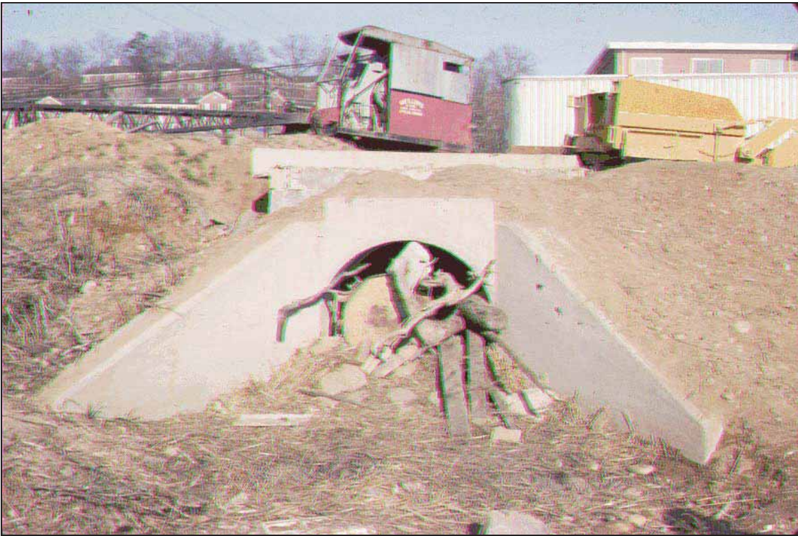
Figure 3. Photo. Example of severe debris blockage. (2)
