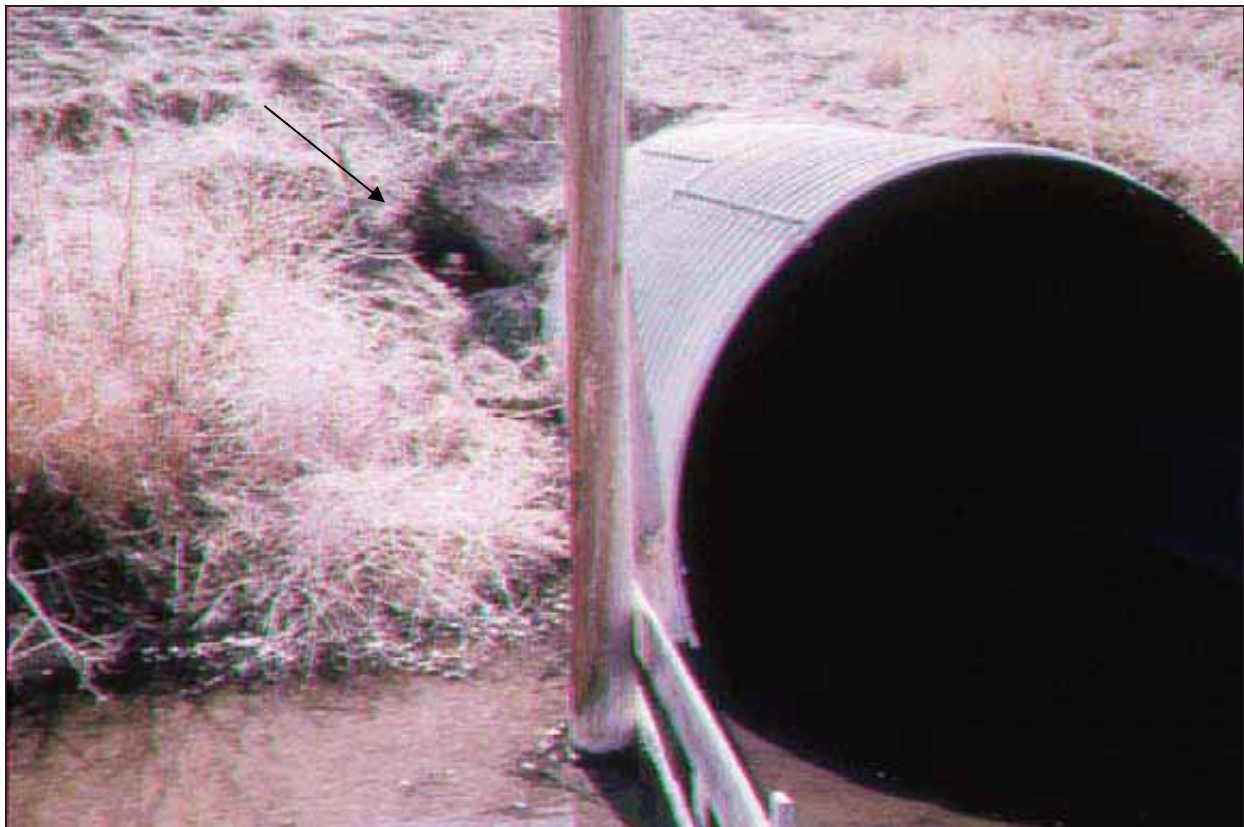
Figure 9. Photo. Example of piping through an embankment. (2)
