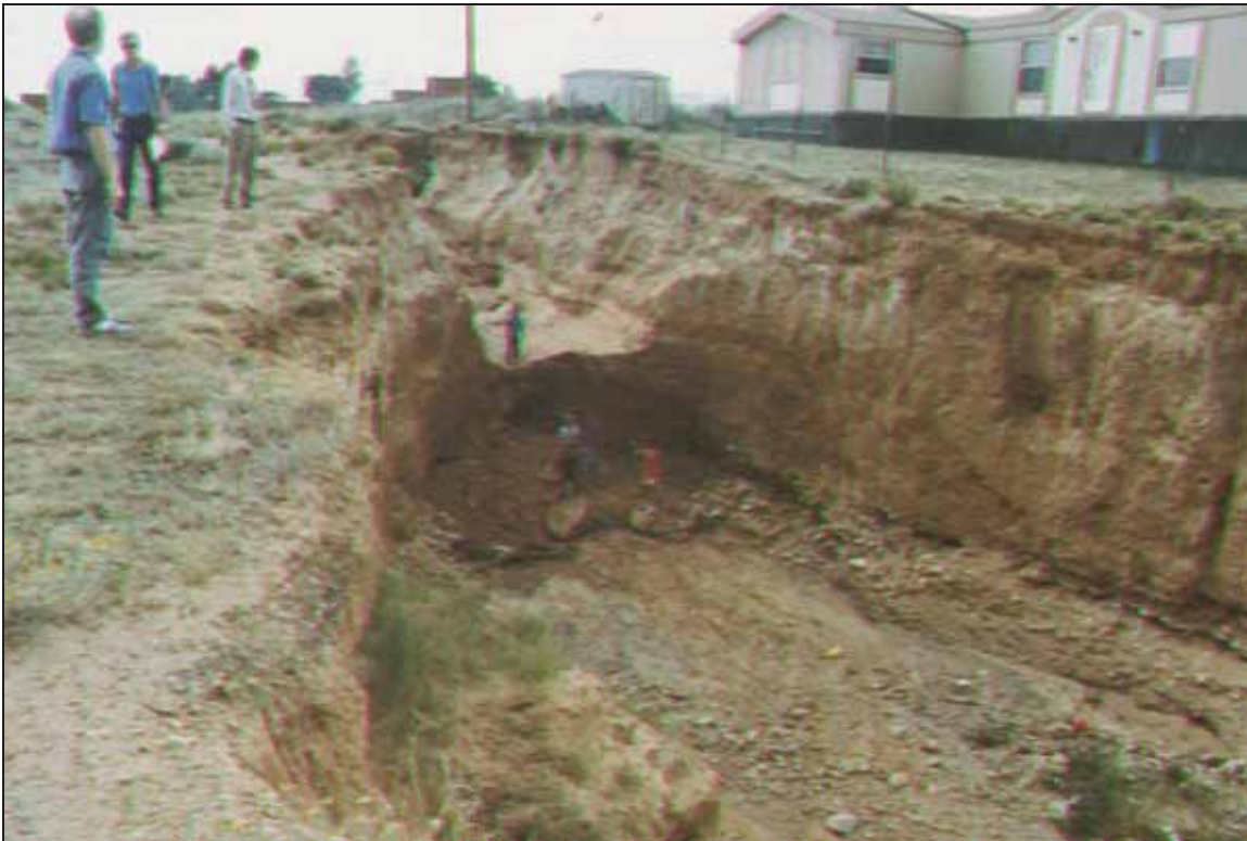
Figure 13. Photo. Example of head cut that can be expected to move upstream over time. (7)
