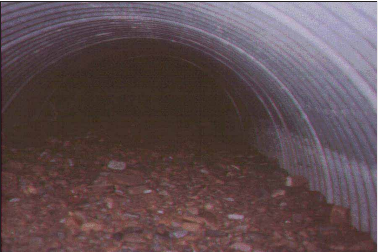
Figure 14. Photo. Culvert barrel filled with sediment up to half its rise, possibly due channel aggradation. (2)
