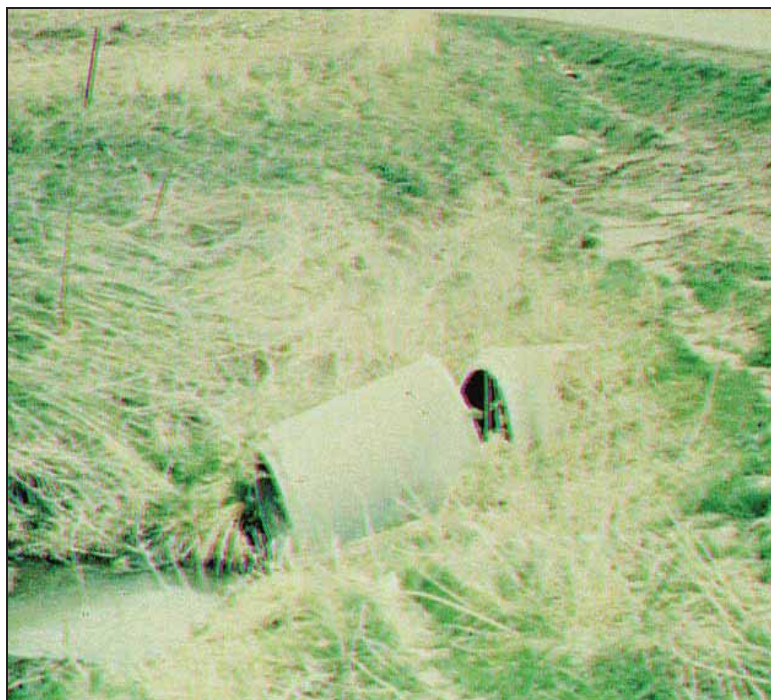
Figure 8. Photo. RCP culvert damaged by scour. (2)
