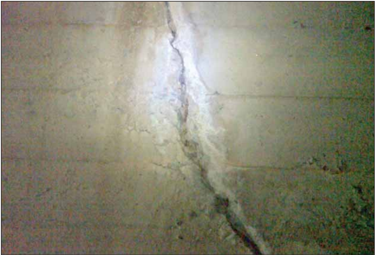
Figure 38. Photo. Vertical crack in culvert wall with exudence.
