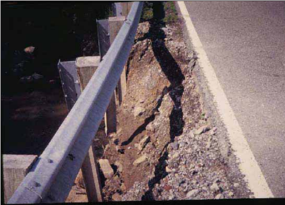
Figure 6. Photo. Erosion damage to downstream embankment slope and shoulder from previous overtopping. (3)
