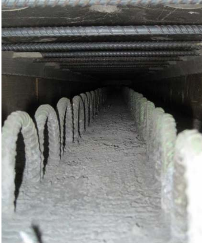
Figure 10. Photograph. Composite connection between concrete girder and precast concrete deck immediately prior to field-casting of UHPC.
