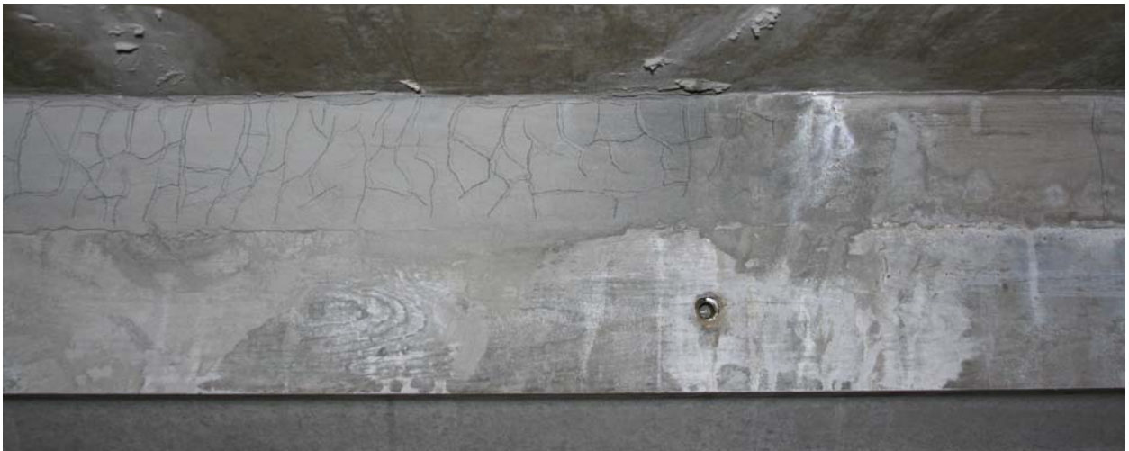
Figure 36. Photo. Cracking apparent on north face of haunch near east end of test specimen.
