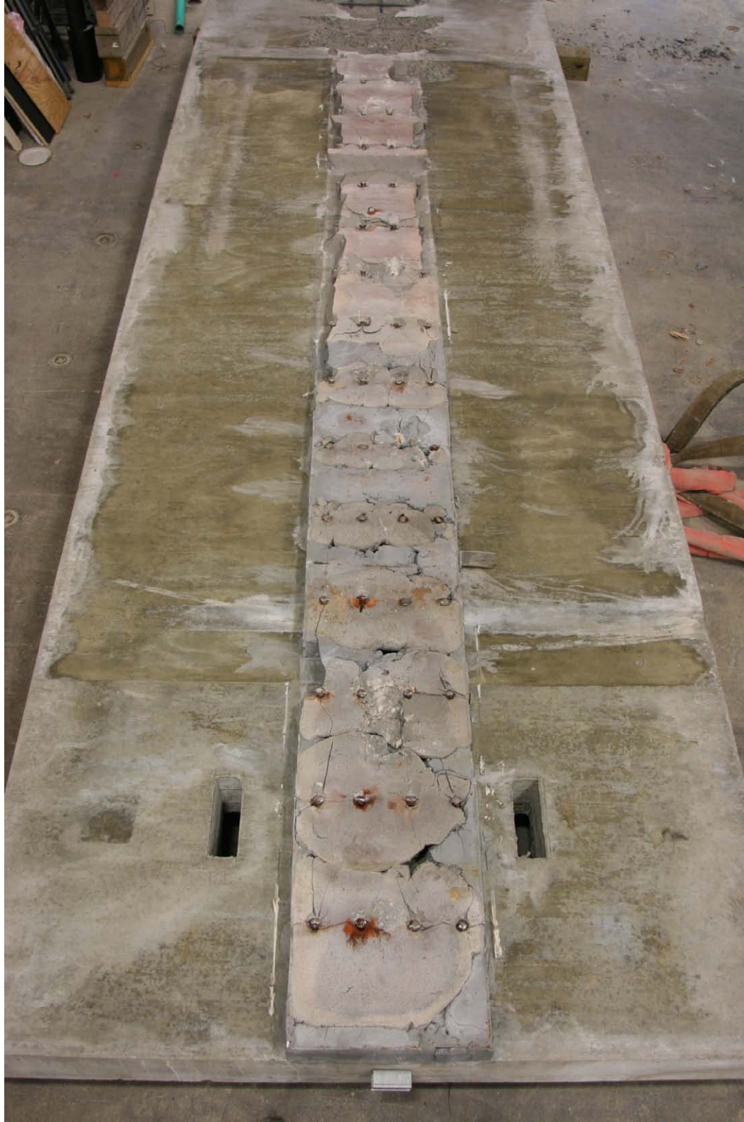
Figure 54. Photo. Emulated steel girder composite connection after completion of test and removal of haunch/deck.
