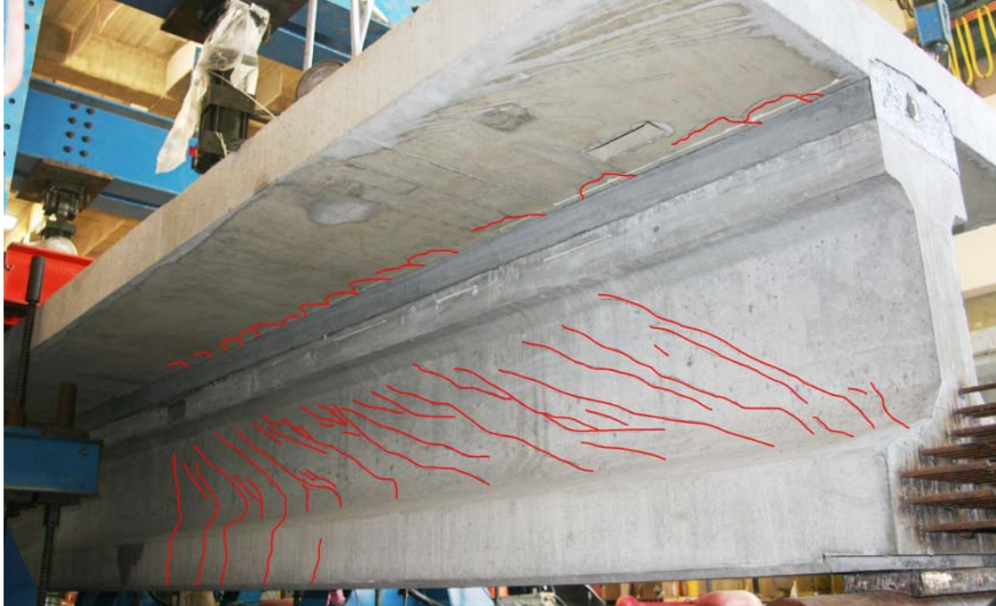
Figure 32. Illustration. Cracking apparent on north face of west end of test specimen after completion of static testing.
