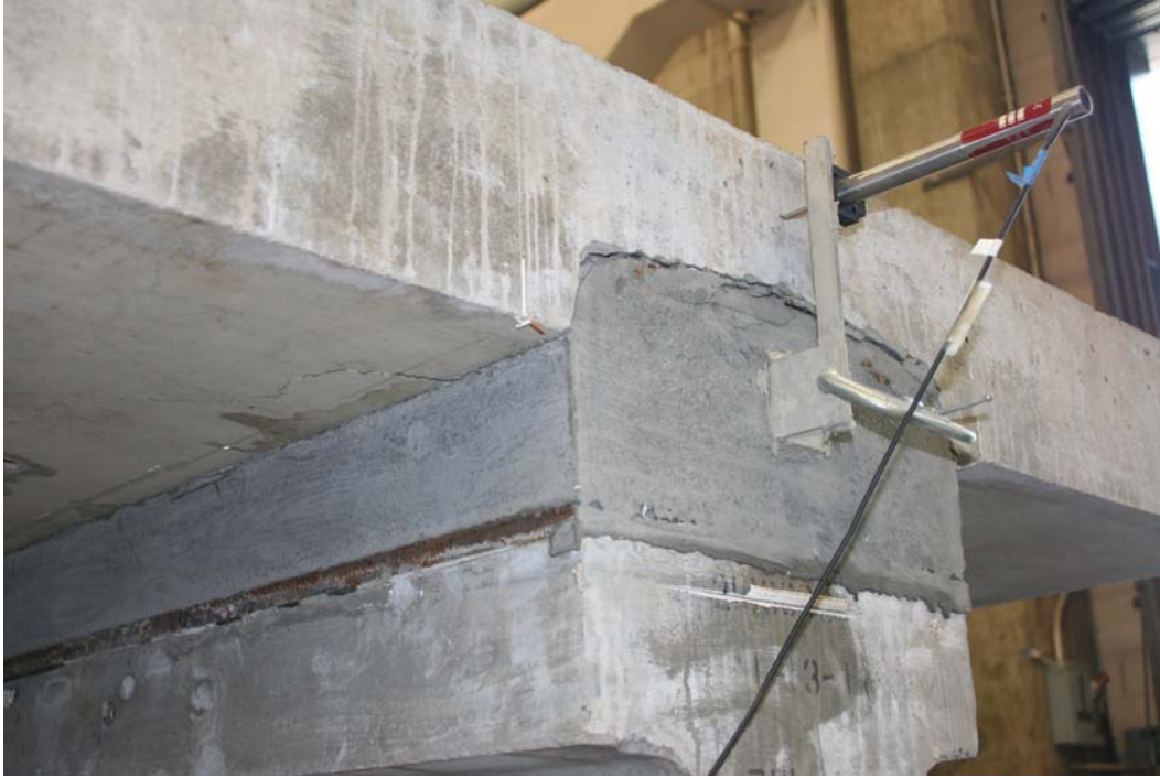
Figure 30. Photo. Haunch connection which emulated the composite connection to a steel girder (i.e., east end) after completion of static testing.
