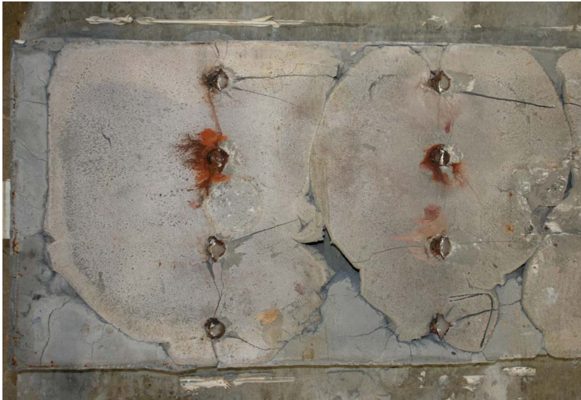
Figure 56. Photo. Easternmost two rows of shear studs emanating from conventional grout and precast deck.
