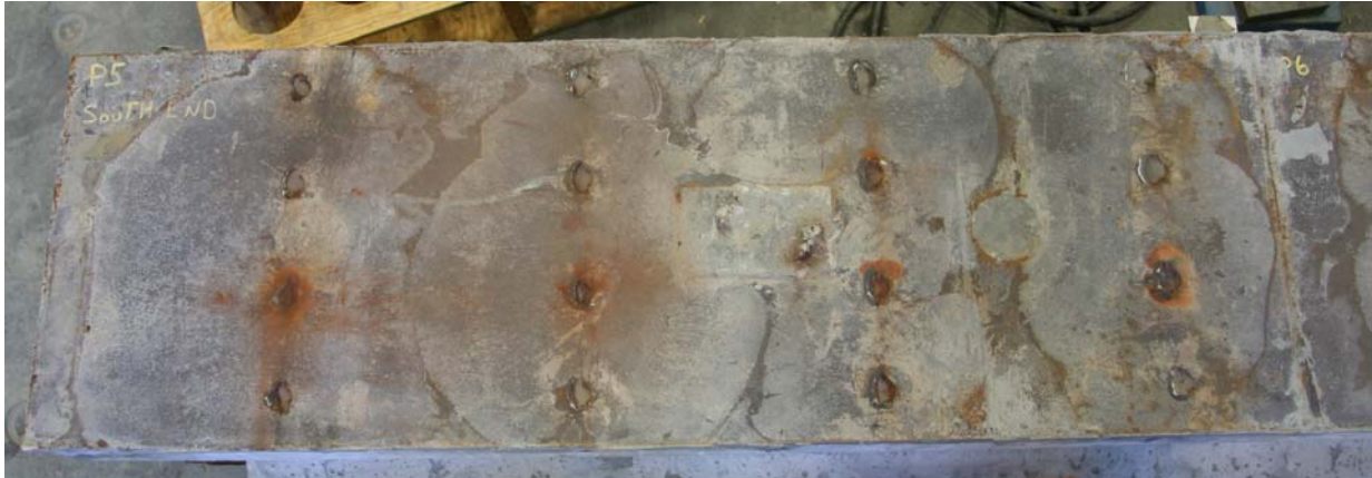
Figure 55. Photo. Easternmost steel plate on top of girder within emulated steel girder composite connection.
