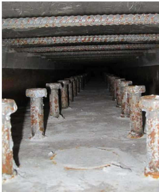
Figure 9. Photograph. Composite connection between emulated steel girder and precast concrete deck immediately prior to field-casting of UHPC.
