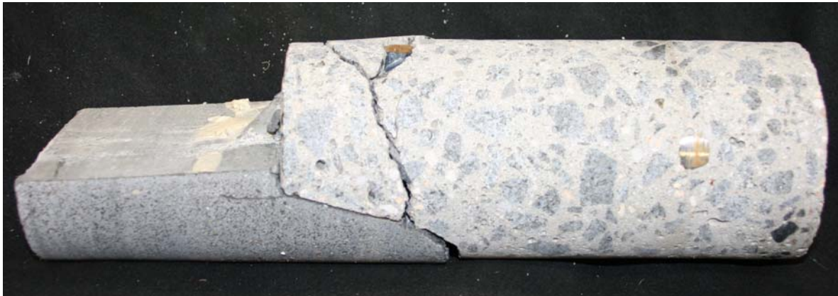
Figure 35. Photo. Distress in core extracted from haunch connection near east end of test specimen.
