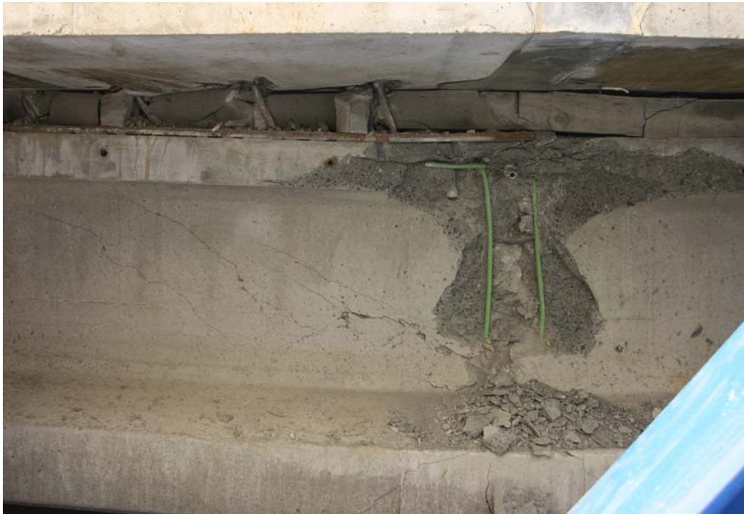
Figure 52. Photo. Midspan north face of test specimen immediately after completion of test.
