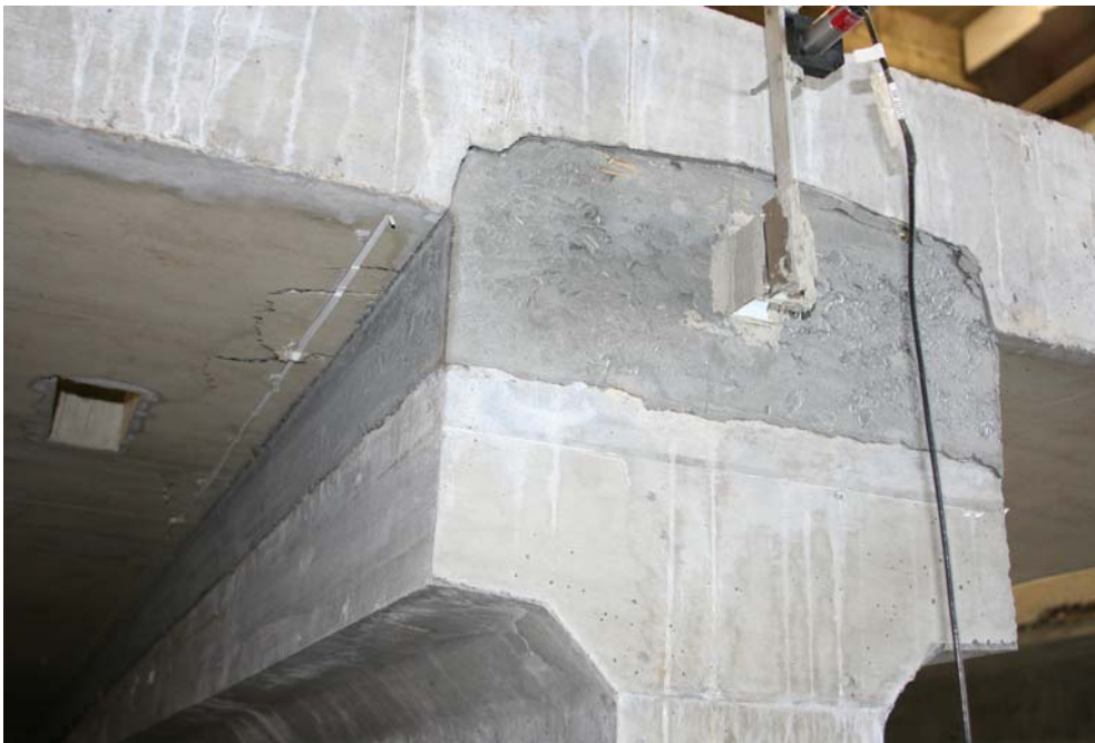
Figure 31. Photo. Haunch connection which emulated the composite connection to a concrete girder (i.e., west end) after completion of static testing.
