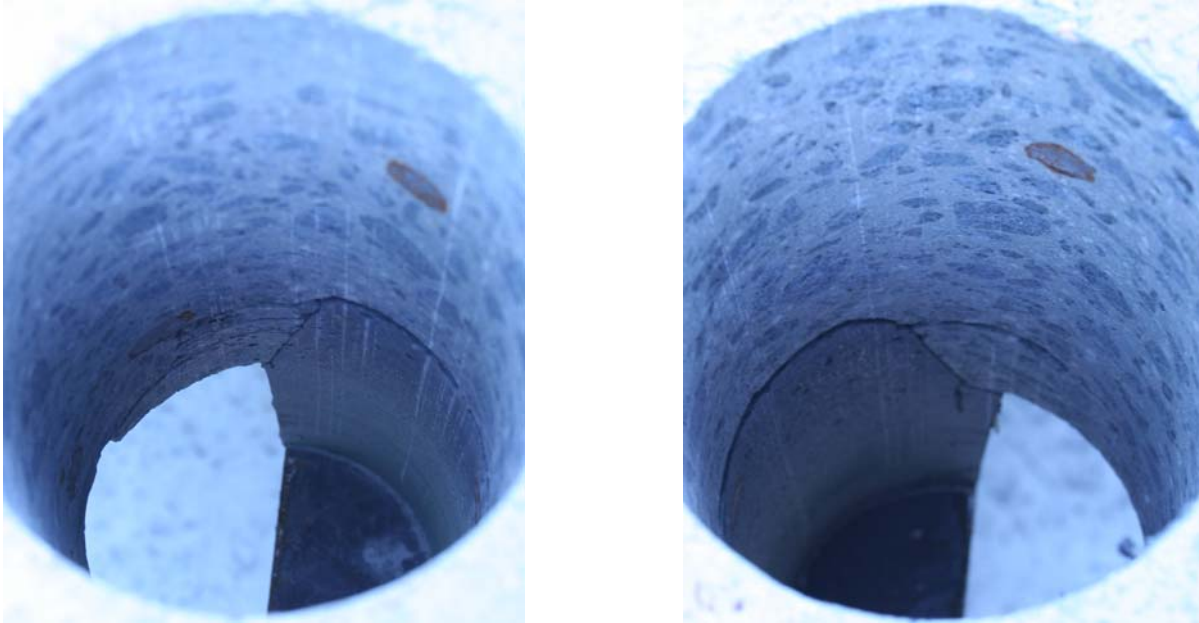
Figure 34. Photo. Distress in deck concrete at haunch connection near east end of test specimen which emulated the composite connection to a steel girder. Left photo pertains to south face. Right photo pertains to north face.
