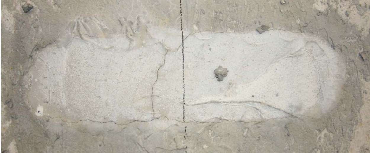
Figure 37. Photo. Cracking apparent on top of deck at grout pocket near east end of test specimen prior to start of structural loading.
