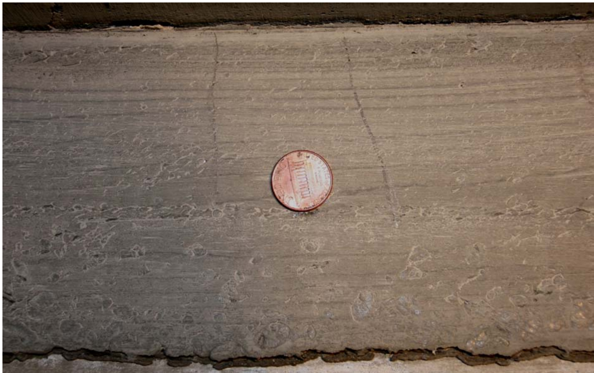
Figure 70. Photo. Shrinkage cracks in haunch on north face near west end of UHPC test specimen.
