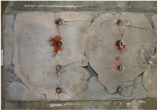
Fig A3. Close-up of the detached stud welds, so called ‘divots’. [Reproduced from Figure 56 of main body of report.]
