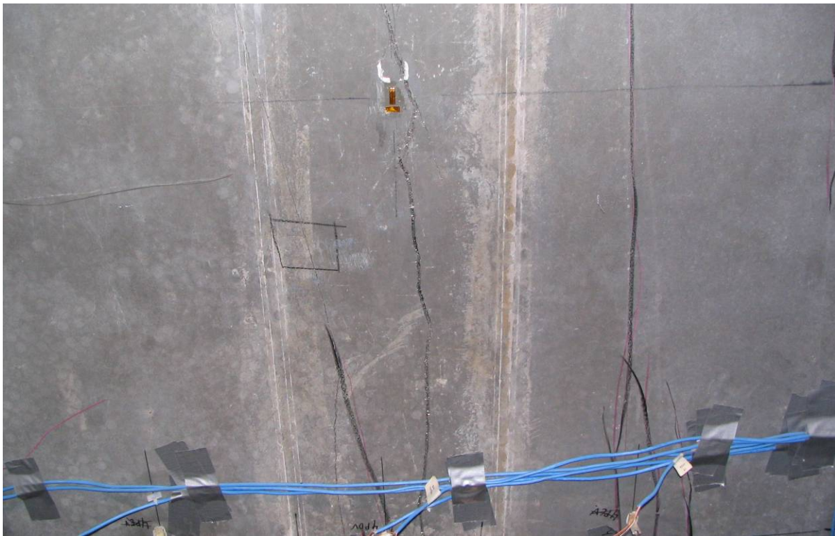
Figure 146. Photo. Longitudinal mid-deck crack on P4-24T after conclusion of test.
