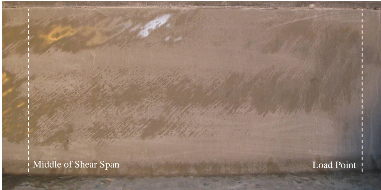
Figure 134. Photo. Cracking on south face of P4-57Ss web at 2,000 kN applied load.
