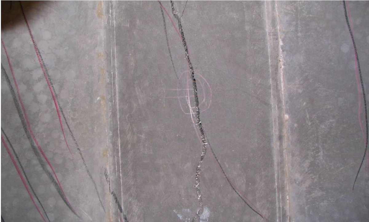
Figure 156. Photo. Longitudinal mid-deck crack on P4-24D after conclusion of test.
