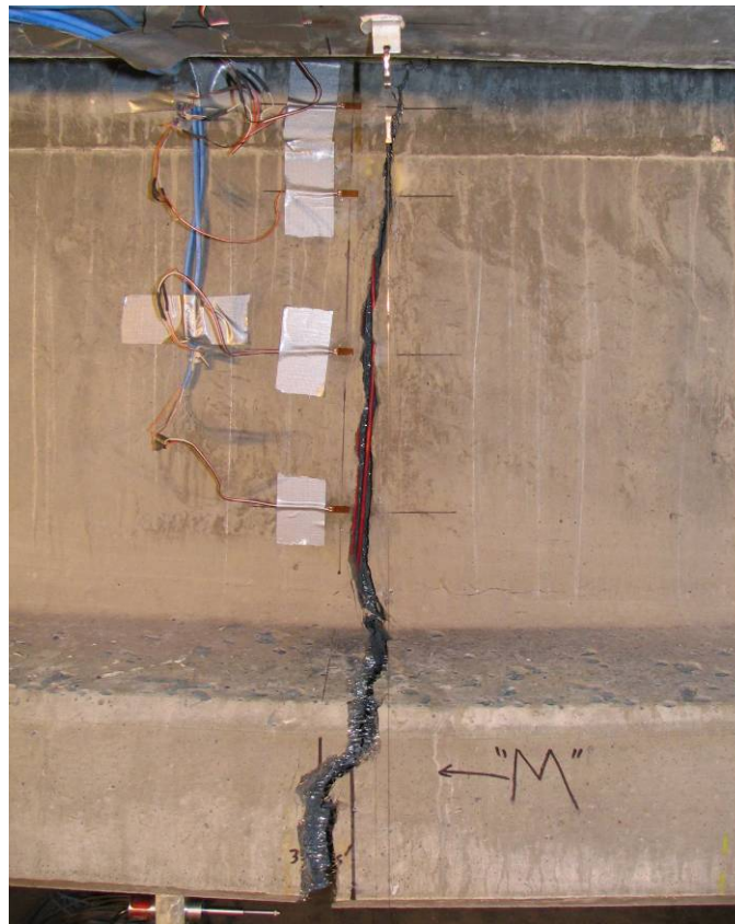
Figure 90. Photo. Crack on south face of Girder P4-45F just after failure.
