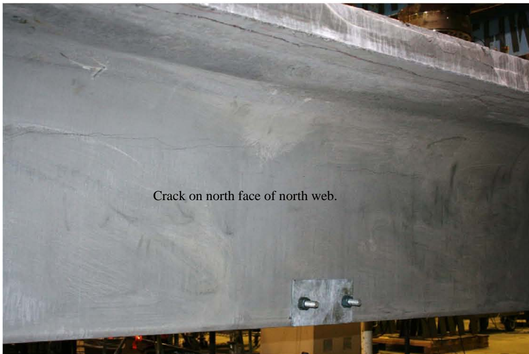
Figure 68. Photo. North face of north web at 1780 kN (400 kips) applied load in Test T1J.
