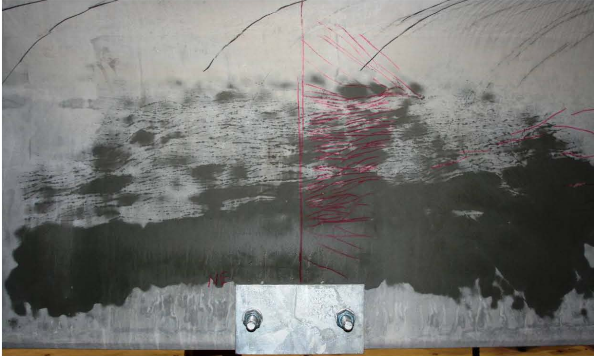
Figure 87. Photo. Cracking on north face of north leg at east diaphragm after conclusion of Test T2J.
