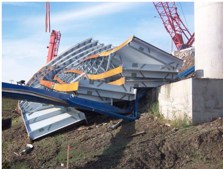
Figure 2.53 Failure of Girders During Construction
