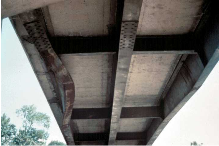
Figure 2.2 Violation of Vertical Clearance Requirement
