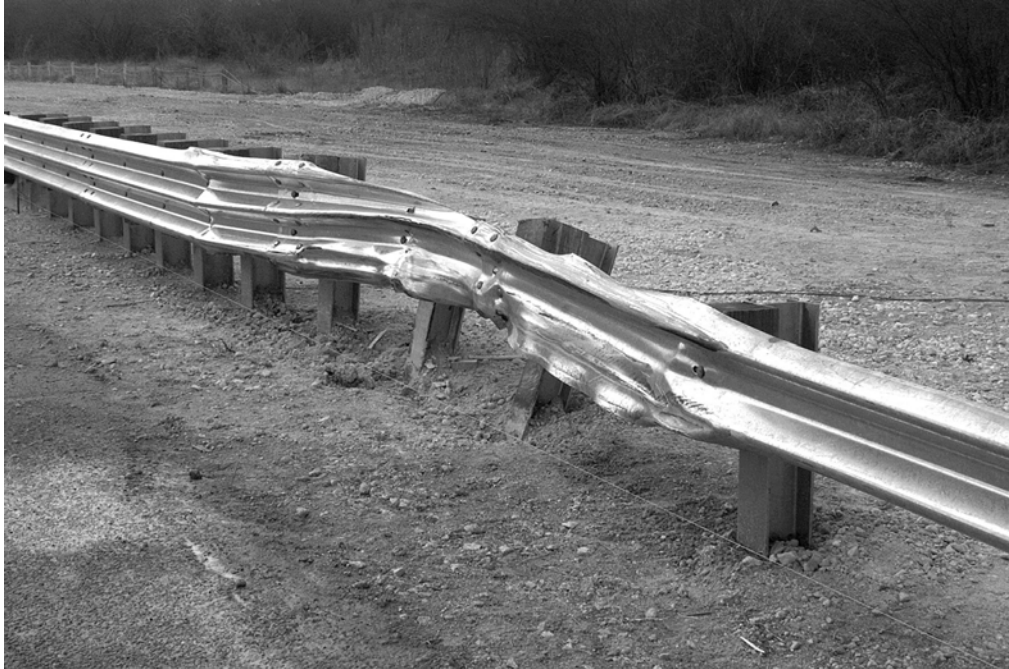
a) Damage at impact.
