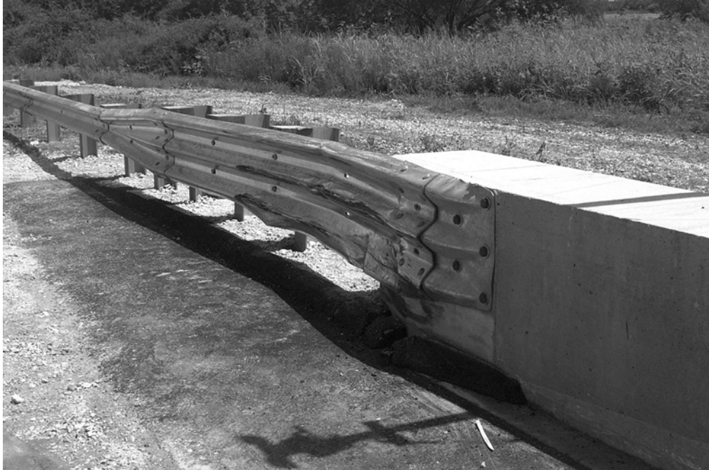
a) Overall view of damage.
