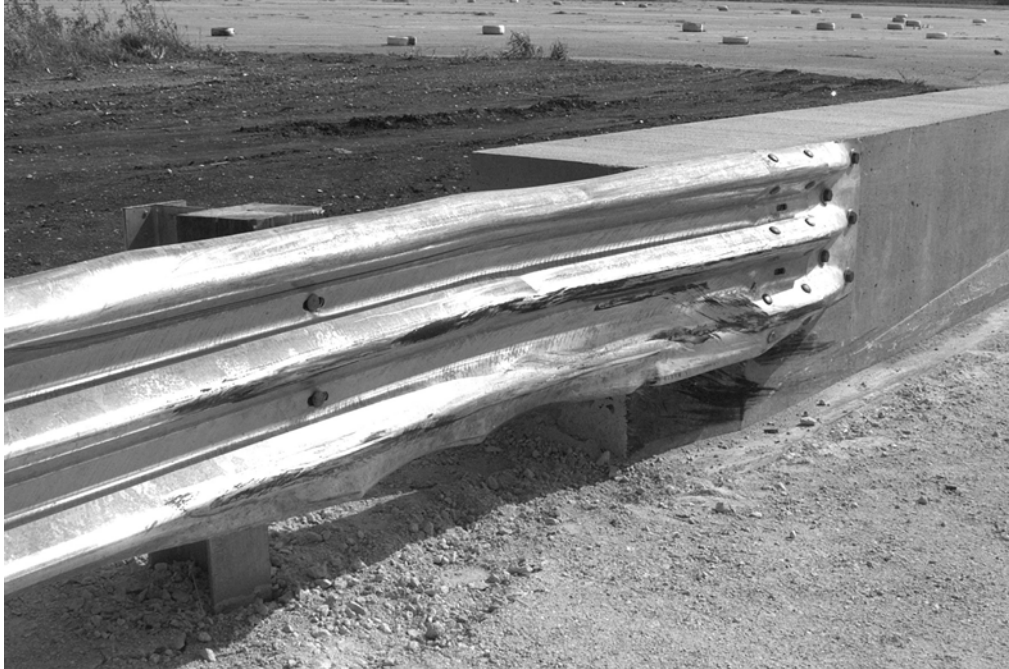
a) Damage at impact.
