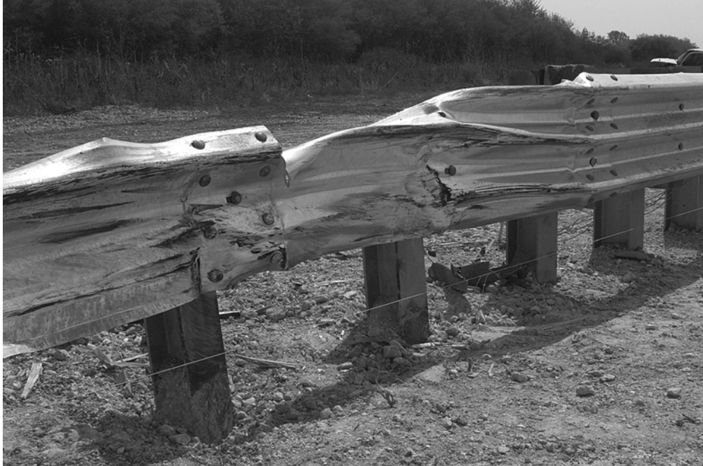
a) Damage at impact.
