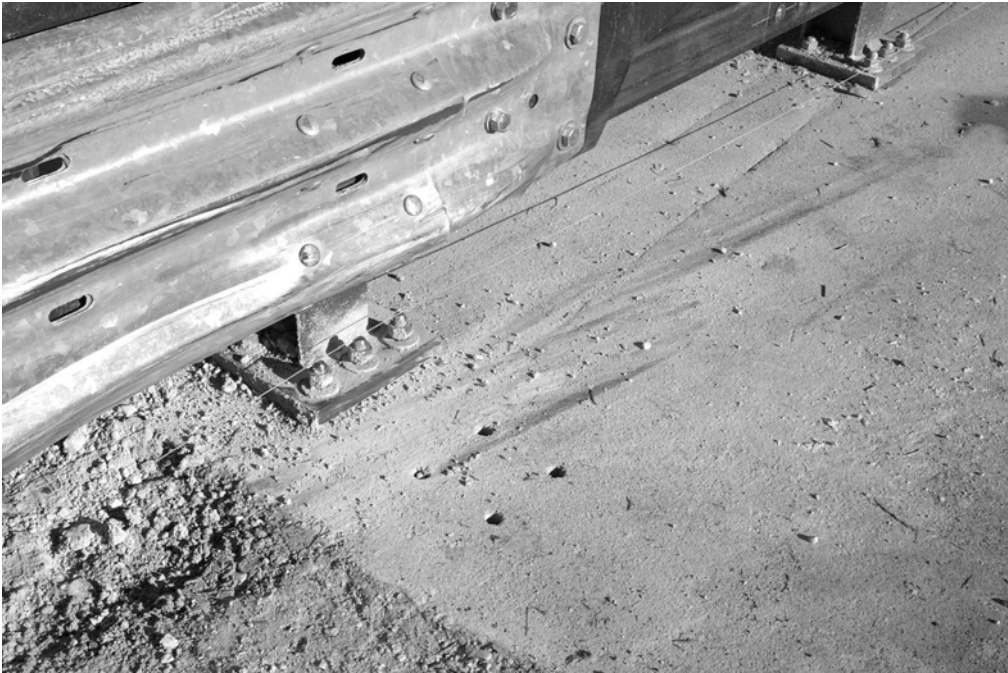
b) Damage at end post.
