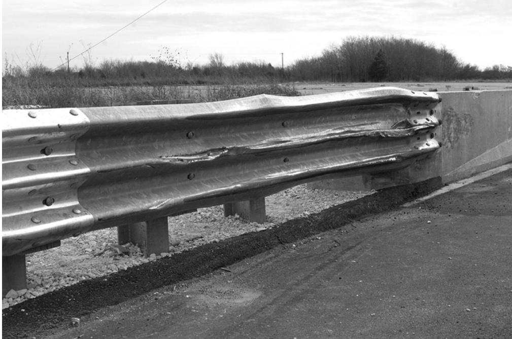
a) Overall view of damage.
