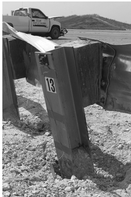
b) Damage at post 13.
