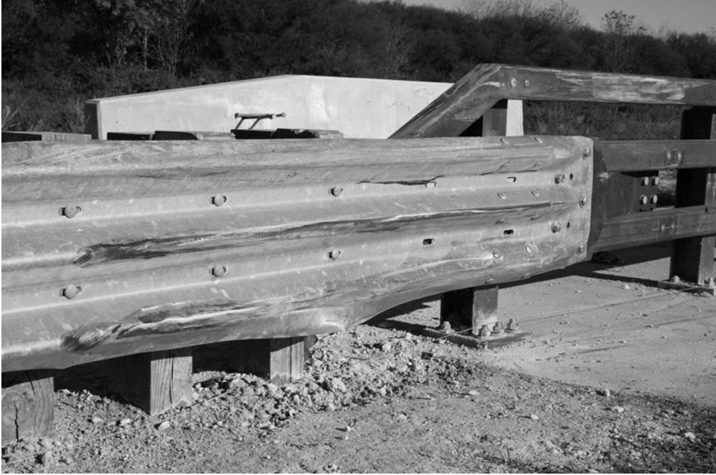
a) Damage at impact.
