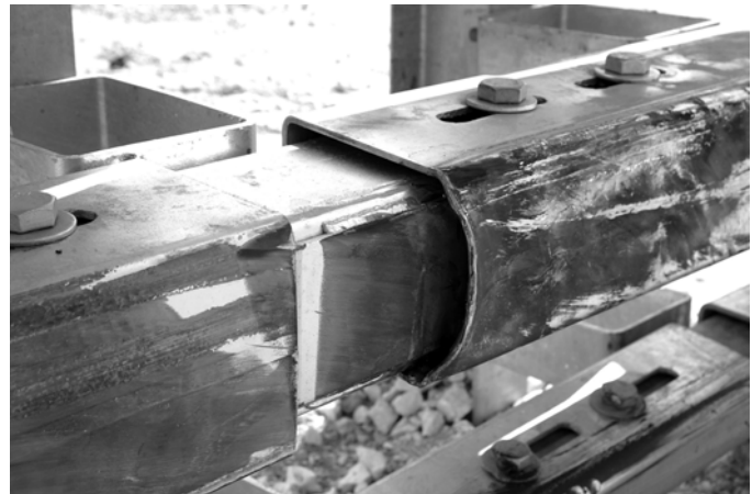
c) Damage at upper splice.
