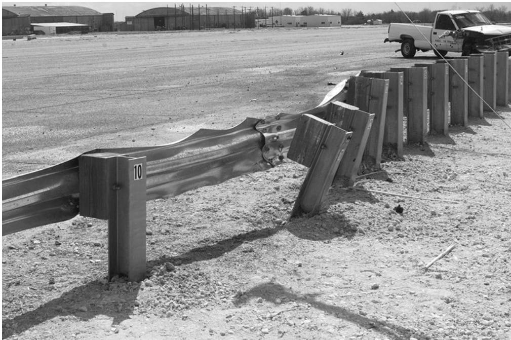
b) Damage from field side.
