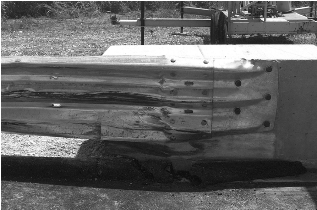
b) Damage at transition.
