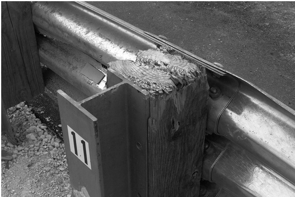
b) Damage at post 11.
