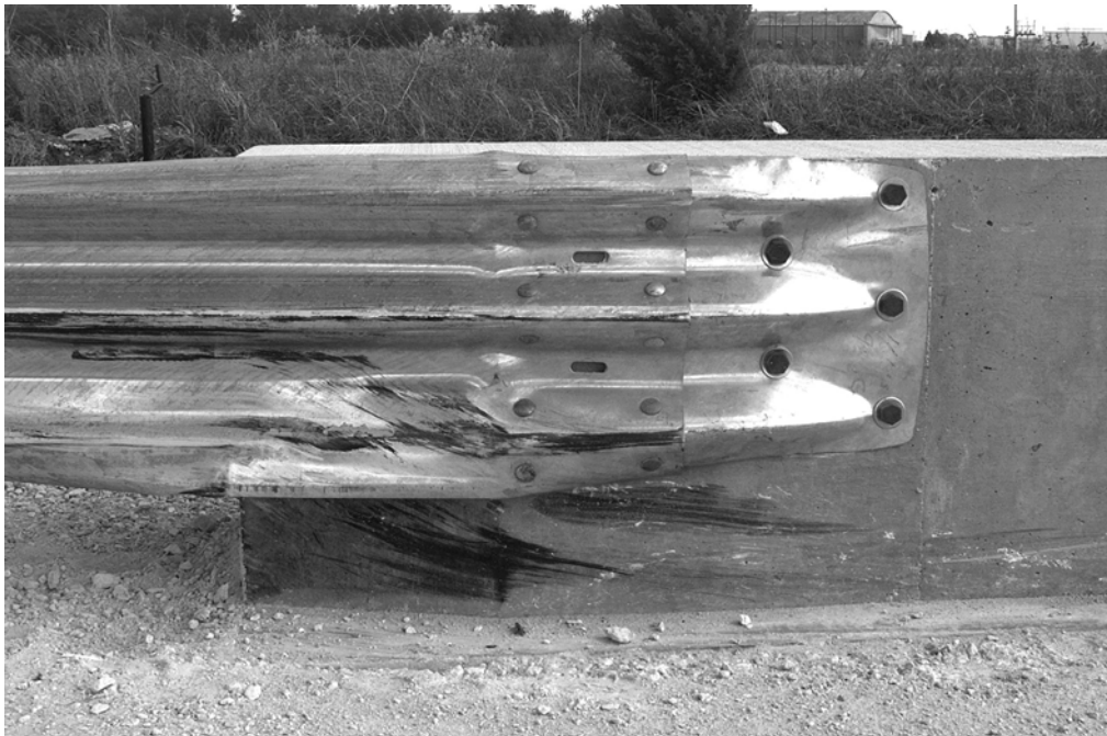
b) Damage to parapet.
