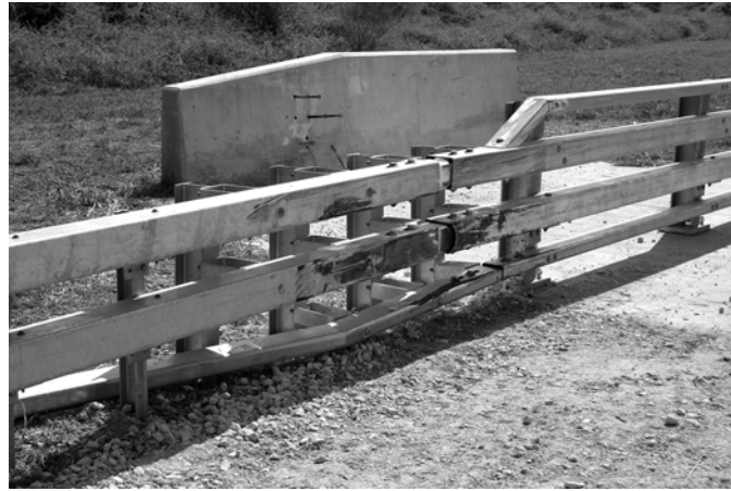
b) Overall view of damage.
