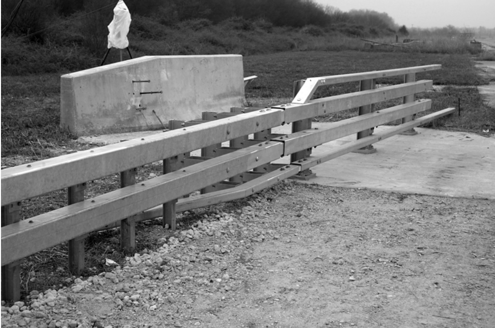
a) Traffic side of installation.
