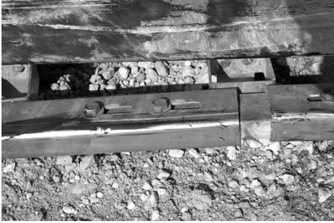
a) Damage at lower splice.
