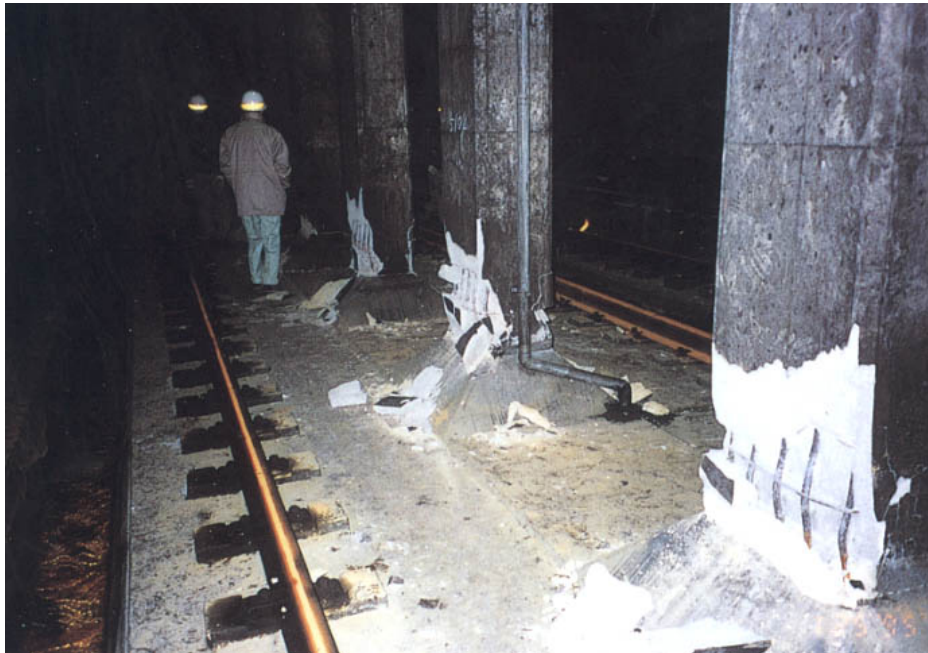
Figure 13-10 Fracture at Base of Columns of Cut-and-Cover Tunnel between Daikai and Nagata Stations - 1995 Kobe Earthquake, Japan
