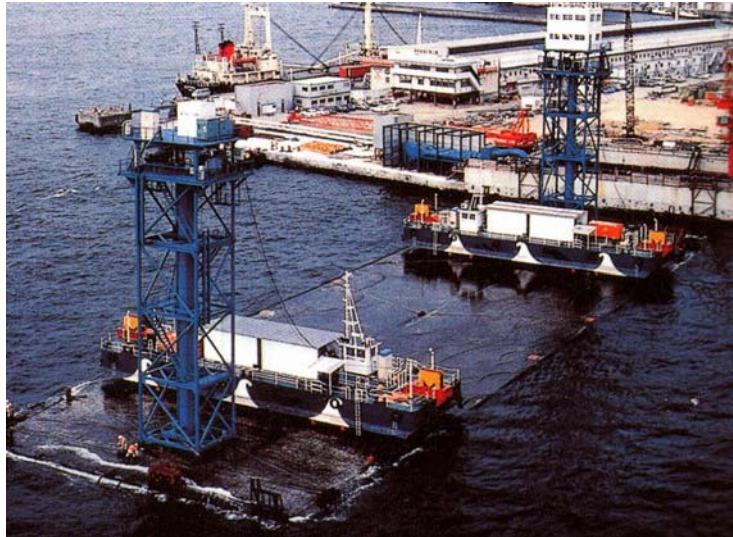
Figure 11-13 Osaka Port Sakishima Tunnel Element Transported to Site with Two Pontoon Lay Barges
