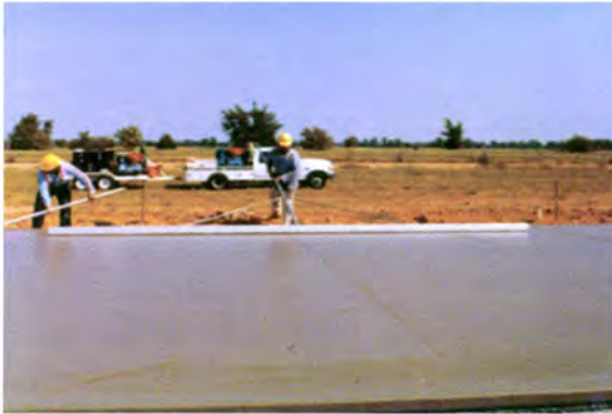
Figure 12. Using a 7.6 m (25 ft) straightedge to check the profile of a pavement.
