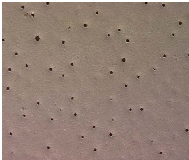
Figure 61. Photo. Surface condition of the three-coat system.
