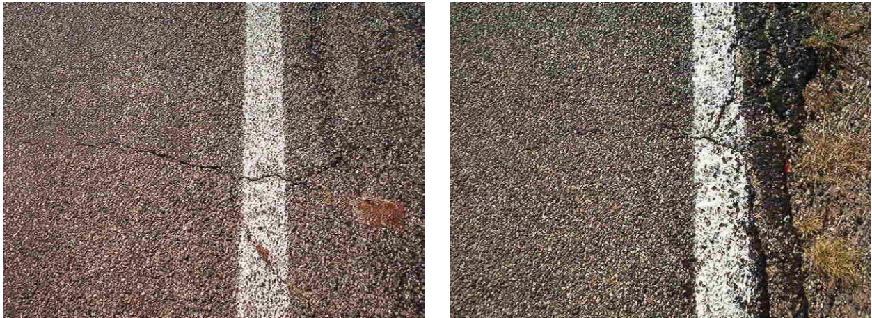
Figure 37. Photo. Examples of Cracks at Site 2.
