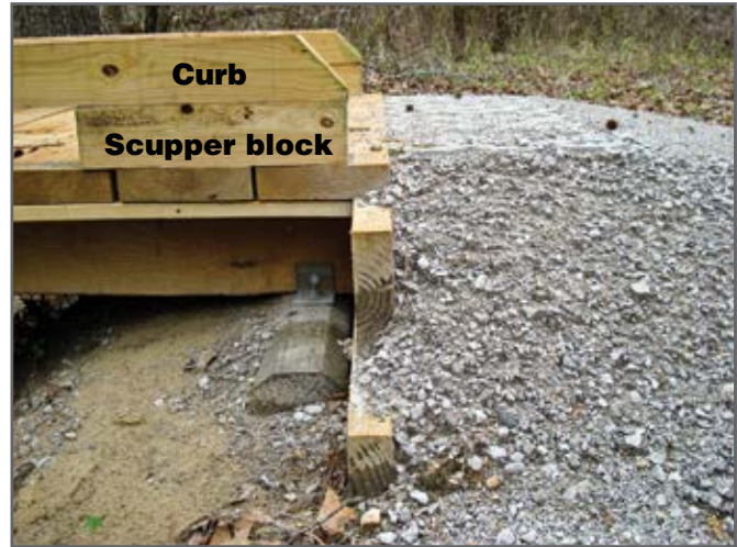
Figure 6—Place curbs on top of scupper blocks, which are held in place with carriage bolts placed through the curb, scupper block, decking, and curb retainer.
