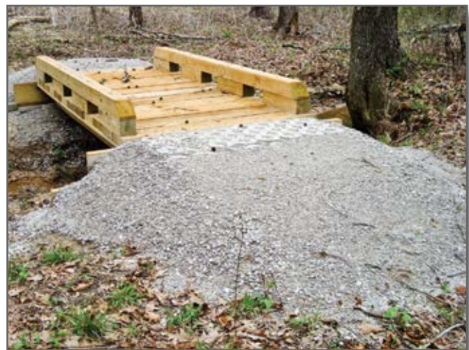
Figure 1—This bridge was constructed on an all-terrain vehicle trail at the Tombigbee National Forest, Mississippi.
