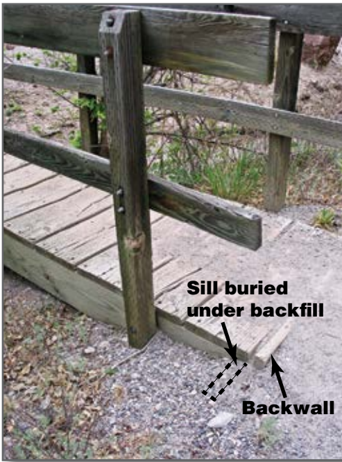
Figure 5—When backwalls are not extended beyond the sides of the stringers, backfill wraps around the backwall, which causes dirt to accumulate on the sills, causing the decay process to begin and allowing the bridge approaches to unravel.
