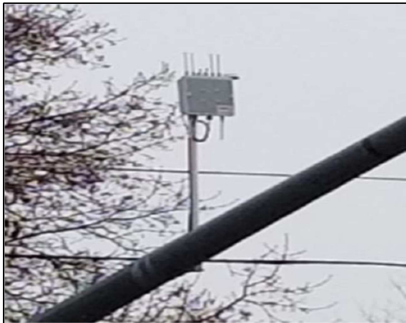
Figure 4-13 RSU Installed on Mast Arm (Leonard, 2002)
