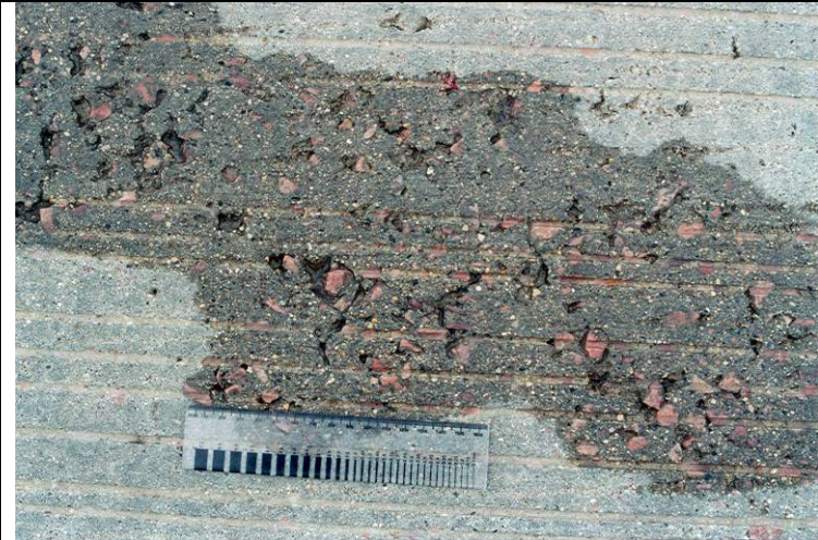
Photo 7: Honeycomb defects observed on Span 2 of Southbound Bridge.
