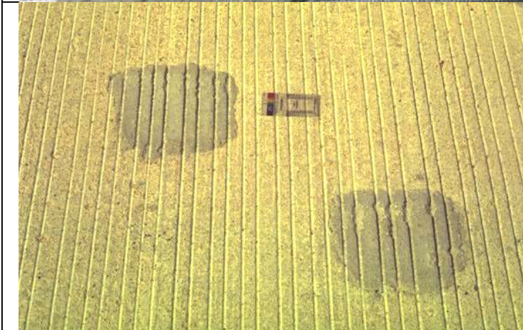
Photo 8: Typical patched area.
