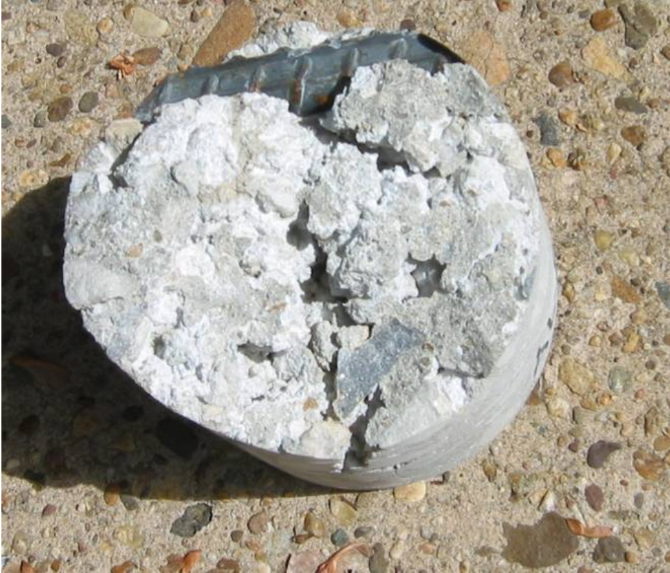
Figure A1-9: Honeycombing in core AL-5.
