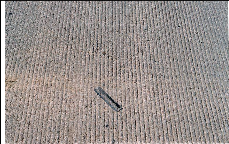
Photo 4: Close up view of typical diagonal crack.
