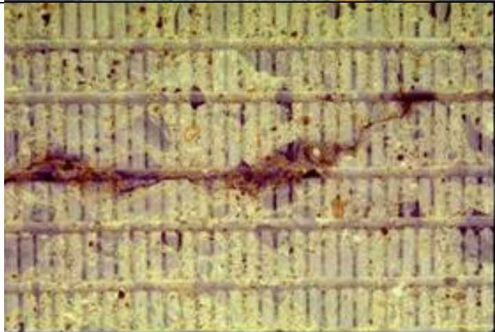
Photo 7. Typical Map Crack (Detail view 0.010 in).
