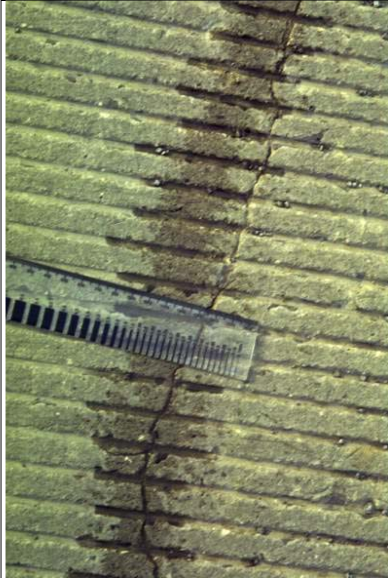
Photo 8: Close-up view of the longitudinal cracks. The width of the crack is 0.022 in.
