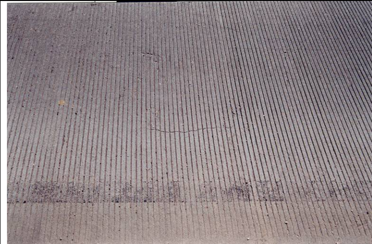
Photo 7: Close up view of longitudinal cracks on bridge deck.
