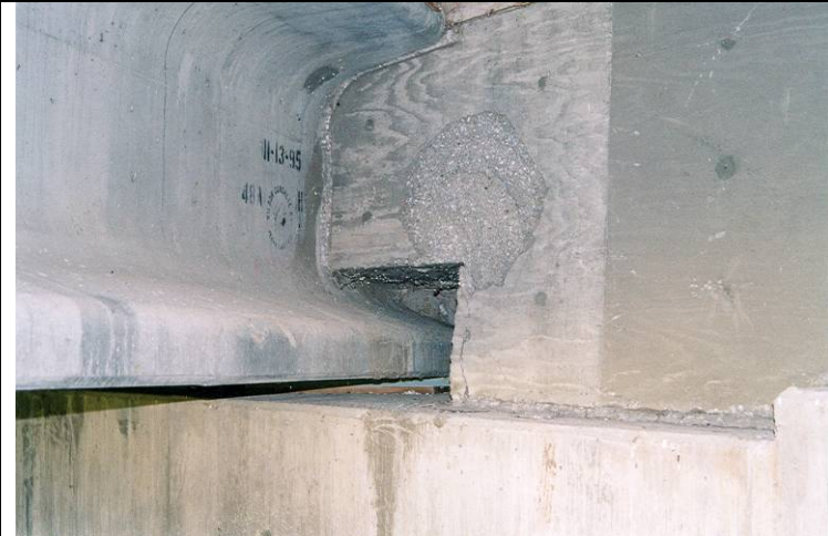
Photo 10: Spalling near the joints of second girder north side.
