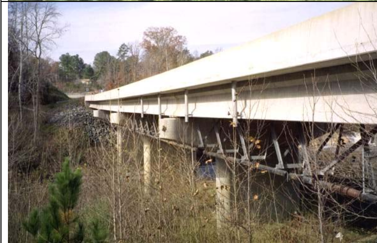
Photo 23: South elevation, exterior Girder E. Note 8-in. sewer pipe below Girders D & E.
