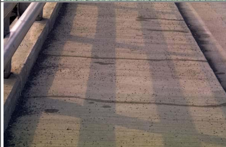
Photo 15: Cracks on the sidewalk.
