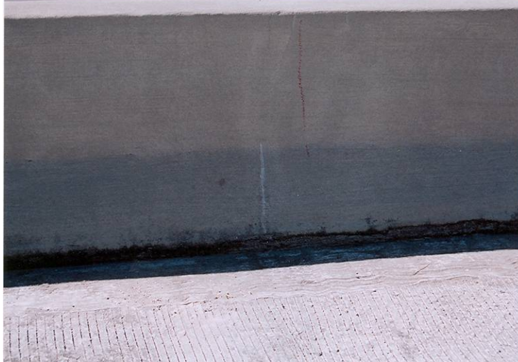
Photo 8: View of the concrete barrier at westbound bridge showing cracking and efflorescence.
