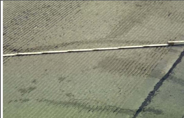
Photo 13: View of the diagonal crack. The width of the crack is 0.010 in.
