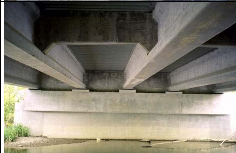
Photo 17: View of the girders A through E, Span A, Pier 1 (fascia girder A is on the left).
