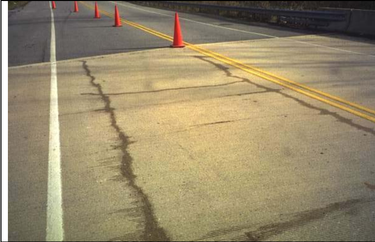
Photo 7: General view, longitudinal cracks, west bound
