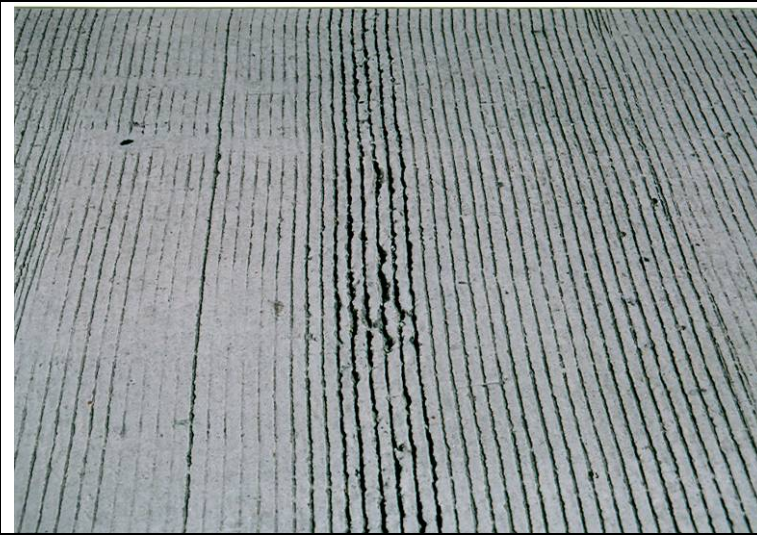
Photo 10: Broken tined edges at eastbound bridge Span 3.
