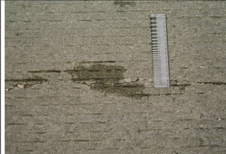
Photo 5: Closeup view of a transverse crack.
