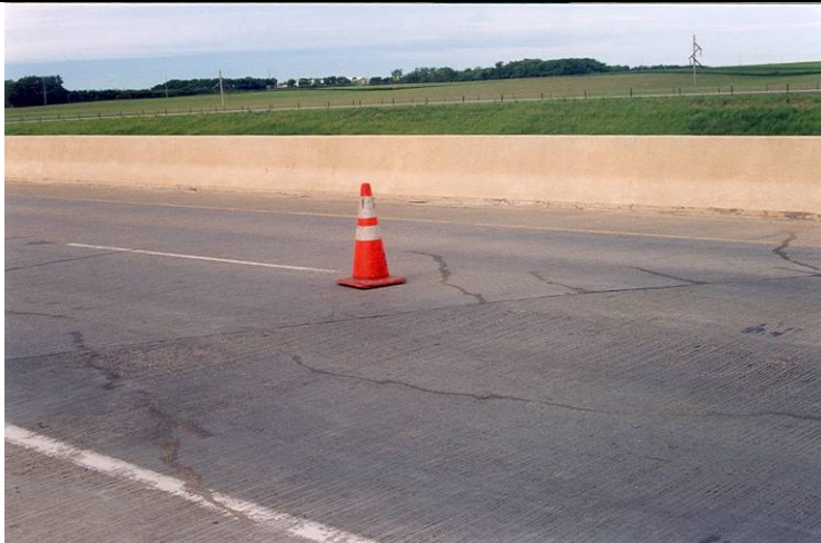
Photo 3: Cracks on the north side approach slab on the I-29 Northbound Bridge.
