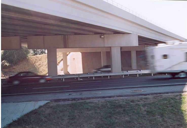
Photo 4: View of the underside of bridge, the pier in foreground supports Span 2.
