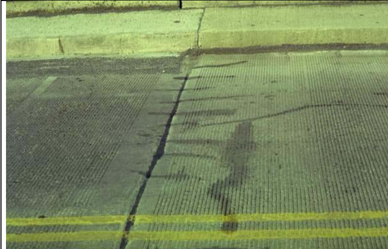
Photo 4: General view of the longitudinal cracks at the south end of the bridge.
