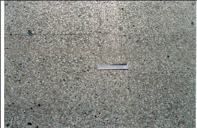
Photo 6: Close up view of typical longitudinal crack.
