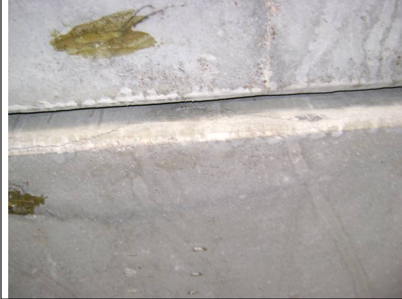
Photo 11: Close-up view showing of the impact crack in the 16 th girder.
