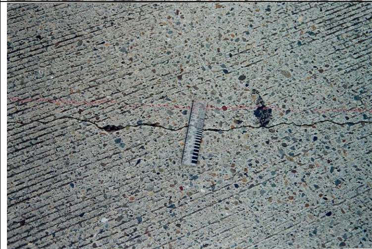
Photo 8: View of the typical diagonal cracks. Crack width is 1mm.
