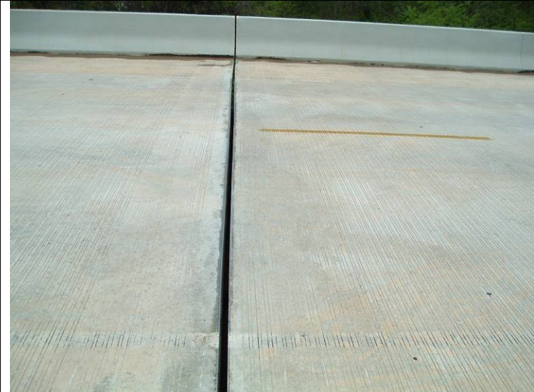
Photo 11: Unsealed gaps in between adjacent spans.
