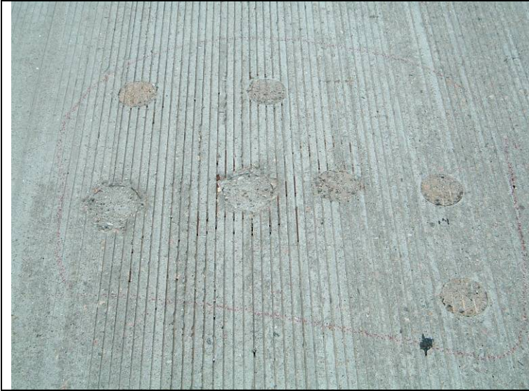
Photo 10: Failed patching work on bridge deck.
