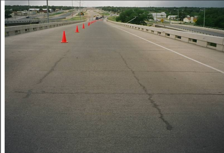
Photo 8: View of the westbound bridge, the western end of Span 4 showing the rectangular cracking pattern.
