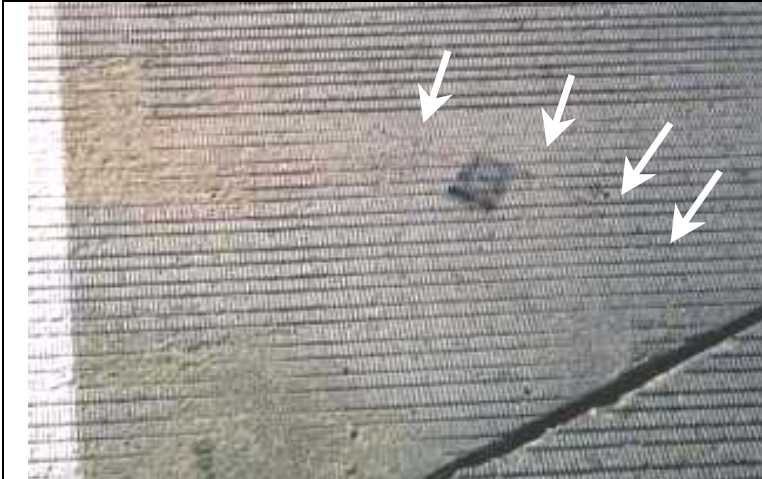
Photo 7: General view of the typical diagonal crack.
