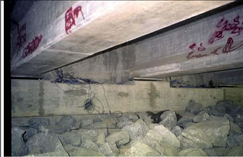
Photo 19: View of the girders B and C, abutment B (interior girder B on the left).
