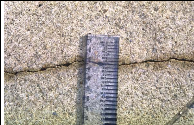
Photo 9: Typical diagonal crack, detail view, 0.018 in. width.
