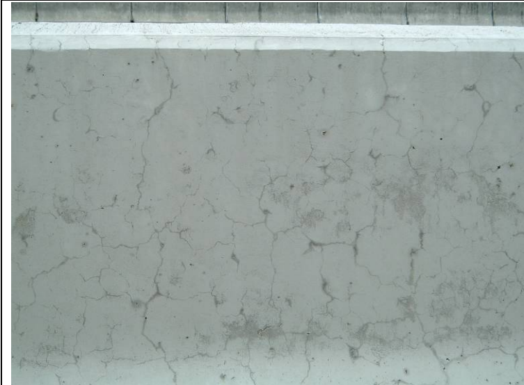
Photo 11: View of the map cracking on concrete barrier wall at eastbound bridge south facing side. Concrete barrier wall showing cracking and efflorescence.
