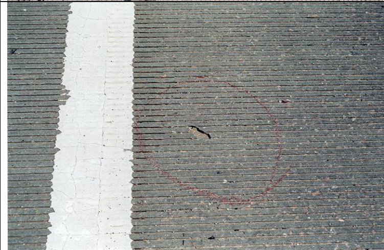
Photo 9: Close up view of typical pop out.
