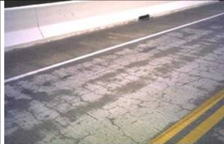
Photo 6. Typical Map Crack General view.
