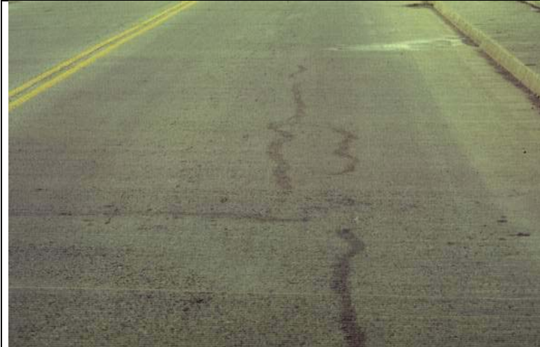
Photo 10: General view of the longitudinal cracks on the north bound.
