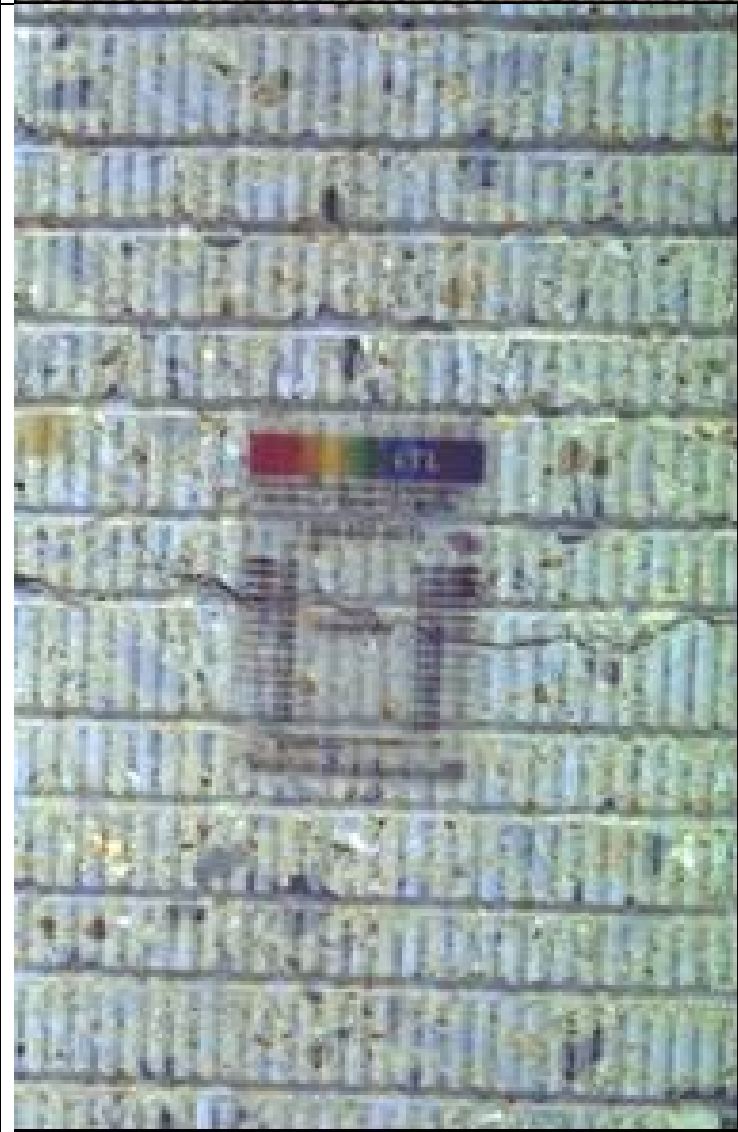
Photo 5. Typical Transverse Crack (0.016 in. width).
