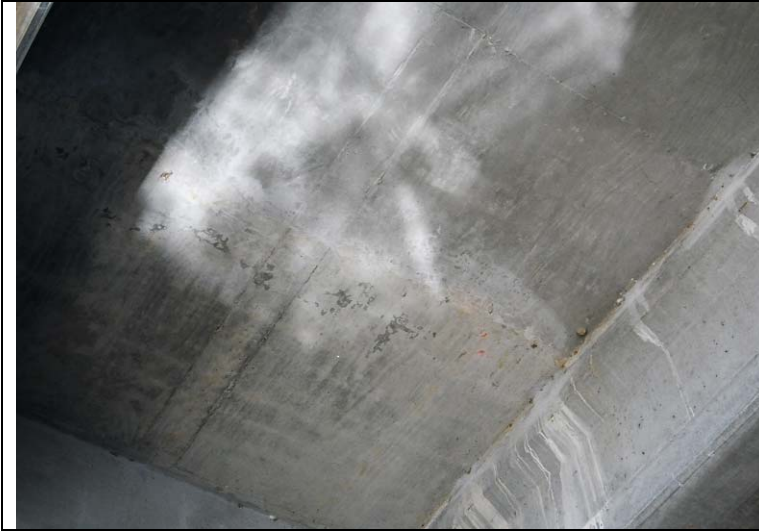
Photo 7: White precipitants along the overhang on the eastbound bridge.
