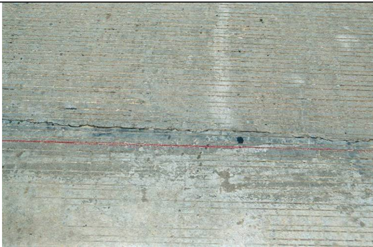
Photo 8: Close up view of typical transverse crack at deck joints.
