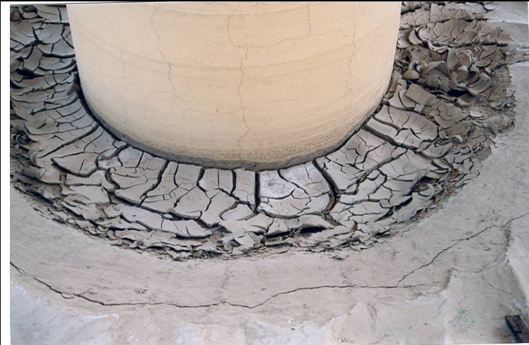
Photo 4: General condition of the piles at eastbound bridge. Cracks observed around the pile in the stucco.
