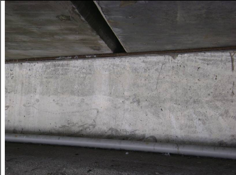
Photo 8: View showing cracks on the abutment at span ends.
