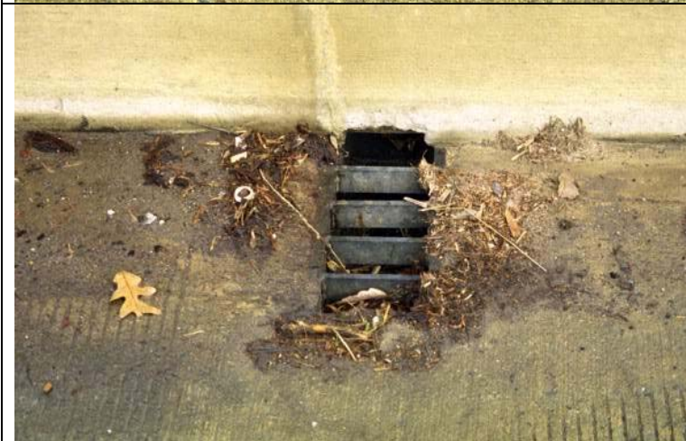
Photo 17: Typical deck drain with moderate debris.
