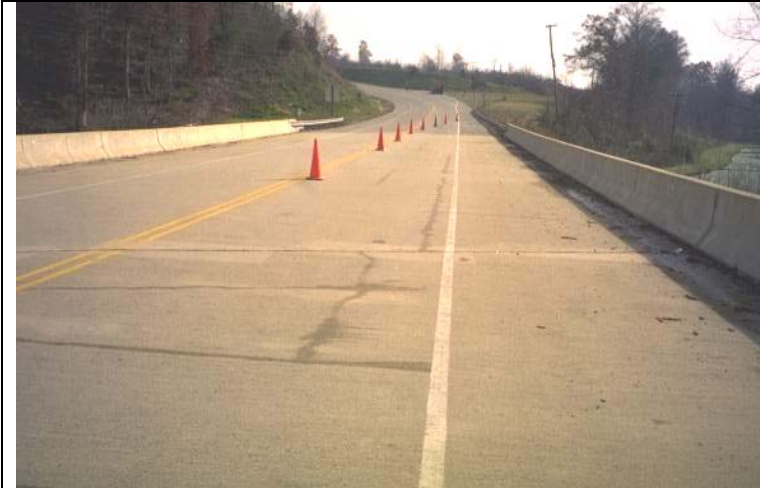
Photo 4: General view longitudinal cracks east bound.
