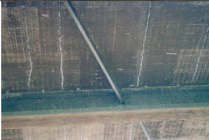
Photo 8: Close up view of underside of the bridge. Note the crack and efflorescence.
