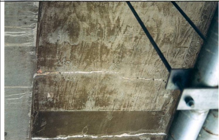
Photo 6: Close up view of the cracking at underside of bridge deck.
