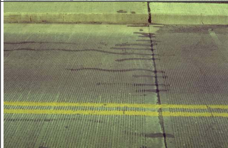
Photo 5: General view of the longitudinal cracks at the north end of the bridge.
