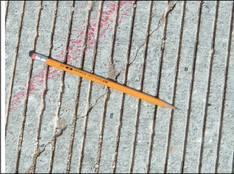
Photo 10: Close up view of the transverse crack at eastbound bridge Span 1.
