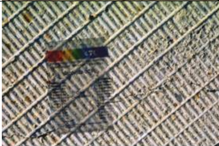
Photo 8. Typical Diagonal Crack (Detail view 0.010 in).
