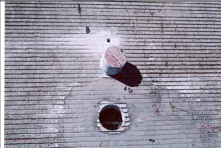
Photo 9: Broken tined edges core #6 at the shoulder of eastbound bridge Span 2.
