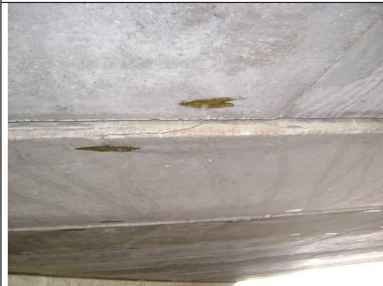
Photo 10: View showing the impact crack in the 16 th girder.
