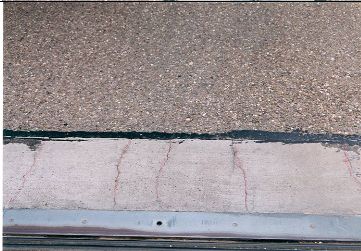
Photo 6: Close up view of the cracks at the joints.
