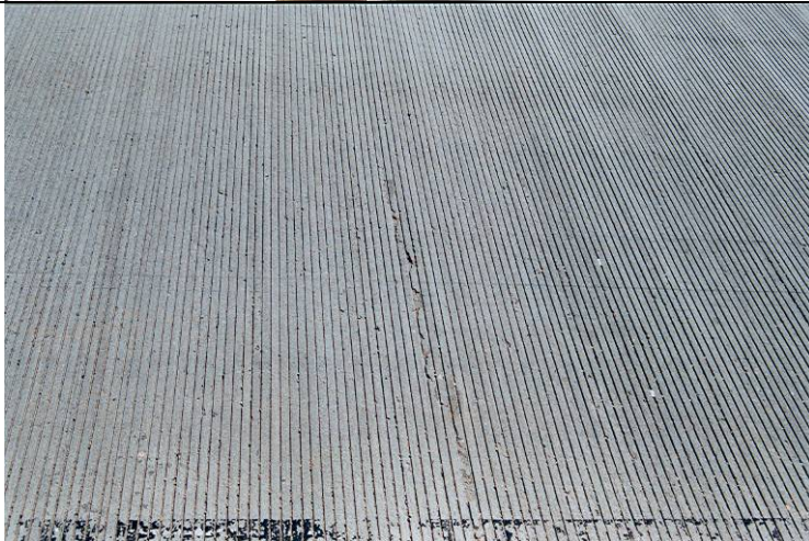
Photo 5: View of the transverse cracks on bridge deck.
