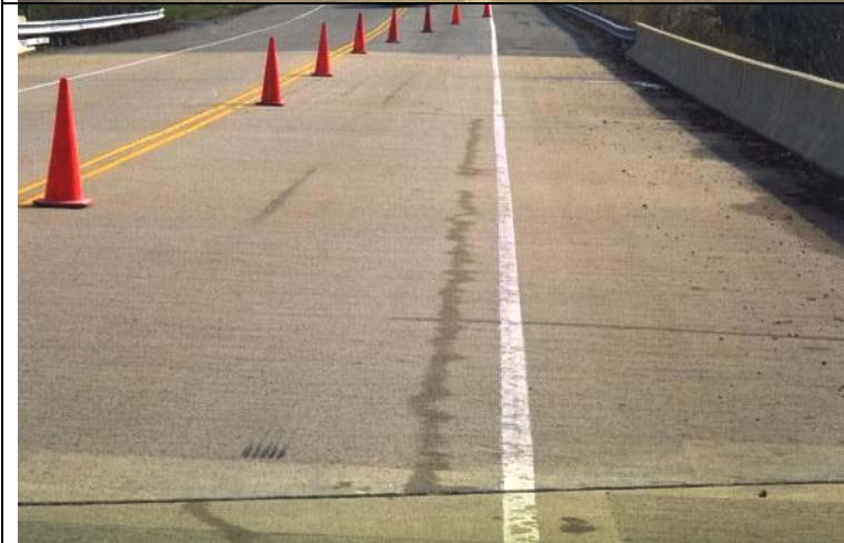
Photo 5: General view, longitudinal cracks, east bound.
