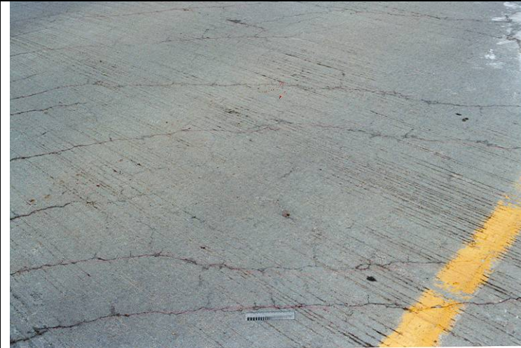
Photo 3: Crack patterns on the Southbound Bridge.
