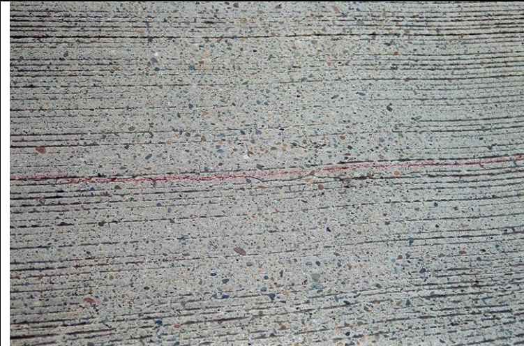
Photo 7: View of the typical transverse cracks.
