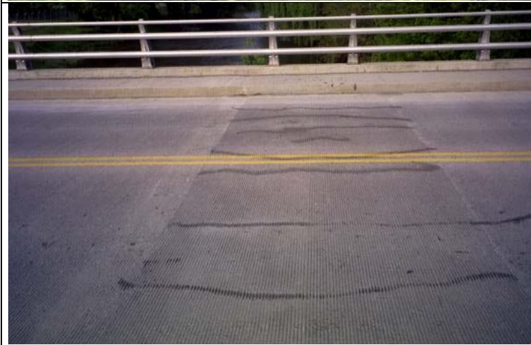
Photo 9: General view of the longitudinal cracks over the pier.
