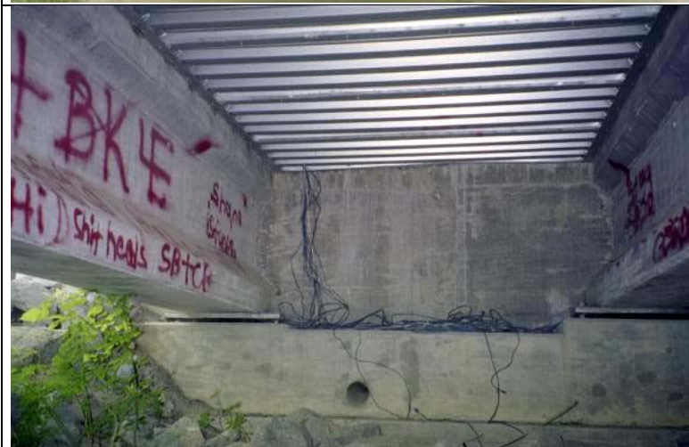
Photo 18: View of the girders A and B, Span B, abutment B (Fascia girder A is on the left).
