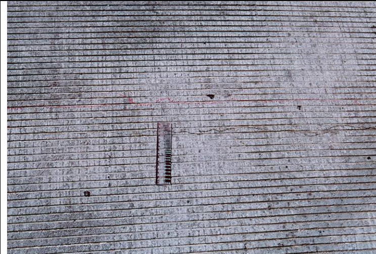
Photo 7: Close up view of transverse crack at Span 2. Crack width is 0.35 mm.
