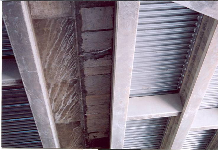
Photo 5: General condition of the girders at Span 2 facing west (southside). Cracks observed near efflorescence.
