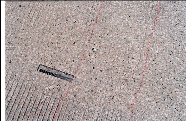
Photo 5: Close up view of typical transverse crack.
