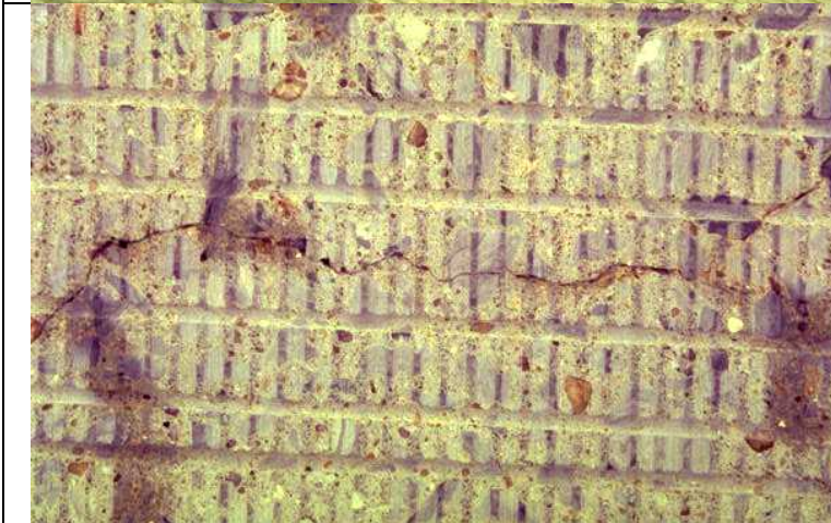
Photo 6: Close-up view of the typical map cracking. Crack width 0.010 in.
