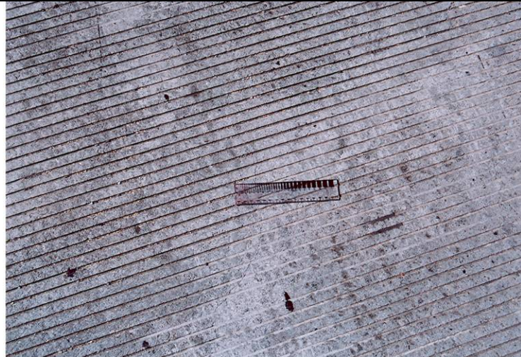
Photo 6: Close up view of diagonal crack at Span 1.
