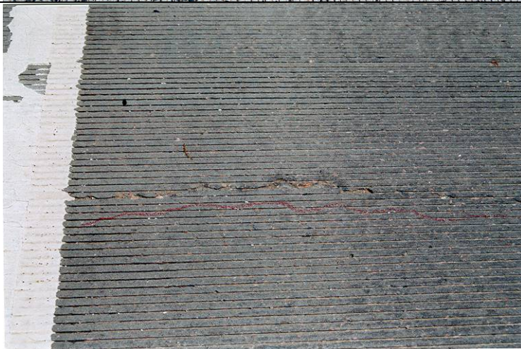
Photo 6: Close view of broken tinned edges along the transverse crack.
