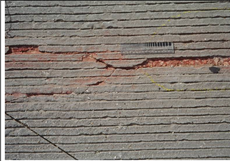
Photo 8: View showing spalling associated with cracks in the deck at span ends.
