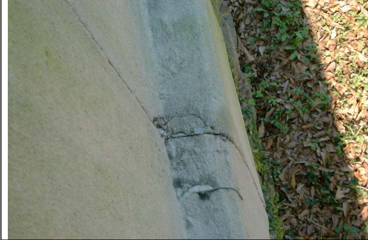
Photo 13: Close up view of the settlement related cracking at the eastern end of bridge Span 5.
