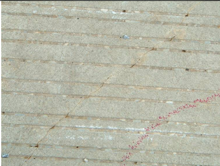
Photo 9: Close up view of typical longitudinal crack.
