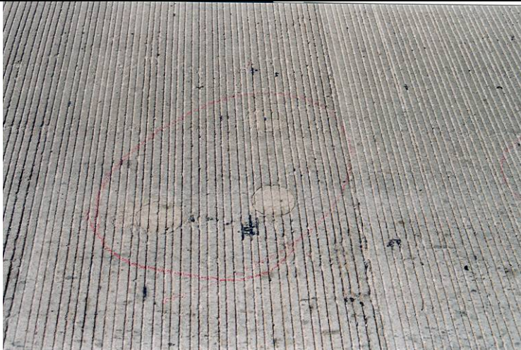
Photo 9: Cores taken by others and sign of broken tinned edges.
