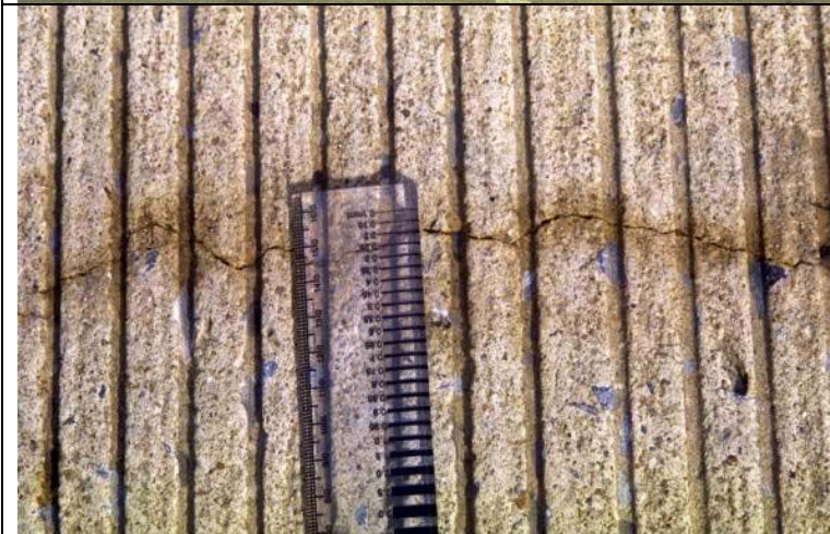
Photo 6: Detail view, longitudinal cracks, 0.008 in. width.
