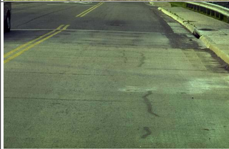
Photo 7: View of the longitudinal cracks on the south bound.
