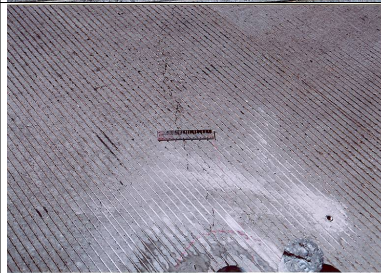
Photo 8: View of the diagonal crack extended through the core location.
