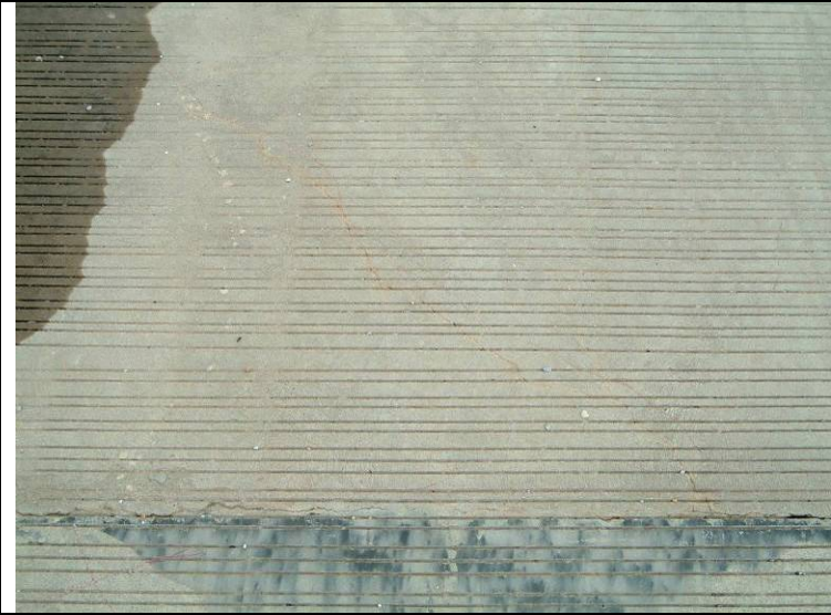
Photo 10: Close up view of typical diagonal crack.
