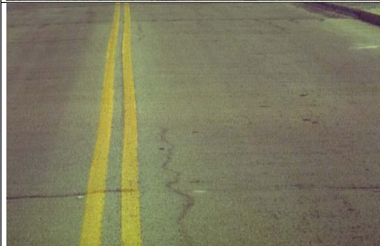
Photo 11: View of transverse cracks.
