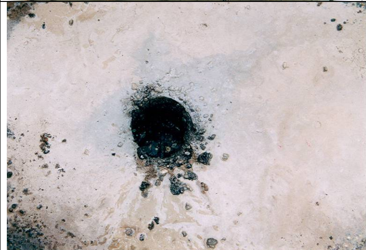
Photo 9: Close up view of coring process through asphalt concrete pavement to the top of girder flange.
