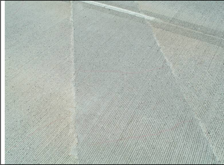
Photo 10: Patch in between the adjacent spans on the eastbound bridge.
