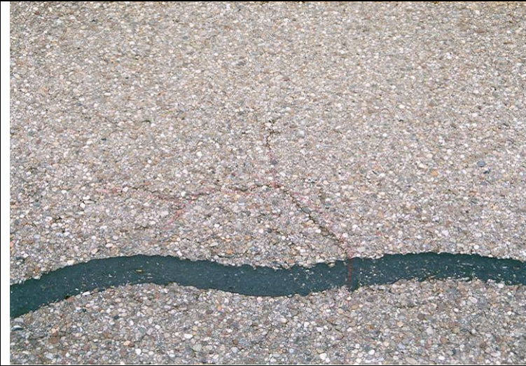
Photo 7: Sealed longitudinal cracks on asphalt overlay.
