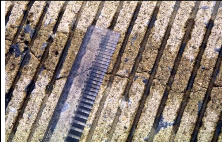
Photo 10: Typical diagonal crack, detail view, 0.025 in. width.
