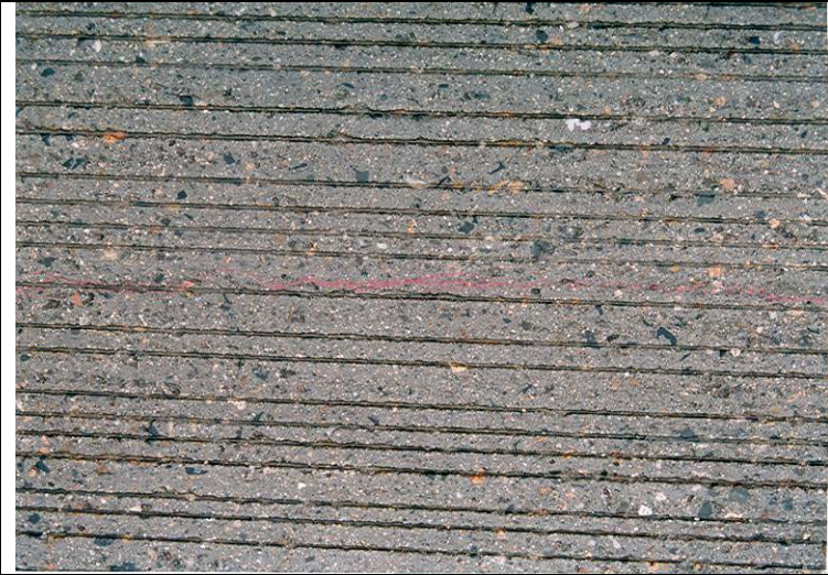
Photo 4: Close up view of transverse crack.
