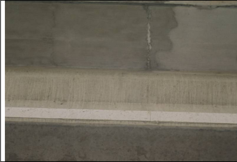
Photo 10: Cracks with efflorescence along the overhang on the westbound bridge.
