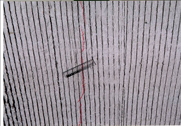
Photo 11: Close up view of the transverse crack at eastbound bridge Span 1.
