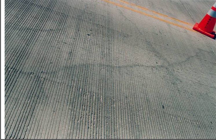
Photo 10: Close up view of the cracks at deck joints.
