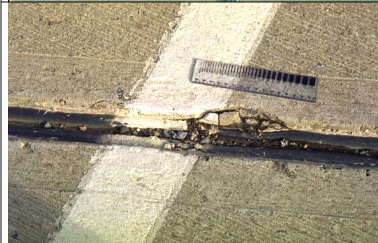
Photo 12: Typical D-Spall, detail view.
