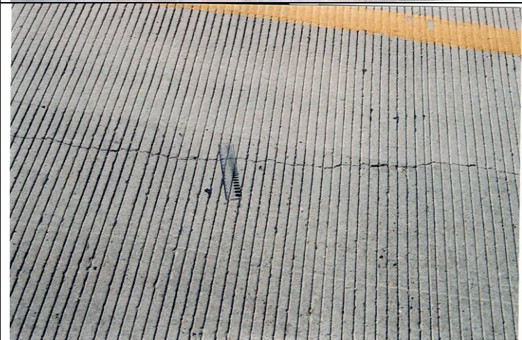
Photo 5: Close up view of longitudinal crack in the traffic lane.
