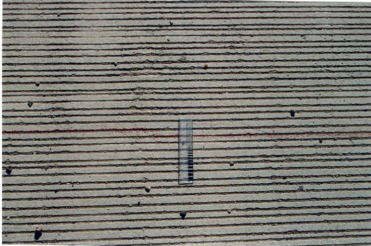
Photo 7: Close up view of typical transverse crack.
