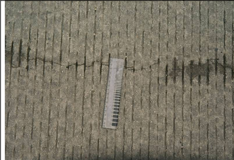
Photo 6: Closeup view of a longitudinal crack.
