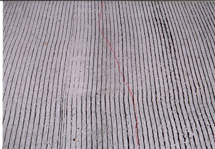
Photo 9: View of the transverse cracks at eastbound bridge Span 1 showing the transverse cracking pattern.
