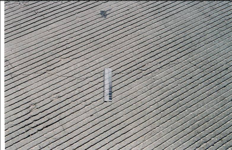
Photo 6: Close up view of typical diagonal cracks at bridge deck.
