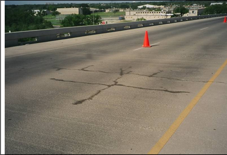
Photo 7: View of the eastbound bridge, the western end of Span 5, showing cracking pattern at the edge of span.
