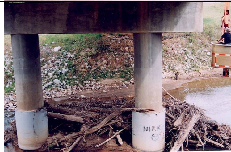
Photo 6: General condition of the piles at Span 2 east facing bridge. Accumulation of debris observed near the pile.
