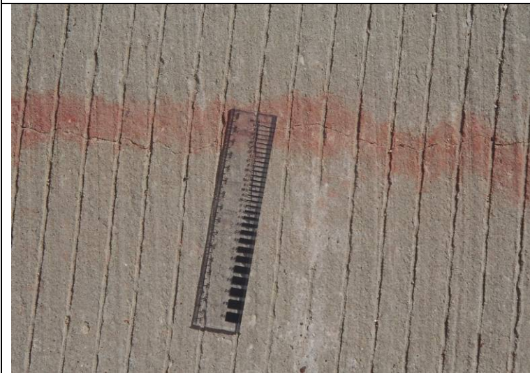
Photo 7: View showing typical crack in the bridge deck. Crack width is less than 1/32 in. and is categorized as hairline.
