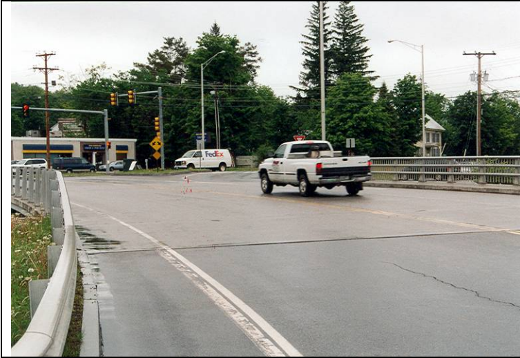
Photo 4: General view of longitudinal crack on bridge deck.
