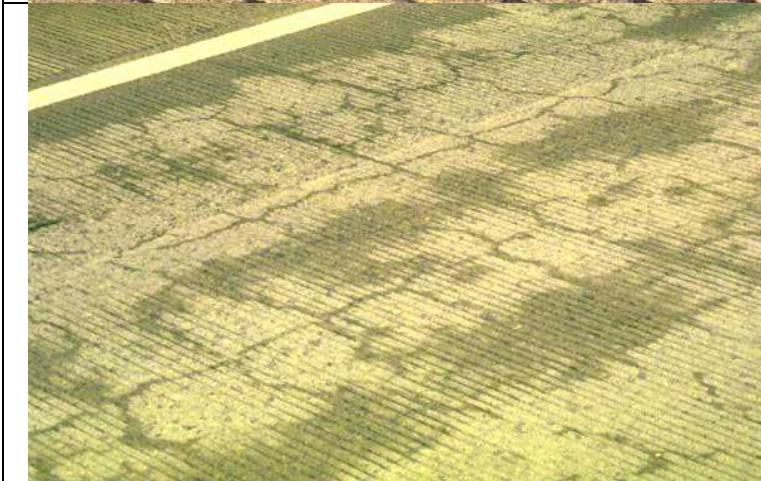
Photo 5: General view of the typical map cracking.
