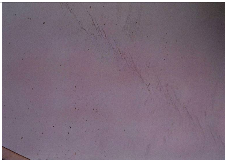
Photo 10: View showing close-up of fine cracks in the northeastern most girder of the northbound bridge.
