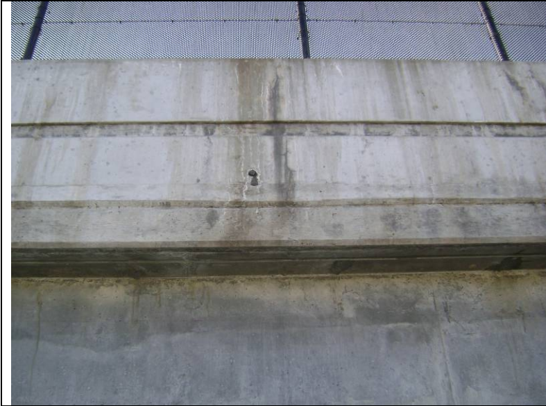
Photo 7: View showing typical cracks on the bridge parapet. Crack width is less than 1/32 in. and is categorized as hairline.
