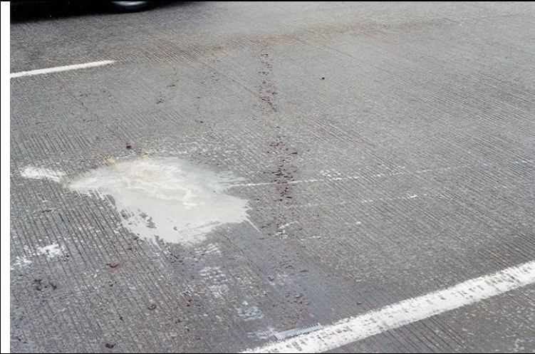
Photo 9: Close up view of patched core location on Southbound Bridge. Note the crack over the core.
