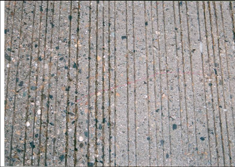
Photo 5: Close up view of longitudinal crack.
