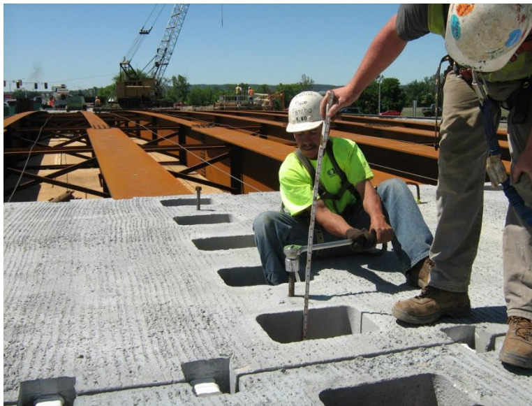
Figure 2 Construction workers adjusting the elevation of the full depth precast concrete deck panels by adjusting leveling bolts (courtesy Iowa DOT).
