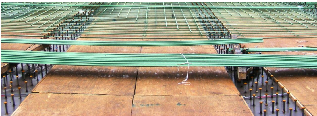
Figure 6 Photo showing temporary wood formwork installed on a steel plate I-girder bridge
