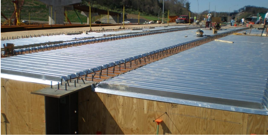
Figure 5 Photo showing permanent steel stay-in-place deck formwork installed on a steel plate I-girder bridge
