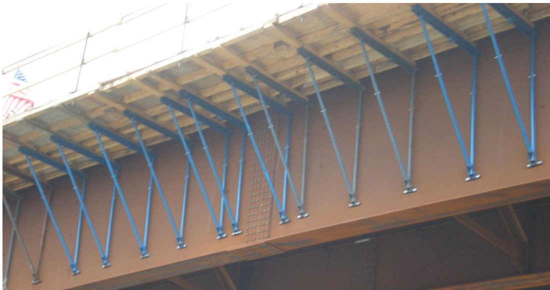
Figure 7 Photo showing deck overhang brackets supporting cantilever slab construction on a steel plate I-girder bridge
