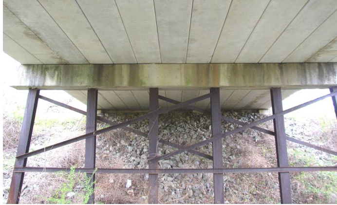
Figure 23 Pile bent with braced steel H-piles serving as both columns and foundations for the pier.
