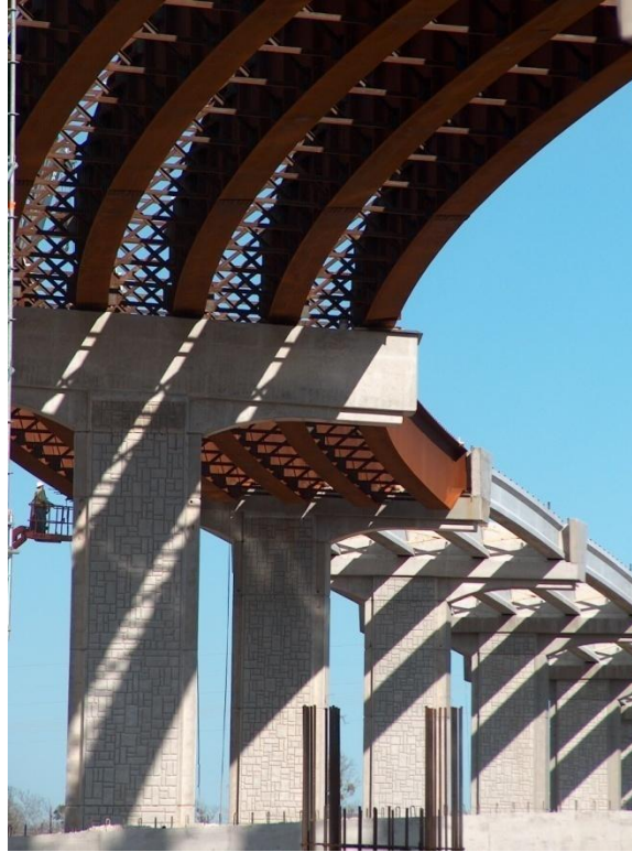
Figure 30 Dapped girder ends rest on an inverted T pier cap in a single column pier.
