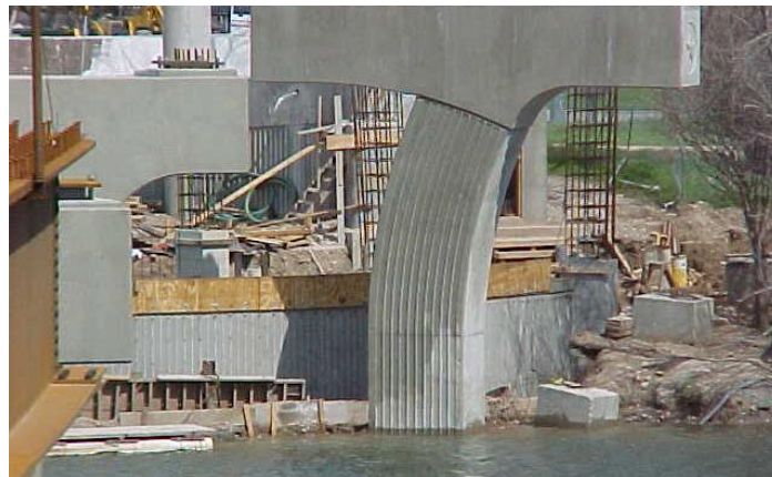
Figure 22 There can be a wide range of variations on the basic single column pier configuration, such as this pier with a haunched pier cap and single, unsymmetrical curved column featuring form liner treatments for a pedestrian bridge.
