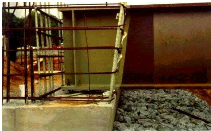
Figure 13 Example of integral abutment details, prior to casting the closure pour. Note the reinforcing running through the girder web and the anchor bolts used as girder supports.
