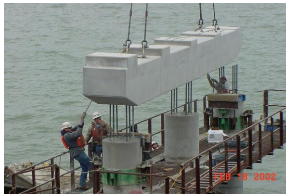
Figure 32 Example of a precast pier cap being used on a long viaduct bridge. The columns were cast-in-place with dowels projecting from the top of the columns. The dowels fit into pockets in the precast pier cap. The pier cap initially rested on collars around the tops of the columns. The collars were adjustable to facilitate leveling of the pier cap. Once the pier cap was set, grout was injected into the dowel pockets and the gap between the columns and the pier cap.
