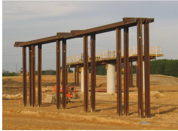
Figure 3 Driven steel H-piles arranged as the foundation for a conventional abutment. Later, MSE retaining walls will be built in front of these piles, and after that the abutment cap and backwall will be cast.
