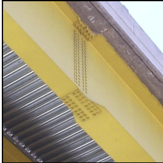
Figure 2 Photograph of a Steel Plate I-Girder Field Splice at a Flange Width Transition
