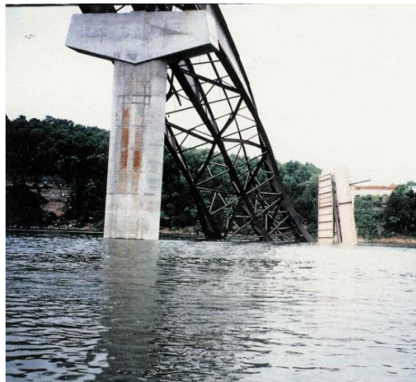
Figure 4 Collapse of a Bridge over the Tennessee River due to Insufficient Bracing
